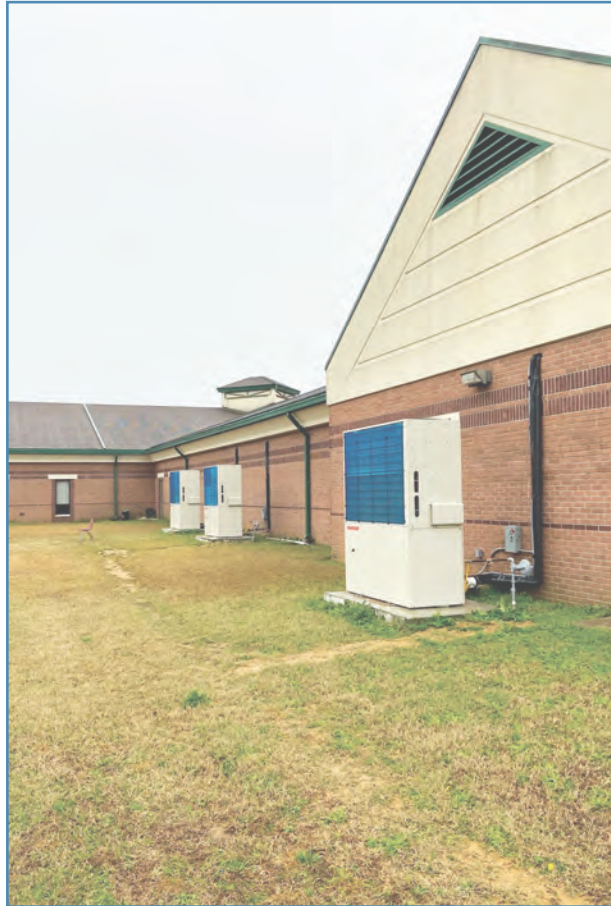
FIGURE 2: Dublin City Schools is in the process of installing 266 tons of VRF GHP systems at the Middle School Campus. The success of the first project in 2019 was a determining factor in this decision. Courtesy: Dublin City Schools and Clay Consulting
