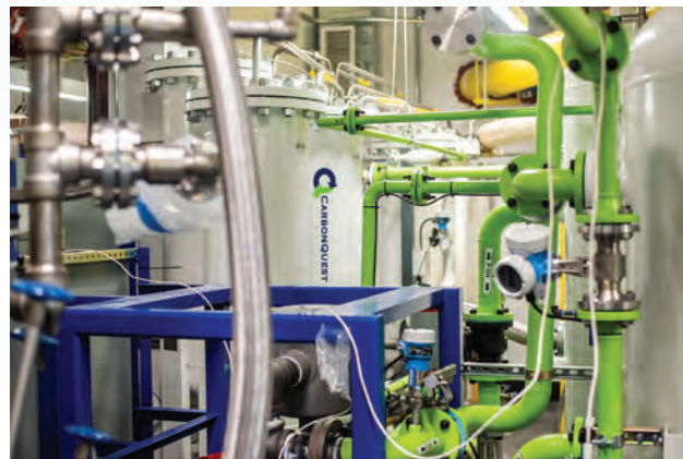
FIGURE 1: CarbonQuest has developed a distributed on-site CCUS they call Building Carbon Capture and Storage™ (BCCSTM) to capture carbon dioxide (CO 2 ) emissions. Courtesy: CarbonQuest
