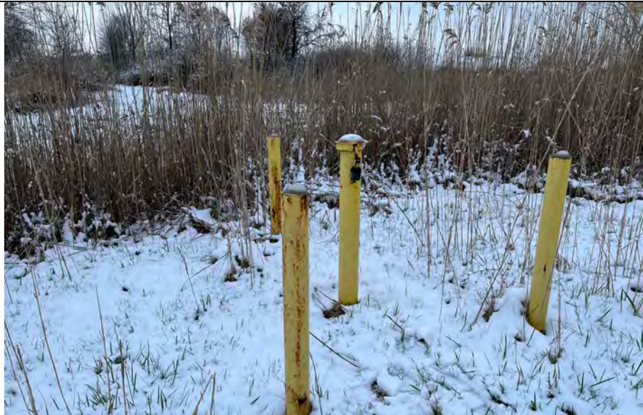
7. Monitoring Well 16-05. Well Protected and Cap Locked. Well Protection and Capping Typical of Inspected Above Ground Monitoring Wells.
