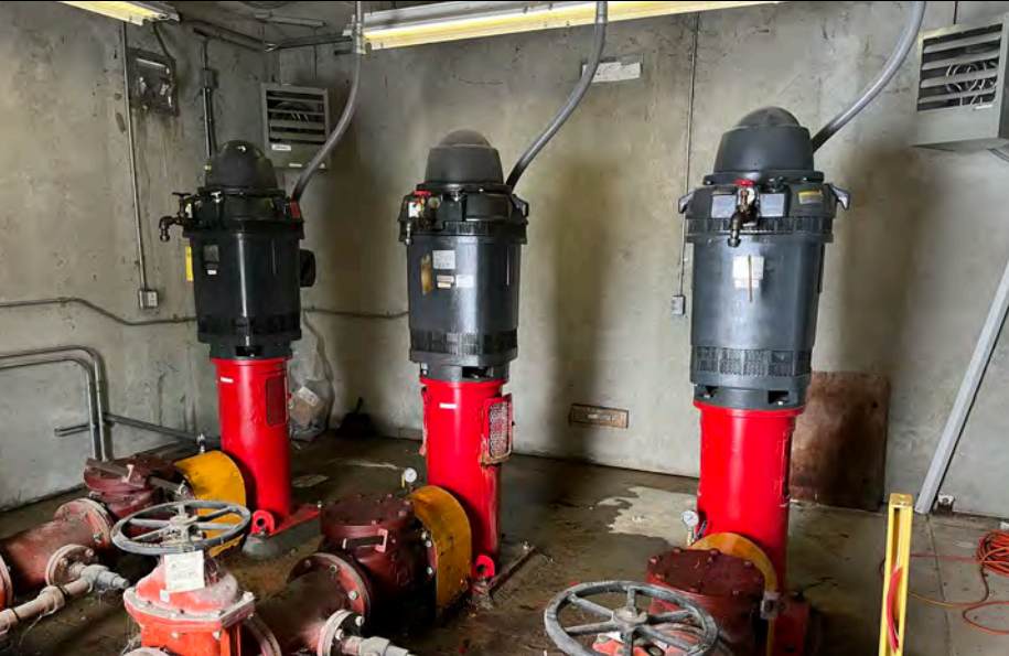
3. Pump Control Panel. All 3 Pumps were Available for Use. Wall Flow Meter (Not Shown) appeared OK. Pumps were Observed but not Pumping at the Time.
