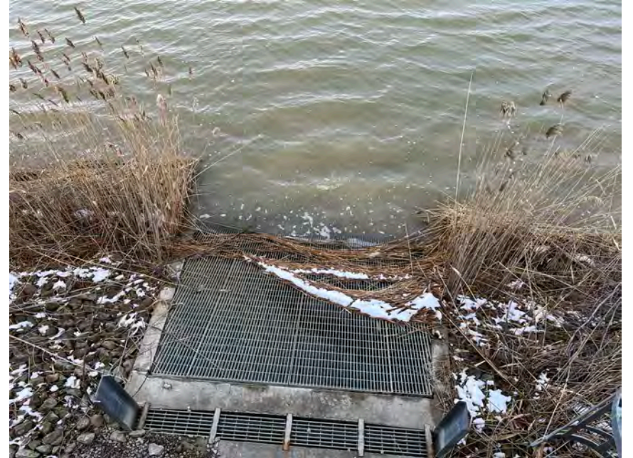
2. Intake Screens at SWDB with Some Minor Vegetation at Bottom. Water from Basin is Pumped Back to Power Plant Using One or More of 3 Pump3.
