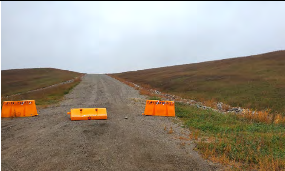
53. DTE Photo of Haul Road to Top of Final Cover with Runoff Collection Ditches Either Side of Road. Previous Re-Occurring Slope Erosion Right Side.
