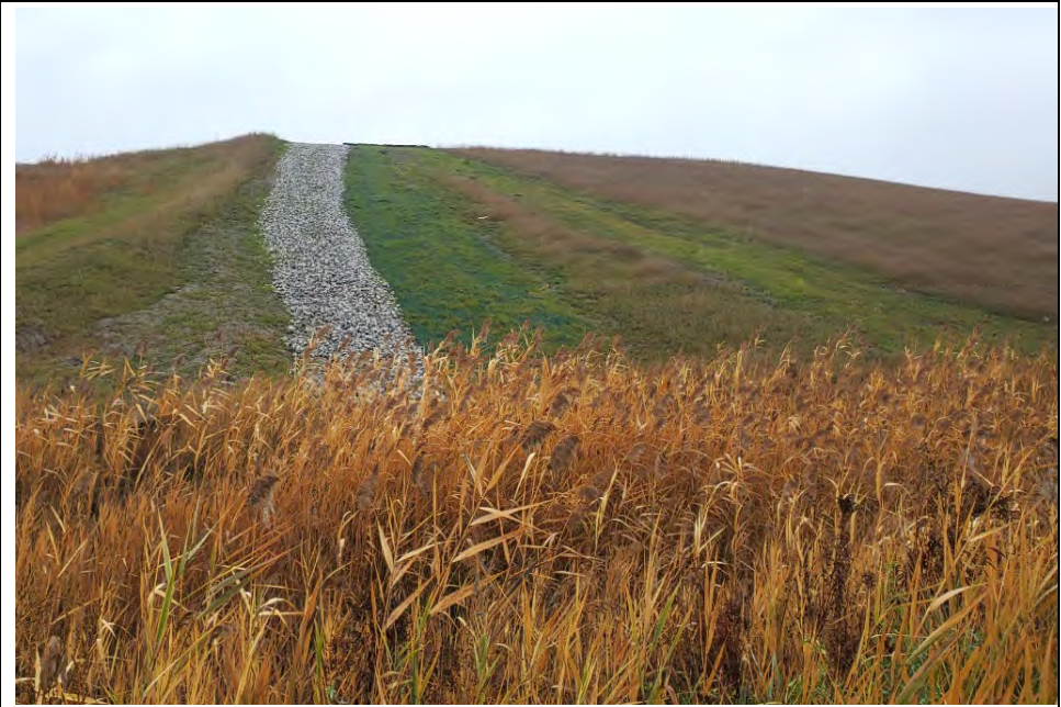
42. DTE Photo of Area G2 Phase 1 Downslope Drain from Cover Swale on Top of Cover.
