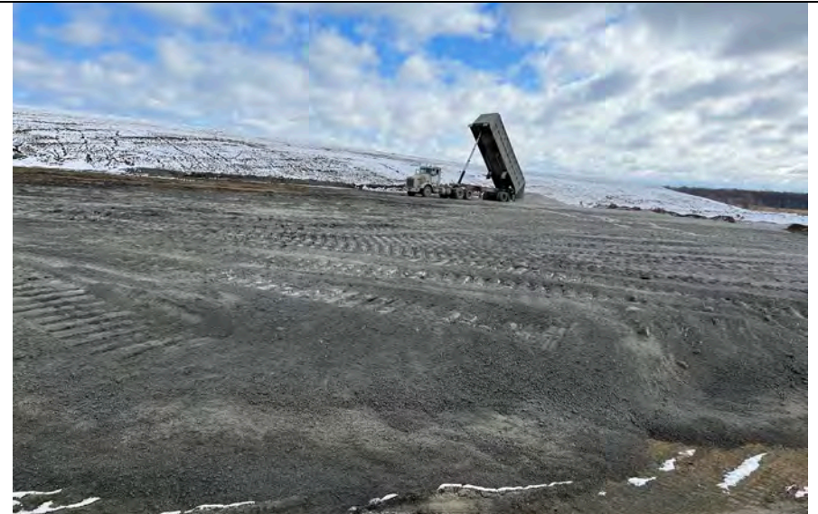
44. CCR Haul Trucks Safely Unloading What from a Distance Appears to be Bottom Ash and/or Fly Ash. Active Area G2 Phase 2 Shown.
