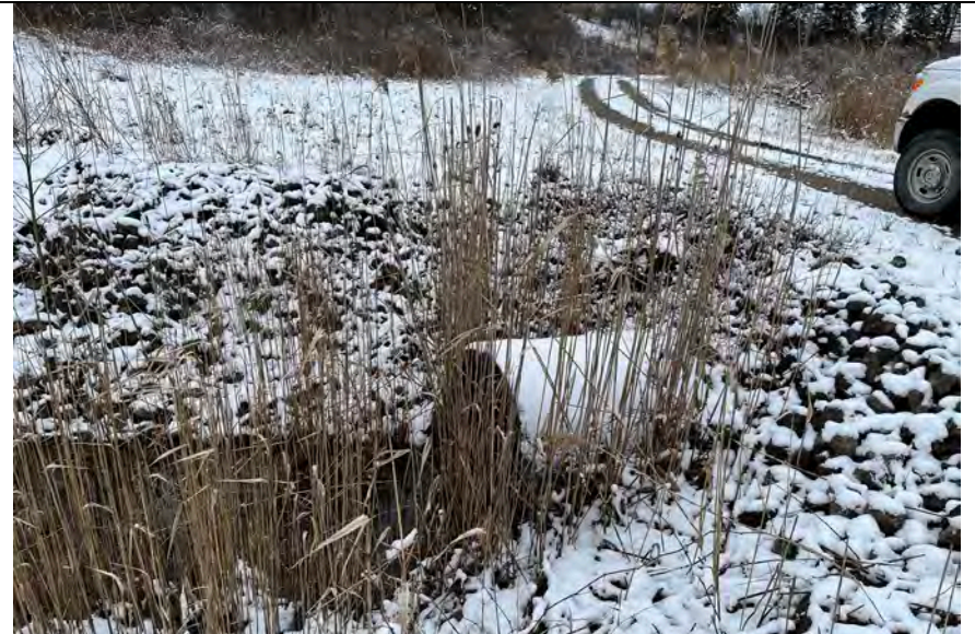
20. Culvert and Riprap Downslope Where Ditch Clearing of Vegetation Had Been Performed in 2021. Flow did not Appear to be Blocked.
