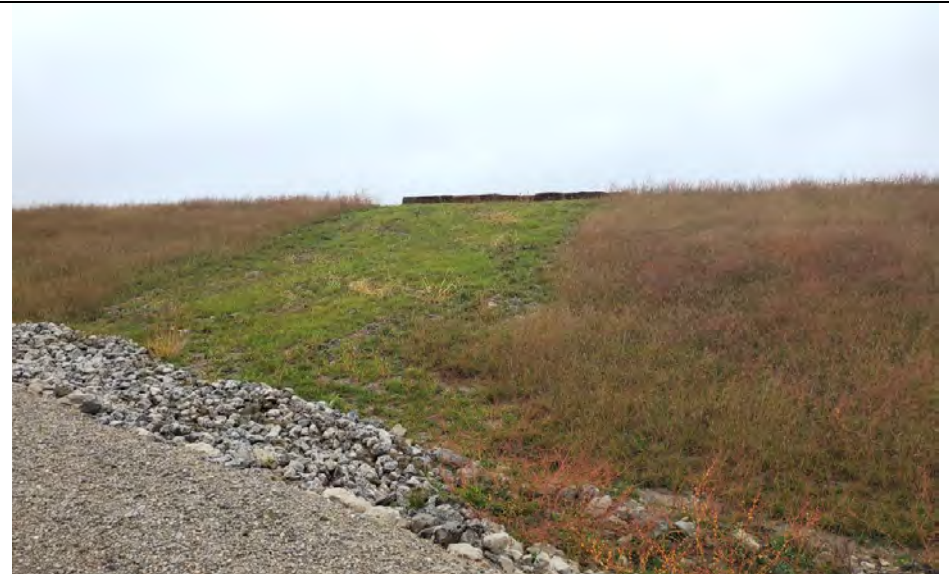
54. DTE Photo of Repair with Added Riprap and Slope Erosion Repair/Re-Seeding. Note Silt Fence at Top where Surface Runoff Meets Slope.
