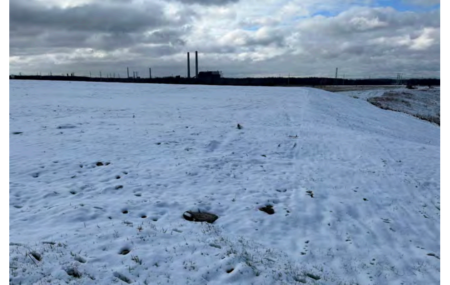
32. Top of Landfill Area G2 Phase 1 Along West Side Slope where Grading and Initial Seeding had Taken Place in Fall of 2021.
