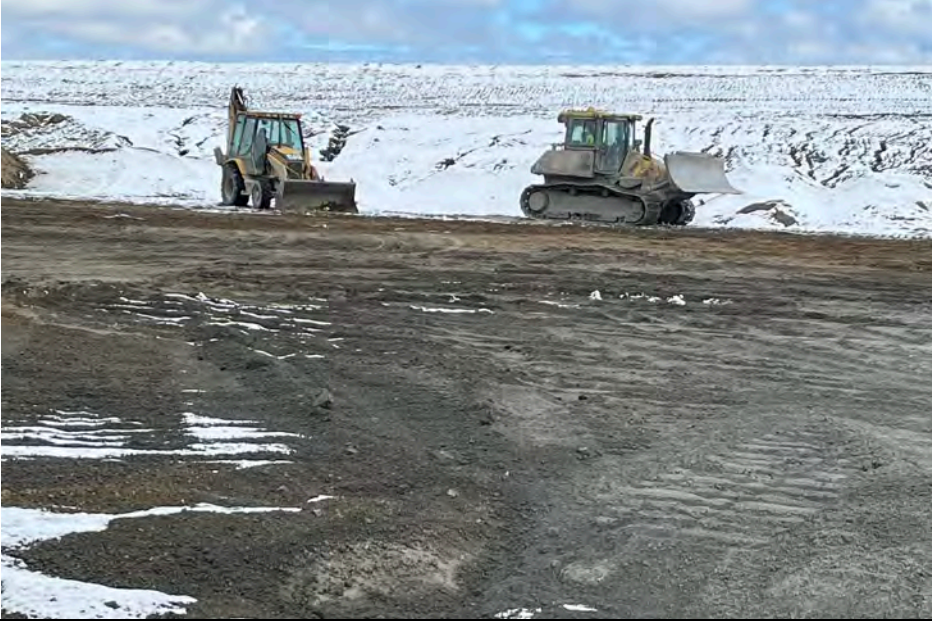
5. Active Area G2 Phase 2 Construction Equipment Working. The Light Snow Cover Occurred the Day/Evening Before.
