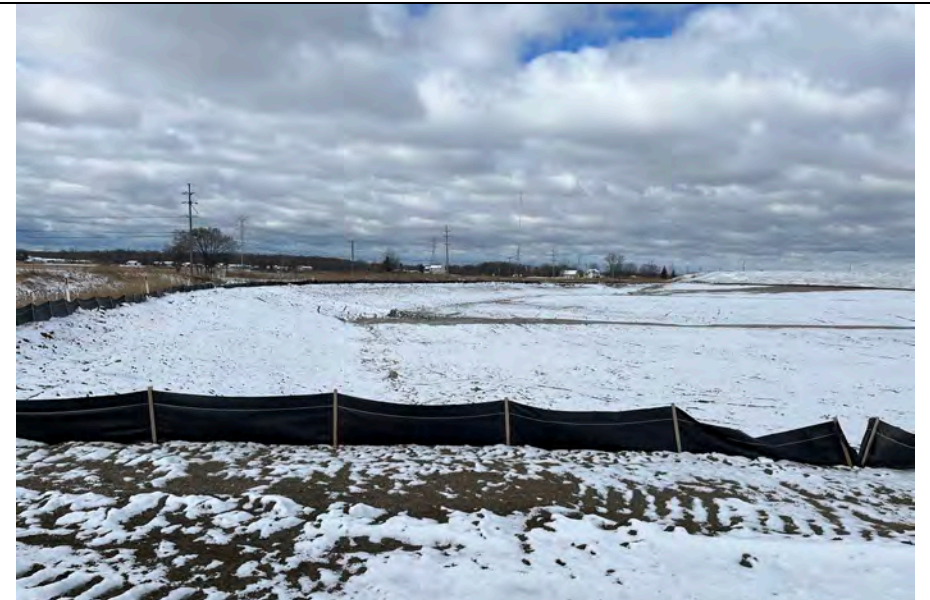
48. Construction Fencing Around Landfill G2 Areas. Internal Drainage Ditch Located Forefront of Photo (Same Ditch as in Photo 47).
