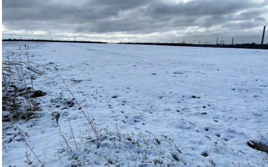
31. View of Top of Landfill Area G2 Phase 1 that has been Graded and Capped in Accordance with Landfill Cover Design. Initial Seeding Completed.
