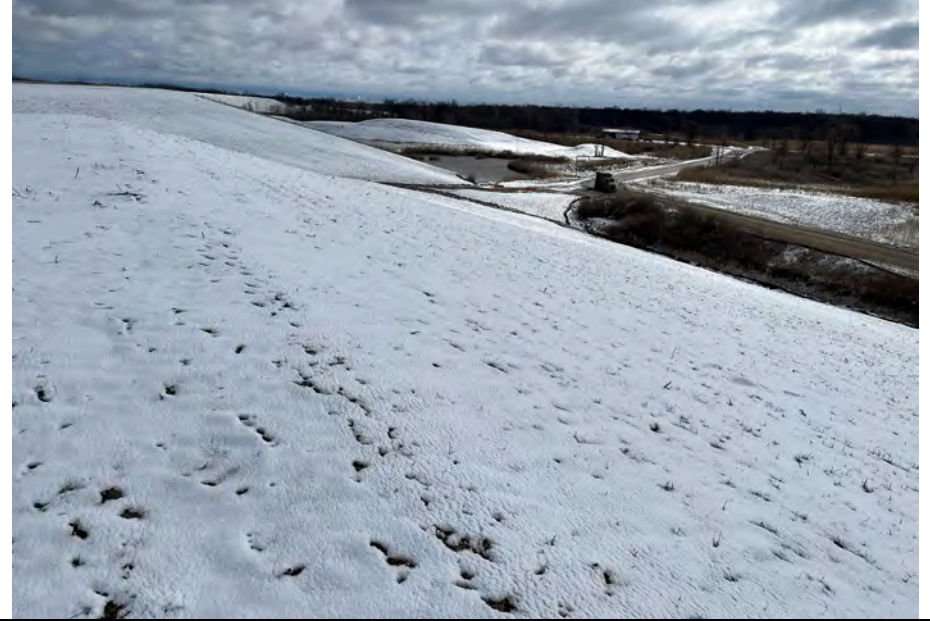
46. Light Snow Cover East Side Slopes of Areas Fe and G2 Phase 1. Slopes Appeared in Good Condition & Stable. See Erosion Gullies Shown in Photo 42.
