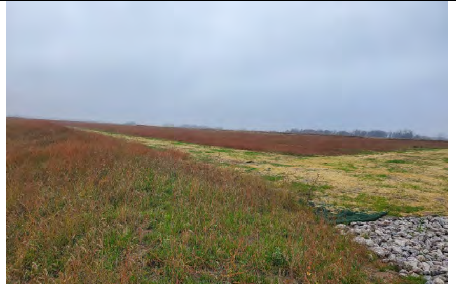
40. DTE Photo of Area G2 Phase 1 Slope Erosion Gullies Repaired and Re-Seeded in Spring 2022 after April Annual Inspection.
