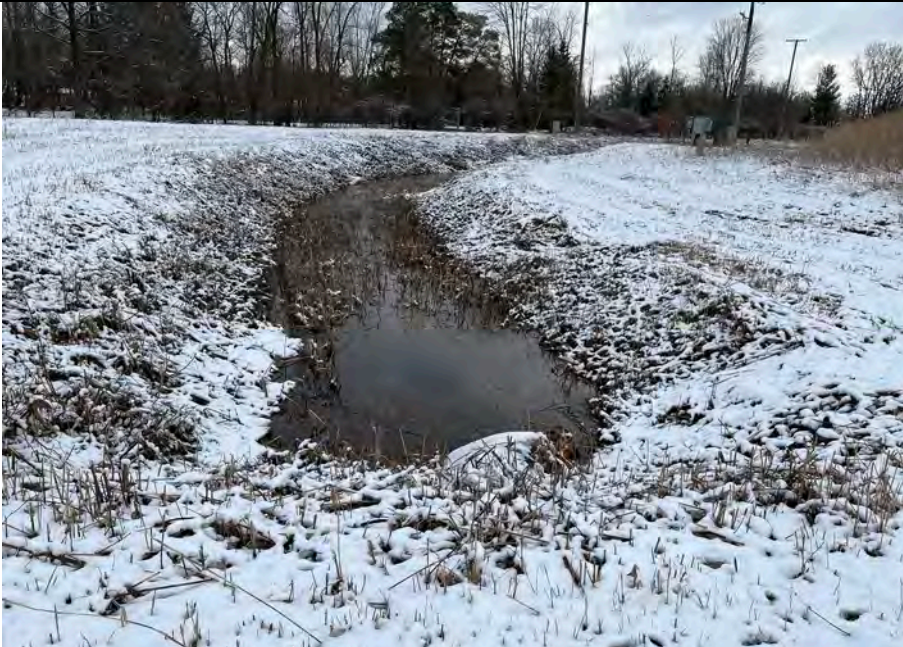
25. Ditch Open and Not Blocked but Some Vegetation Shown in Center Area of Ditch Photo. Culvert Open.
