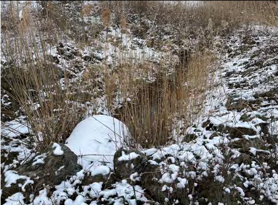
21. Bottom of Downchute Shown in Photo 22 Drains Through Culvert to Perimeter Ditch Along Perimeter Road.
