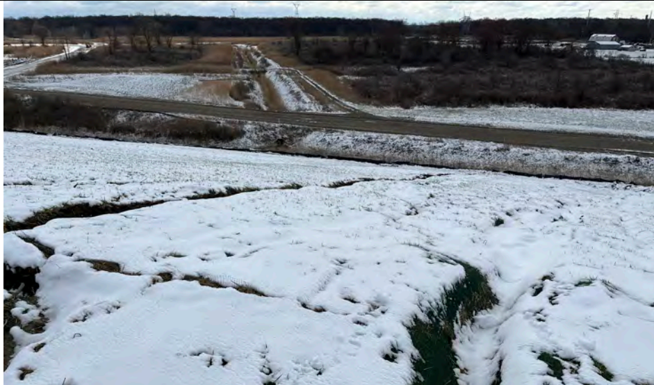
39. East Side Slope of Capped Area G2 Phase 1. Slope Erosion Gully. Cover & Slope Repair & Re-Seeding Completed in Spring. See Photos 40, 41 and 42.
