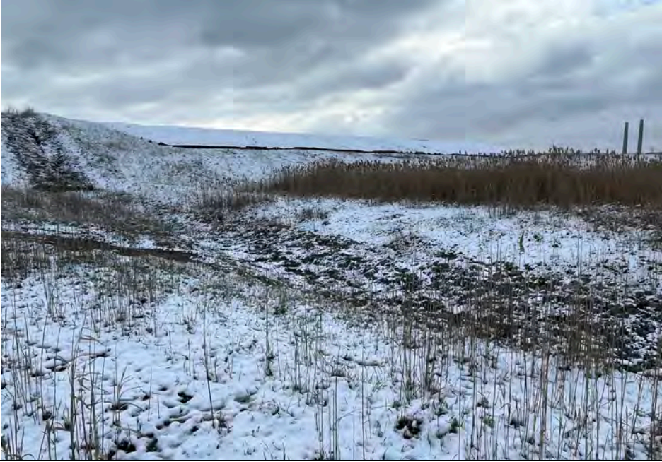
29. Downchute Located at Southwest Corner of Landfill Area F1. Chute Protected from Erosion with Riprap & Steel Mesh. Some Slope Bottom Erosion Noted.
