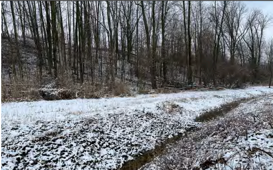
27. View of Perimeter Ditch Past Maintenance with Small Riprap Check Dam. Ditch Slope Maintenance has been Completed Previously.
