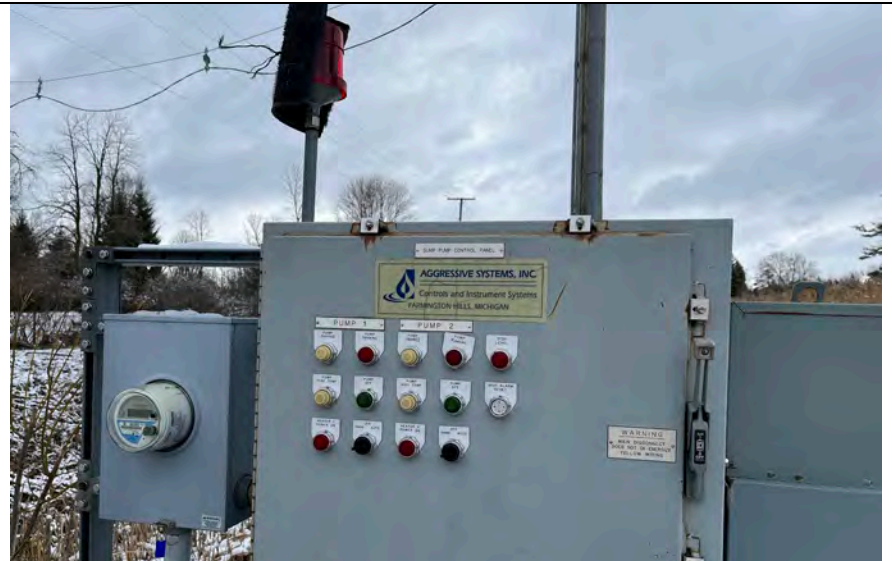
24. Neither Pump Running and in Hand Operation Per Panel Controls. DTE Inspector Manually Verified Pumps Operation. Controls Restored to Auto.
