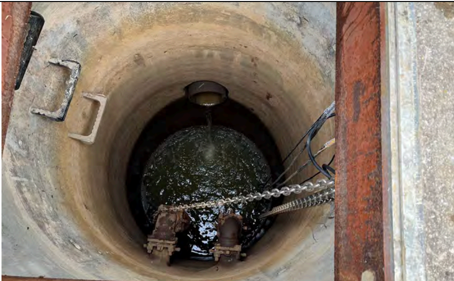
23. Sump Pumps in Manhole. New Pumps were Installed In 2018. Discharge to Culvert Connected to Ditch. Inlet Pipe Shown Little Flow.
