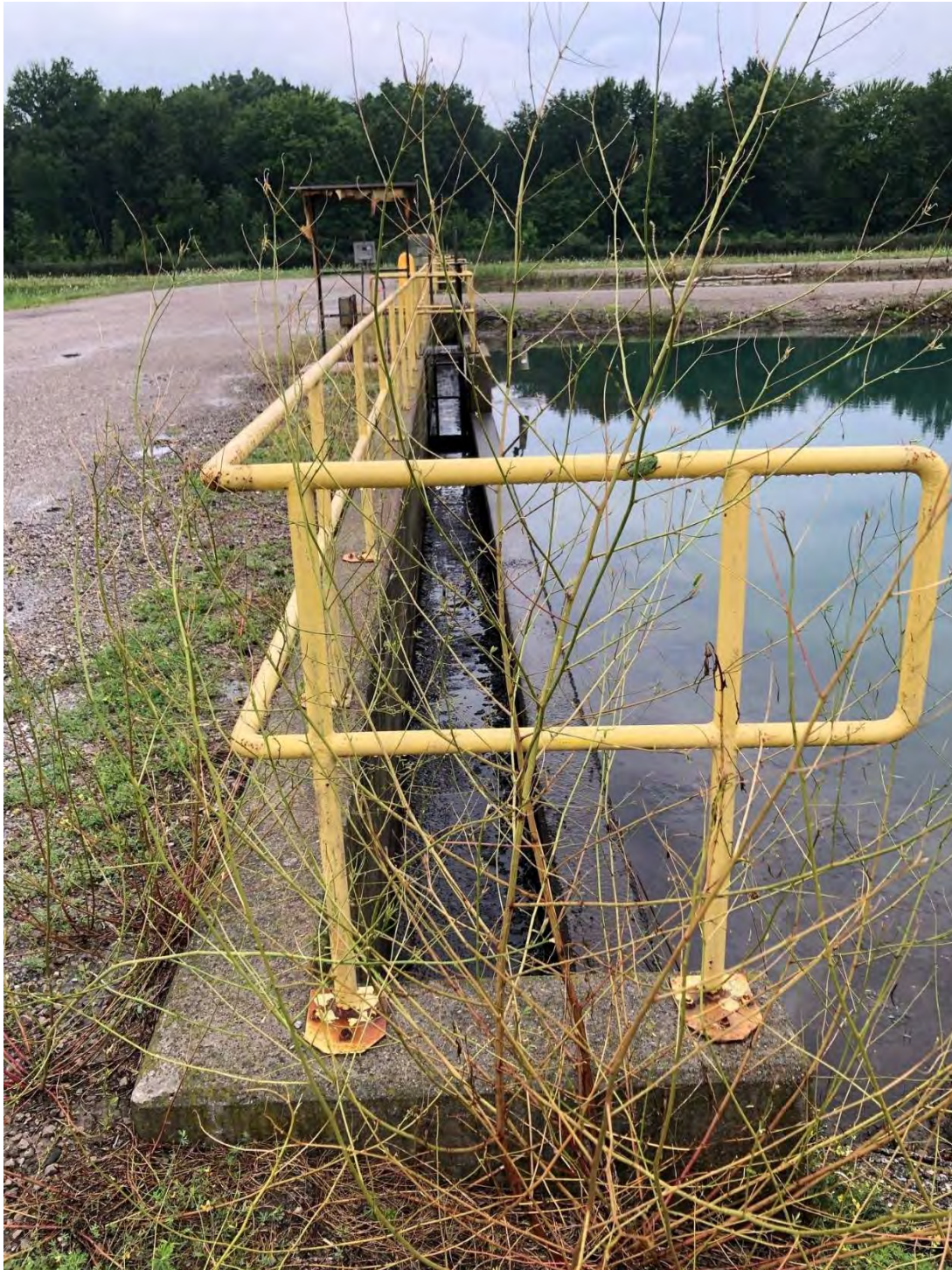
Photograph 2: Weir at the West End of the South Basin Looking Approximately North
