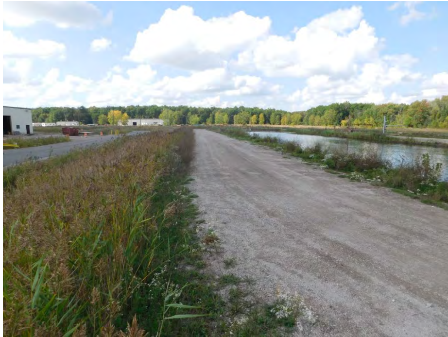
Photograph 1: South Dike of the South Basin Looking Approximately West from Near the Southeast Corner of the Dike
