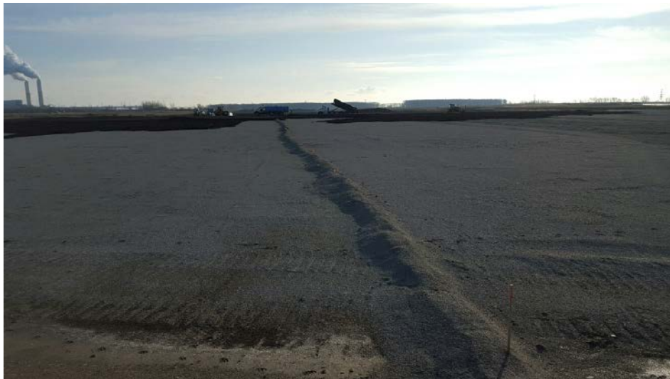
Photo 6: View of filling operations in the background with the buried instrumentation cabling for the inclinometer and piezometers in the foreground and center. Looking east.
