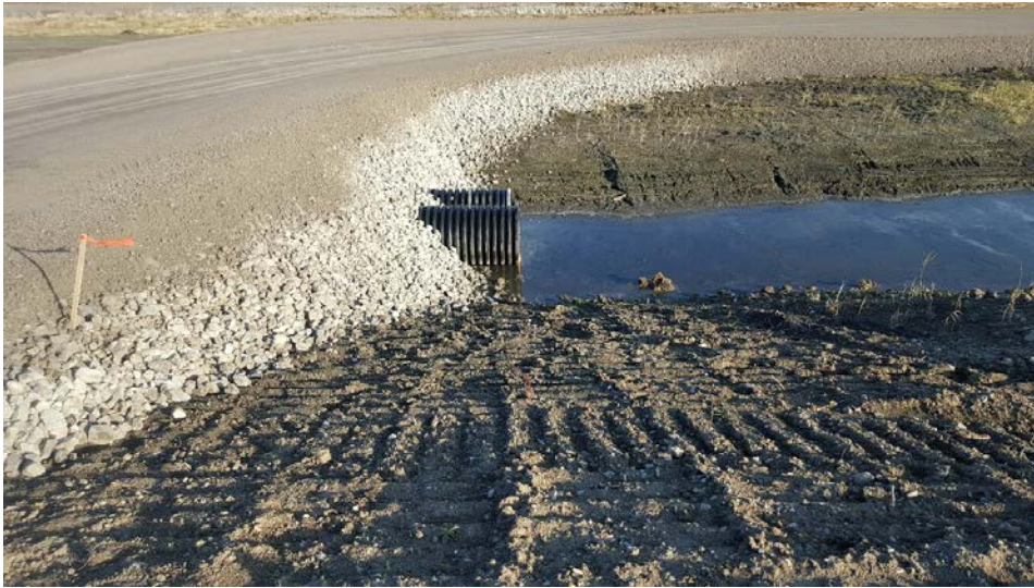
Photo 3: Surface water drainage pipes in the Perimeter Swale to convey runoff below the access road.
