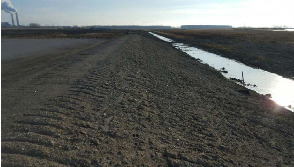
Photo 7: South Perimeter Berm looking east. Perimeter swale on the right and limestone base to the left.
