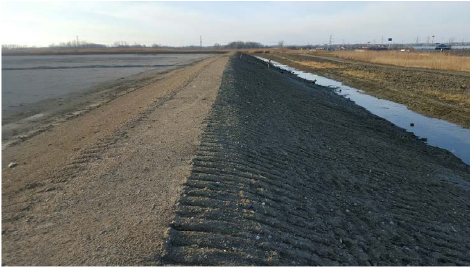
Photo 5: West Perimeter Berm looking south. The perimeter swale is to the right and limestone is to the left in Phase 1.
