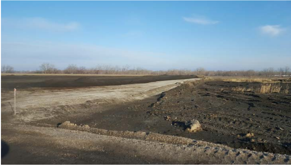
Photo 1: CCRs previously placed in Phase 1. East edge of Phase 1 shown from center left to center right.
