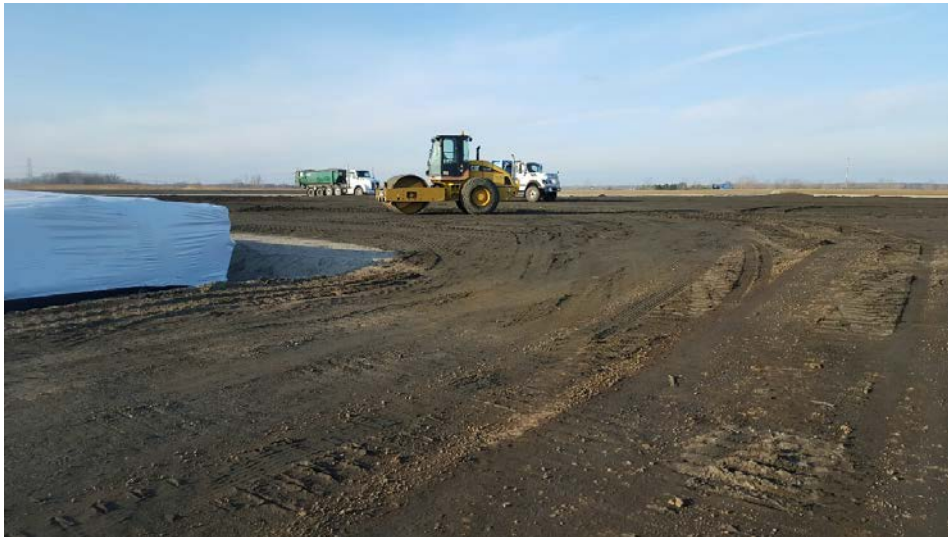
Photo 2: Trucks containing CCR placing in Phase 1 and smooth drum roller compaction equipment. Stored geotextiles under white plastic cover to the left.
