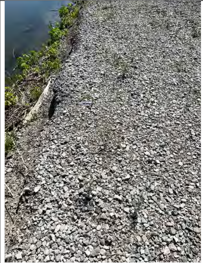
Photo 3: The south separation berm – while the area of upgraded stone placement (12-18" inches) has experienced some sloughing the berm continues to be stable at lower depths.
