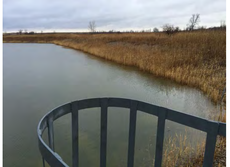
2. Storm Water Detention Basin, North and East Sides. Slopes Protected with Stone. No Visible Slope Erosion or Woody Vegetation on Slope.
