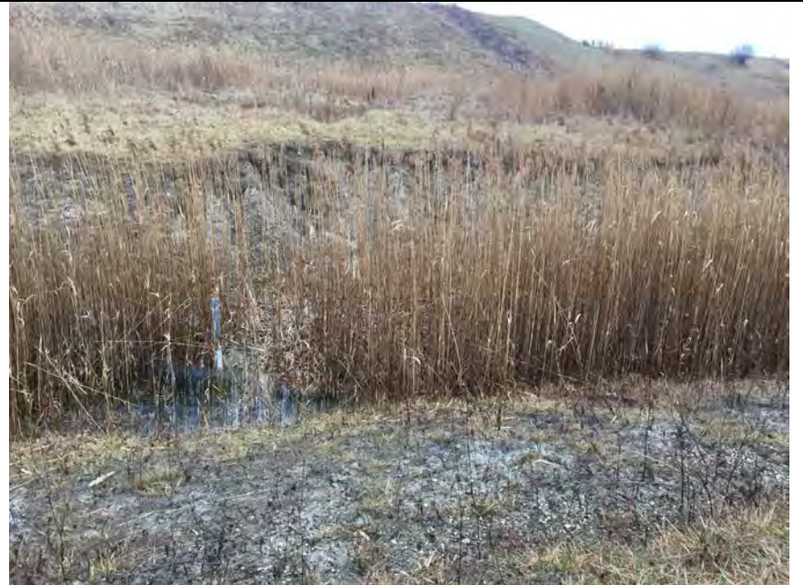
46. Location of Perimeter Ditch Staff Gauge, Believe to be SG 09. Some Ditch Slope Erosion Noted in Photo.
