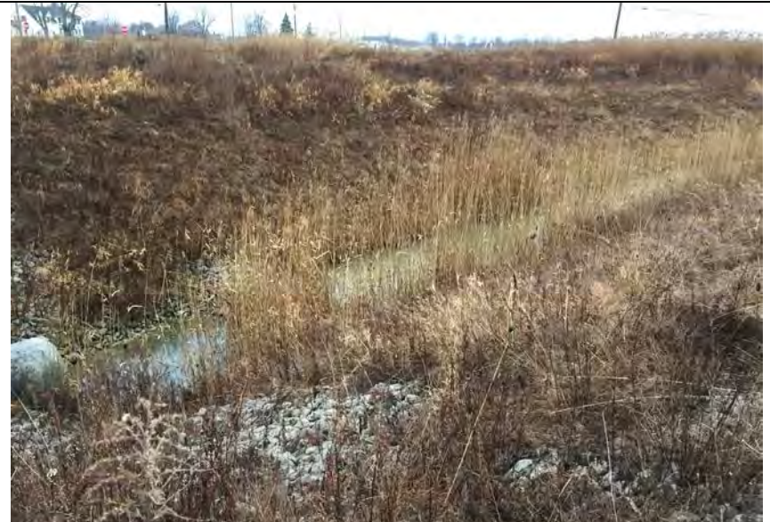
20. Looking South at Perimeter Ditch Near West Corner of Landfill. Slopes Remain Vegetated and Generally Erosion Free. Ditch Flow Observed.
