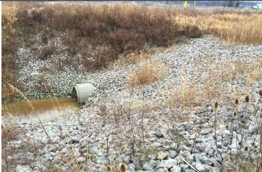
19. North End of Culvert Installed where Perimeter Ditch Located too Close to Existing Landfill Slope. No Blockage. Slurry Wall Exist Along Property Line.
