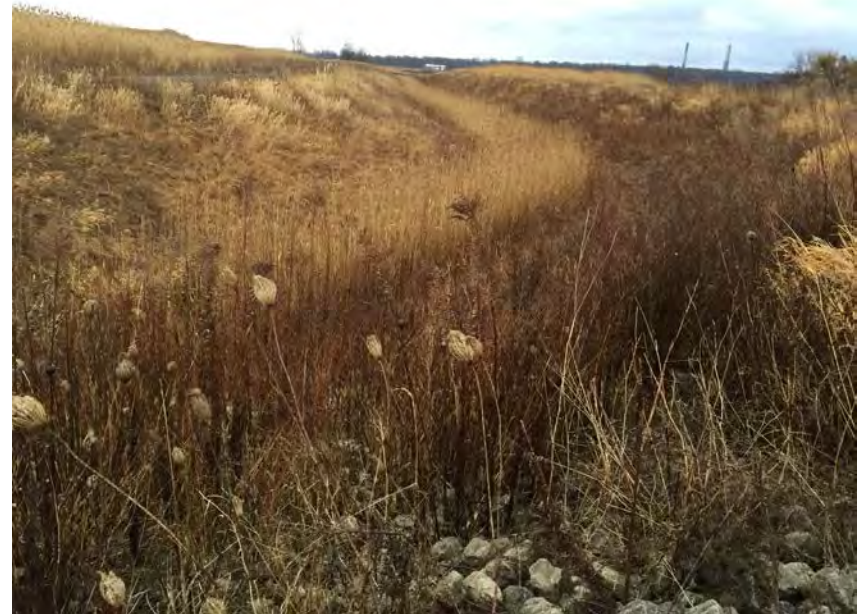
18. View of Perimeter Ditch at Road Crossing Looking Northeast. Slopes Appeared Stable and Well Vegetated. No Observed Woody Vegetation.
