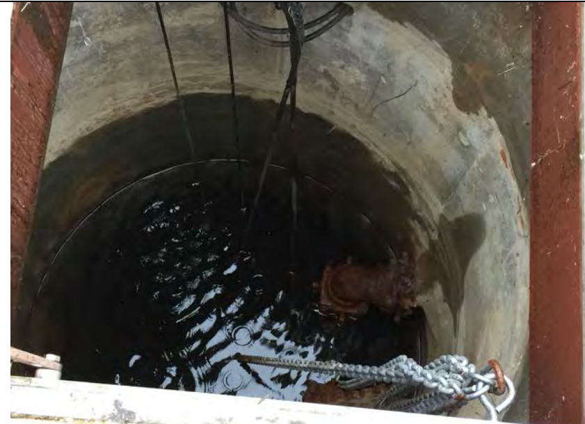
36. Sump with Discharge Pump for Northwest Groundwater Capture System.
