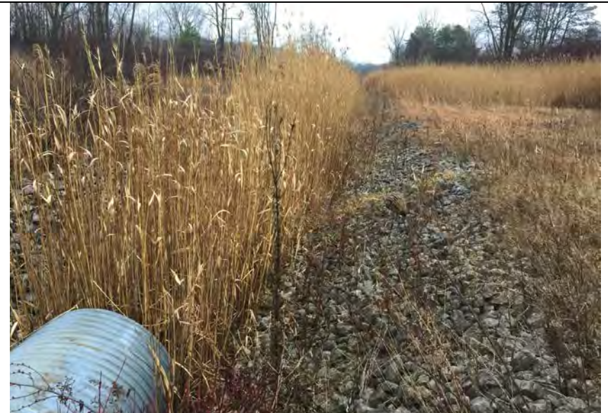
32. Looking South at Perimeter Ditch. Small Riprap Protection Provided in Several Ditch Slope Areas. Slopes were Intermittently Closely Inspected.
