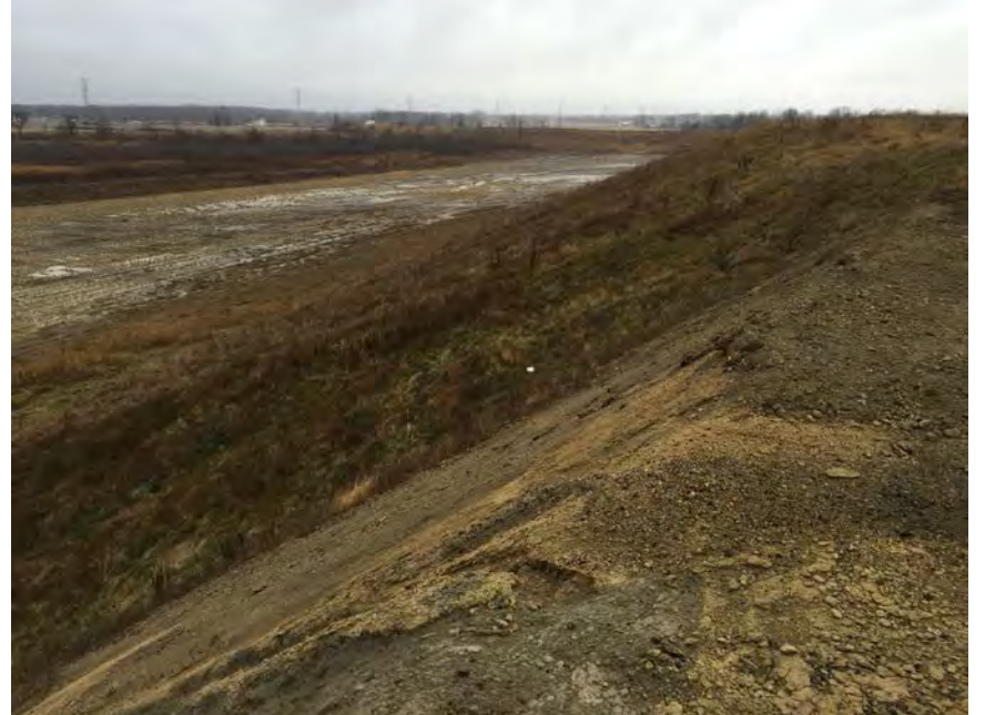
10. Borrow Area in G2. G2 Just Became Active, Approved for Placement. Drilling Confirmed Thick Layer of Clay Soils Beneath.
