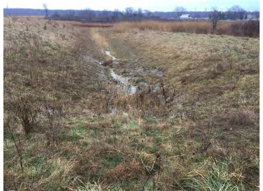
16. Culvert Drains to Existing Ditch which Connects to Ditches Draining into Storm Water Detention Basin.
