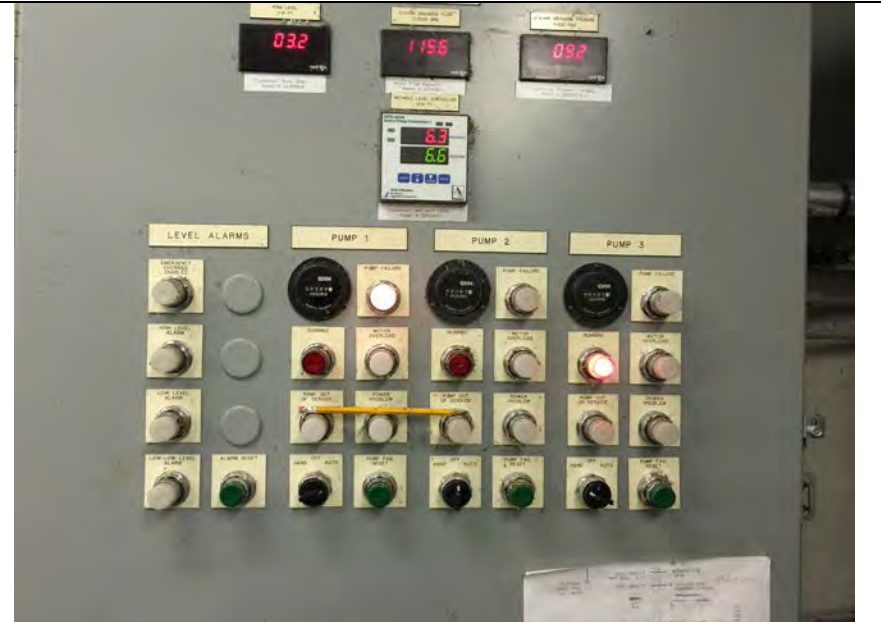
4. Pump Control Panel. Pumps were Run Checked. Pump #3 Running. Pump #1 Light Indicates Failure, but Cause was No Reset after Inspection.
