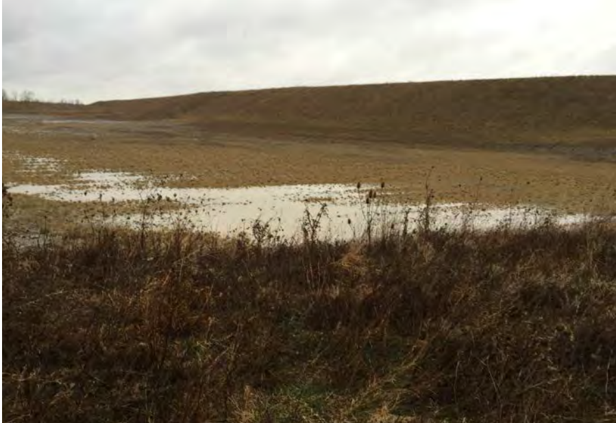
15. Another View of Completed Borrow Area in Phase G2 where Surface Water Drains to Corner Where Below Rd Culvert has been Installed to Drain East.
