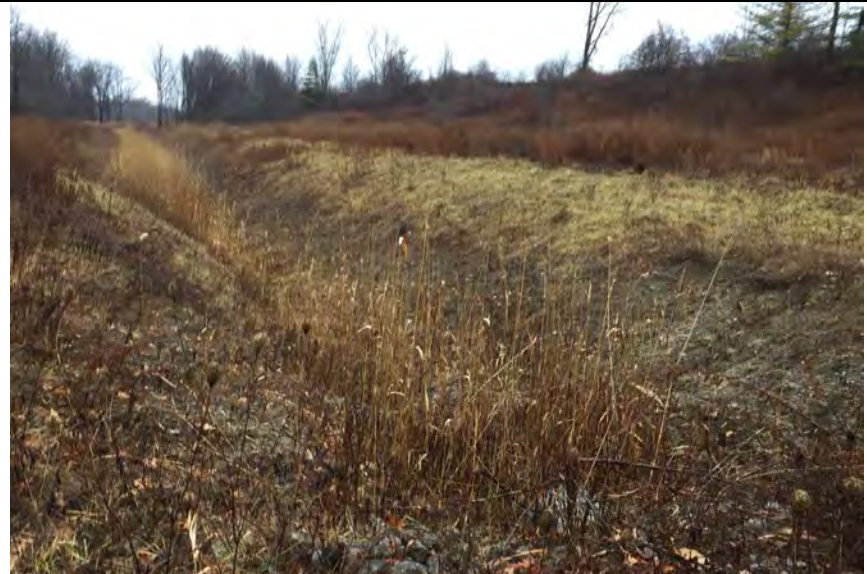
40. Perimeter Ditch Along North Side of Landfill. Road Crossing and Culvert Shown was Open for Flow (Lower Right in Photo).
