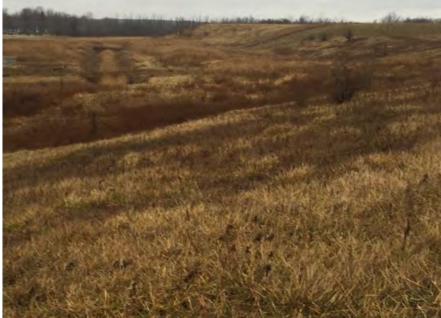
21. West Southwest Side of Landfill. Slopes Well Vegetated and Stable with No Significant Areas of Slope Erosion. Perimeter Ditch w/2 Road Crossings Shown.
