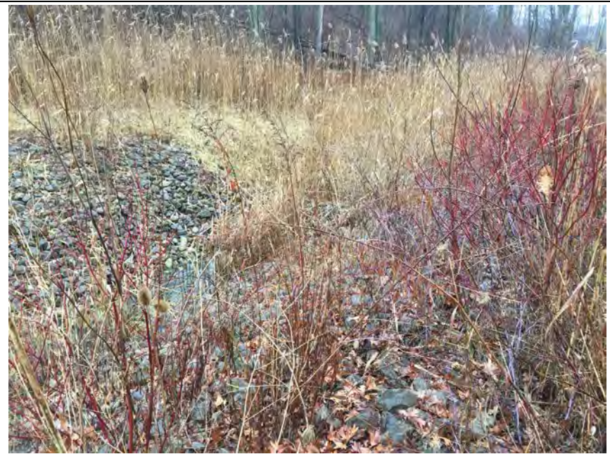
38. Riprap Along Perimeter Ditch at this Location Near NW Capture System. Riprap Placed in Several Locations Especially Near Culverts.
