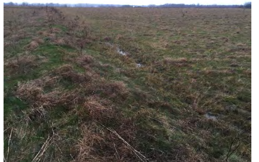
12. Final Cover Temporary Clay Berm at Top of Phase 2 Controlling and Directing Surface Runoff at Boundary with Phase G2.
