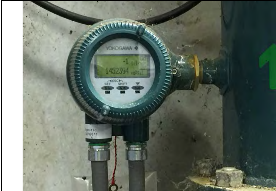
5. Pump System Discharge Rate & Total Meter in Gal/Min and Gallons. Total Recorded Daily on Day Shift Report.
