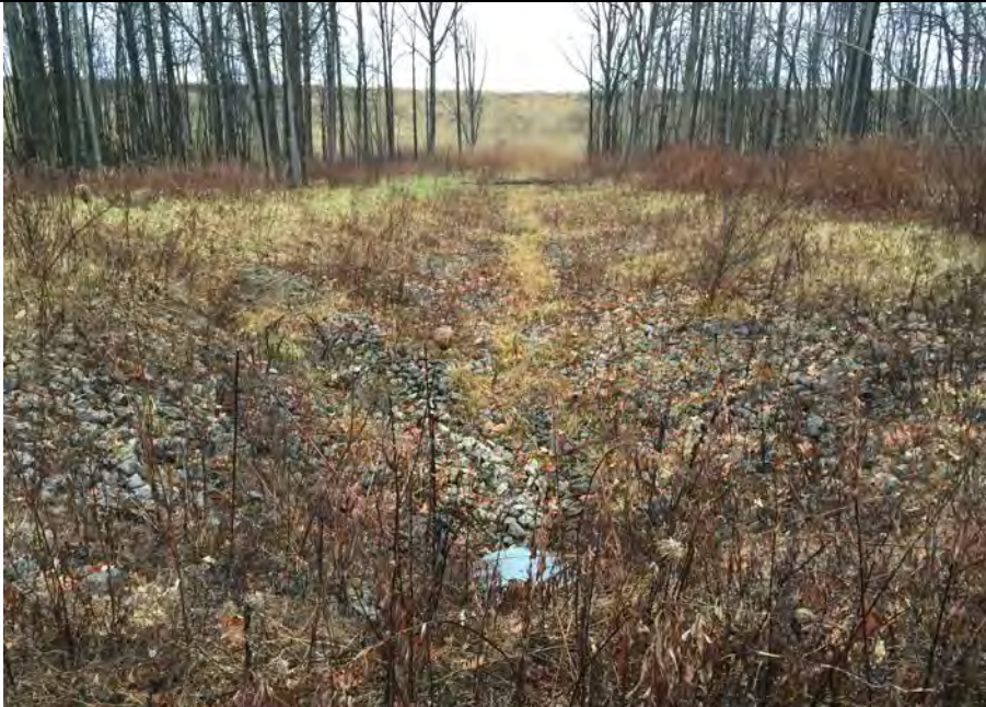
41. Culvert and Secondary Ditch Perpendicular to Landfill Slope. Fallen Tree Across Ditch.
