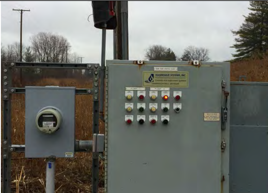
37. Northwest Groundwater Capture System Sump Pump Control Panel. Pump No. 2 is Running. Running was Verified for Pump Nos. 1 and 2.
