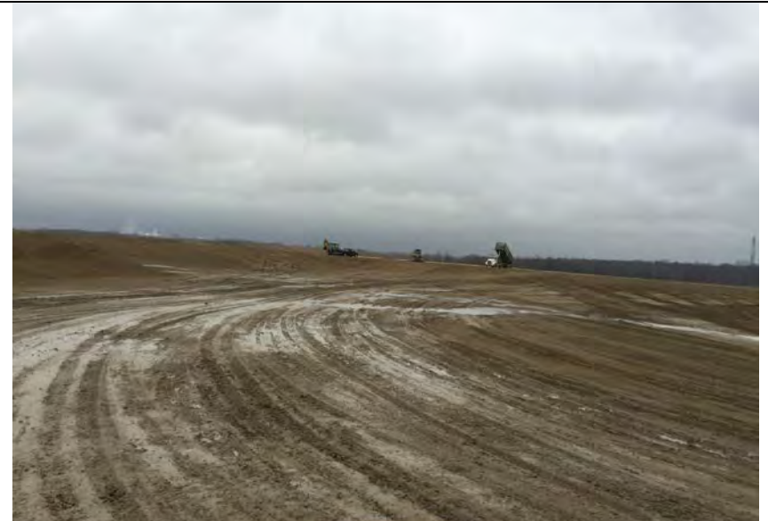
8. Entrance to Active Landfilling Areas over Unconstructed Phase G3 and E Areas. Light Rain (0.38 in) During Inspection. Temperature Reported 48°F.
