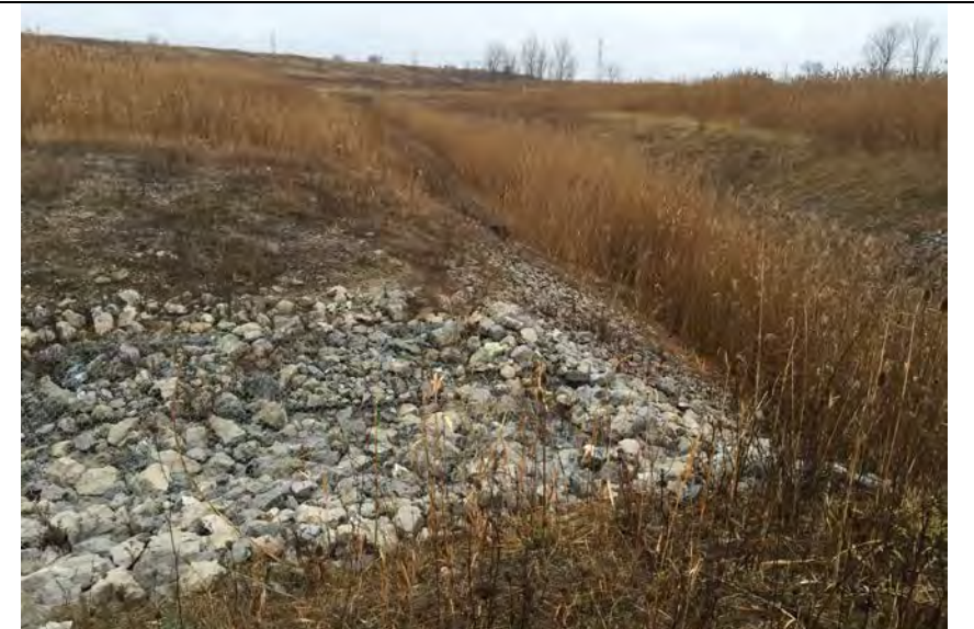
48. Looking South Along Perimeter Ditch Toward Southwest Corner and Fenced Area. Some Woody Vegetation of Landfill SW Berm W of Area G2.
