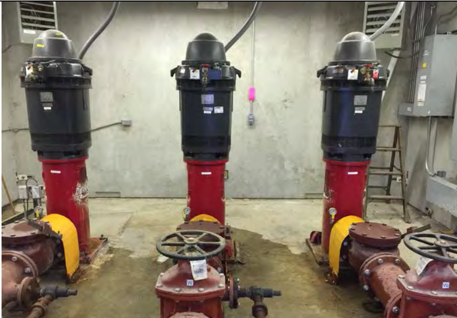
3. Pump House Pumps and Valves. Water from Basin is Pumped Back to Power Plant. DTE Plant Inspects Daily and Records Pump Observations.
