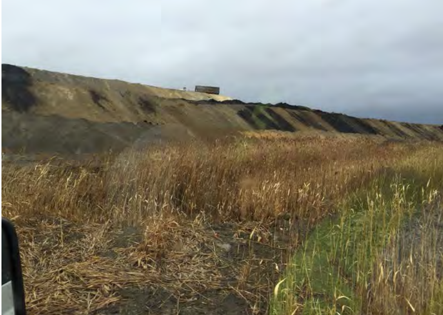
9. Face of Active Placement in Landfill Phase F3. Placement from Top and Bottom. Small Runoff Collection Pond in Center of Photo.
