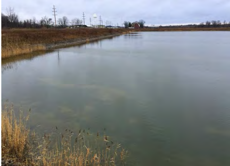
1. Storm Water Detention Basin, South and West Sides. Slopes Protected with Stone. No Visible Slope Erosion or Woody Vegetation on Slope.
