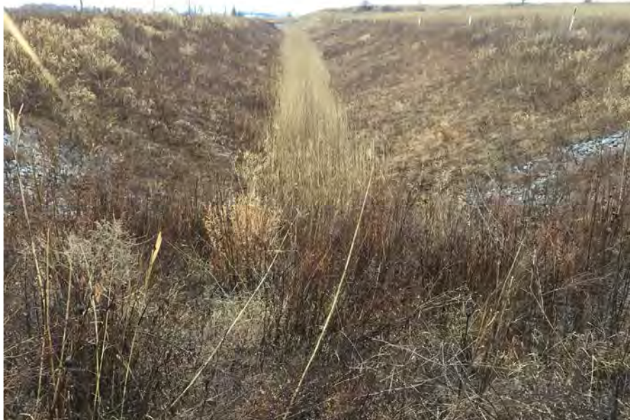
17. Looking West at Perimeter Ditch Parallel to Puttygut Road. Ditch Slopes were Reconstructed in 2010 and Remain Stable and Visually Erosion Free.
