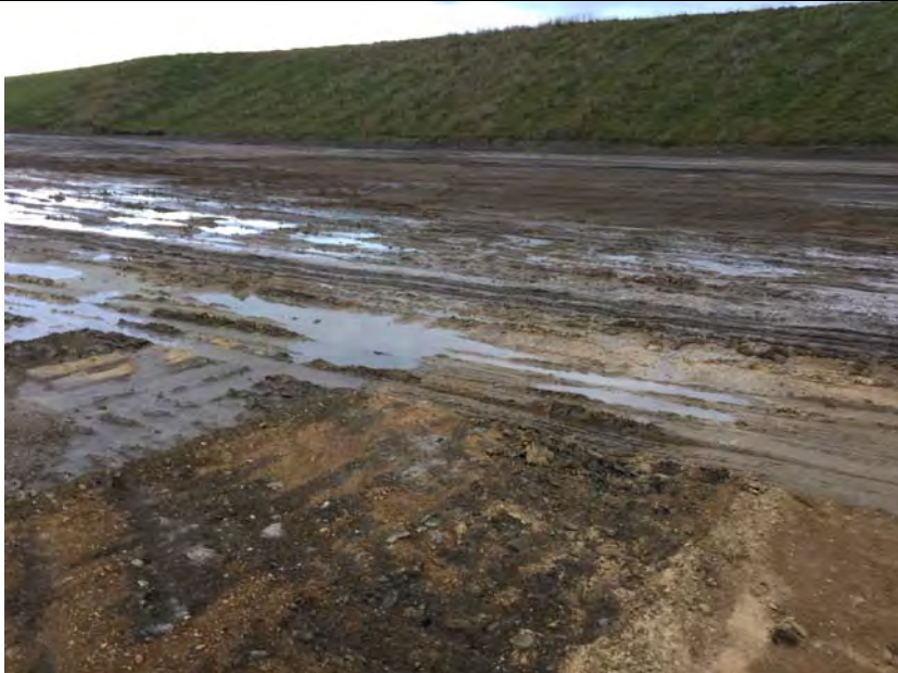
15. Another View of Ash Bottom of Area G2 North End Along Area F2 Temporary Slope.
