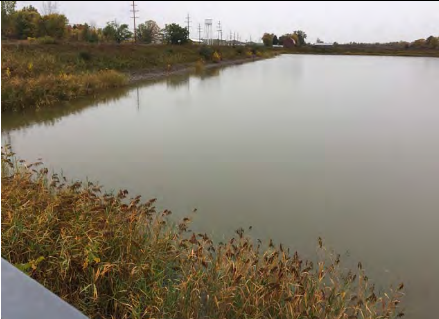
1. Storm Water Detention Basin (SWDB), South and West Sides. Slopes are Protected with Stone. No Visible Slope Erosion or Woody Vegetation on Slope.
