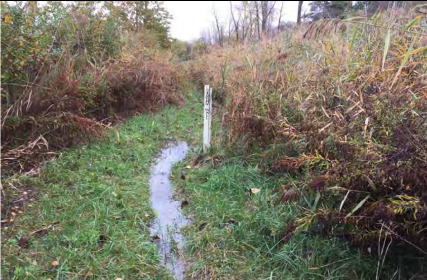
43. Typical Slurry Wall Marker. Roadway/Walkway Along Perimeter Ditch. Ditch on the Right. Fence on the Left.
