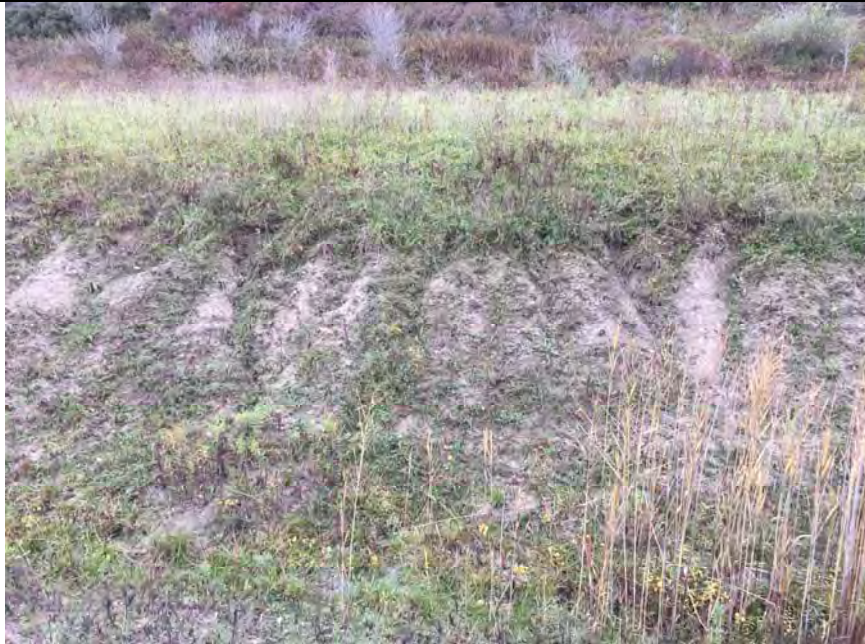
37. Close-up of the Ditch Scheduled for Stone Slope Repair. Erosion Noted and Past Vegetation Seeding Did Not Take Hold.
