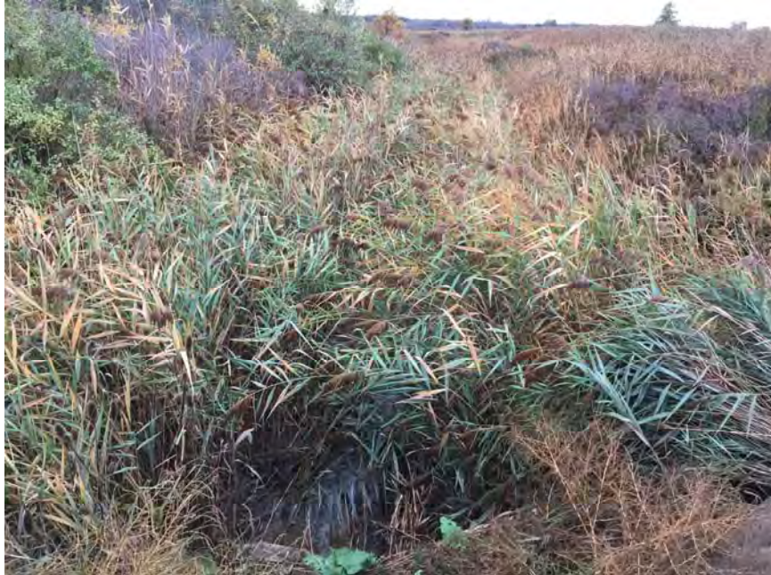
13. View of East End of Concrete Culvert Beneath Haul Road Crossing Ditch West of Area F3 Shown in Photo 12.
