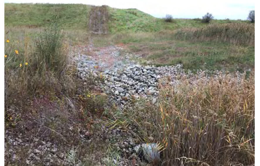
48. Looking East at Drainage Flume as it Enters Perimeter Ditch. Some Woody Vegetation on Outside Existing Slope from Active Area G2.
