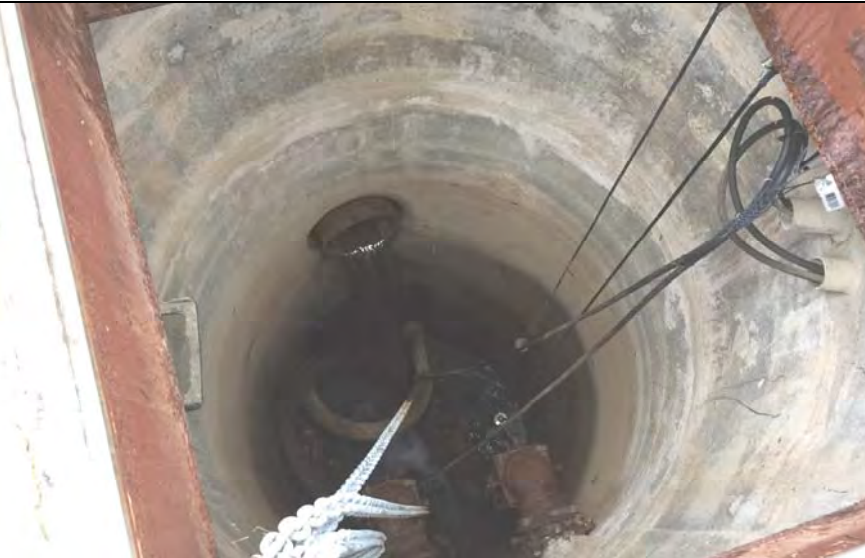
39. Sump Observed at NW Pump Control Location. Water from Offsite Wells is Trickling in.
