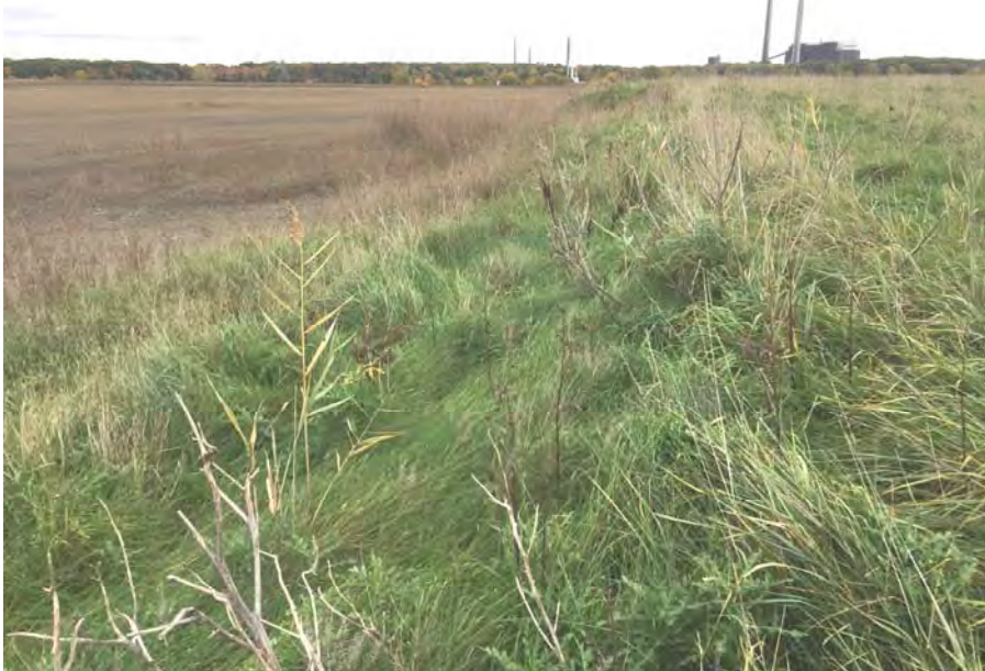
29. Top of Landfill Looking at Drainage Berm. Active Area F3 on Left. No Berm Erosion Noted.
