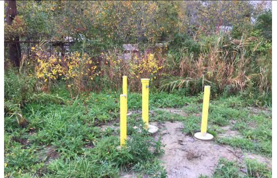
56. New CCR MW 16-04 Located at NE Corner of Property Outside of Slurry.
