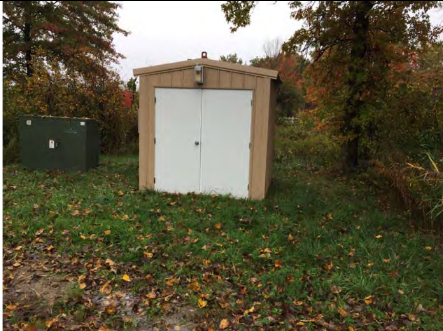
9. Northeast Off-Site Groundwater Capture System Building. Capture System Inspected Routinely and Sumps Not at this Location Inspected and Cleaned.
