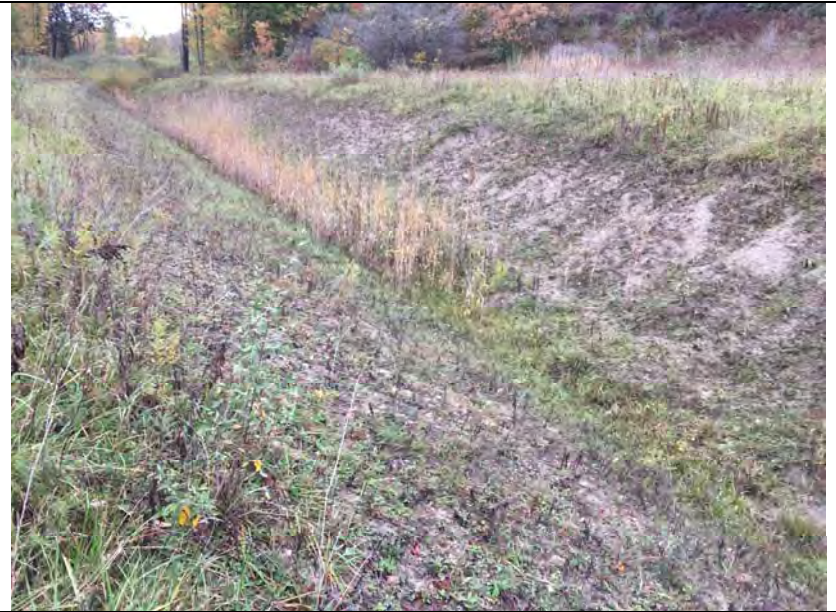
36. Perimeter Ditch Along North Side That is Scheduled for Stone Slope Protection.
