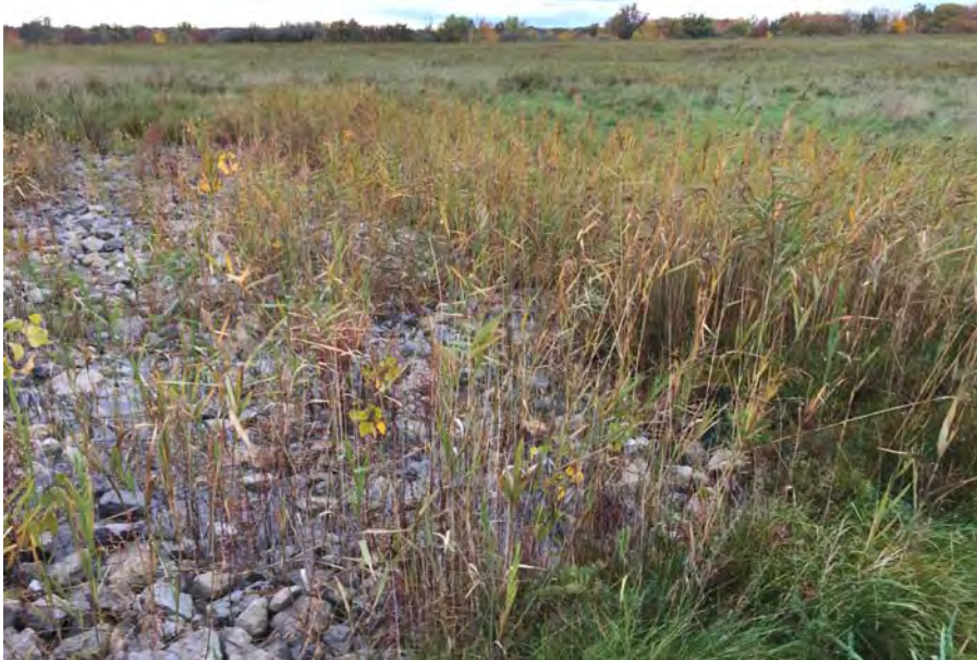
25. Top of Landfill at Beginning of Downslope Drainage Flume at Closed Areas F1 and F2 Corner.
