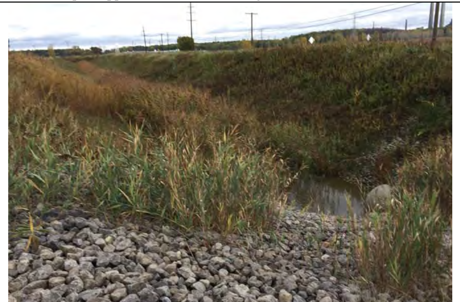
20. Perimeter Ditch at Road Crossing on South Side. Flow was Observed Through the Culvert.
