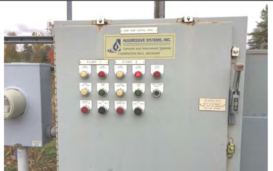
40. NW Pump Station Control Panel in Operation. Pump #2 Running.
