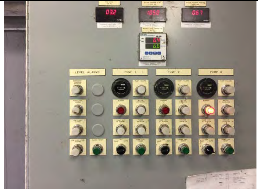
4. Pump Control Panel. Each Pump was Run Checked. Pump #3 Running. Pumps Cycle Each Run Unless Higher Pond Level Needs More Pumps On.
