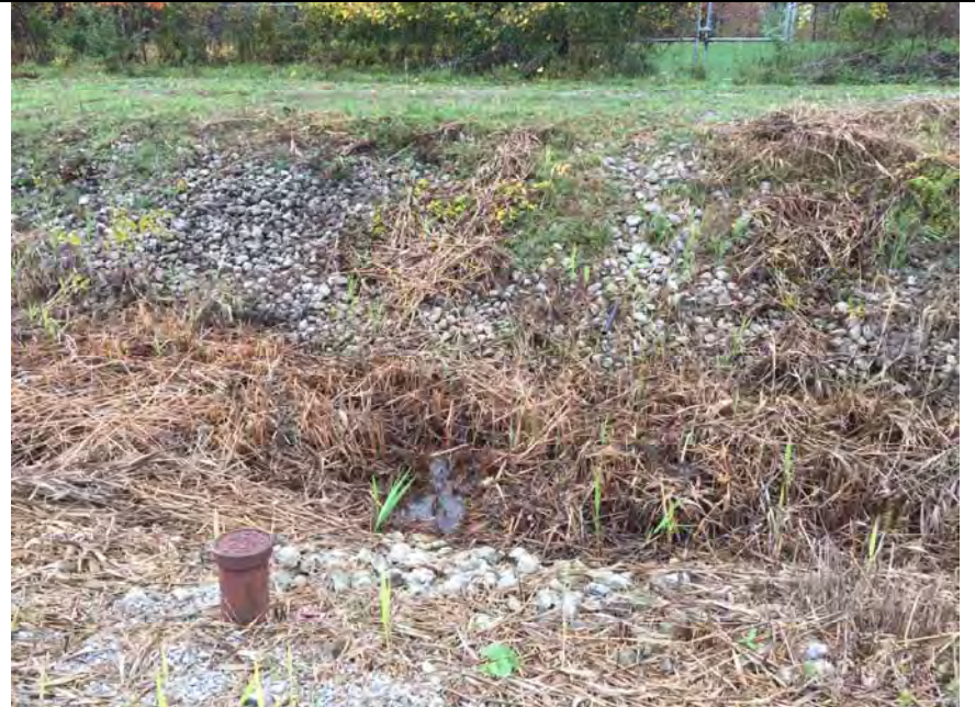
38. Location of Discharge from Sump to Perimeter Ditch. Flow was Observed. Pump #2 was Pumping as Control Panel in Photo 40 Indicates.
