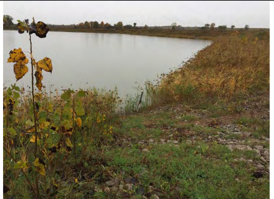
2. Storm Water Detention Basin, North and East Sides. Slopes are Protected with Stone. No Visible Slope Erosion or Woody Vegetation on Slope.
