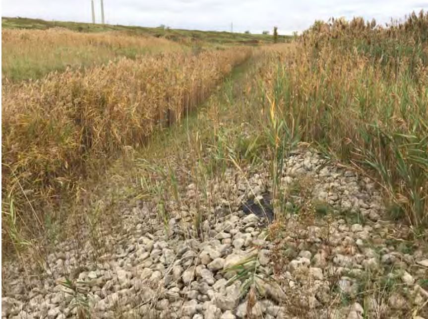
49. Looking South at Close-up of Perimeter Ditch. A 3-year Rotation Ditch Maintenance Schedule is Planned by DTE.
