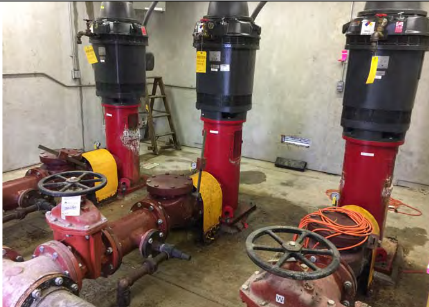
3. Pump House Pumps and Valves. Water from Basin is Pumped Back to Power Plant. DTE Plant Inspects Daily and Records Pump Observations and Flow.
