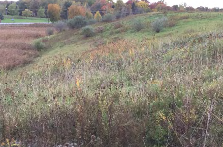
23. Looking at d/s Slope of Closed Area F1 where Small Woody Bushes/Trees Developing. Woody Vegetation was Scheduled for Removal.
