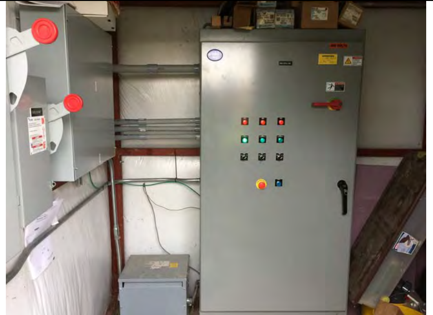
10. Inside of NE Off-Site GW Capture System Building. Pump #1 (Left Green Light On) Running. Water Discharging to Ditch During Inspection.
