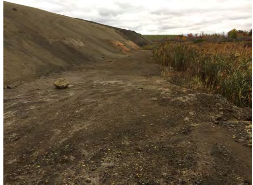
12. View of Active Area F3 East Slope. Drainage Ditch Right Side of Photo.
