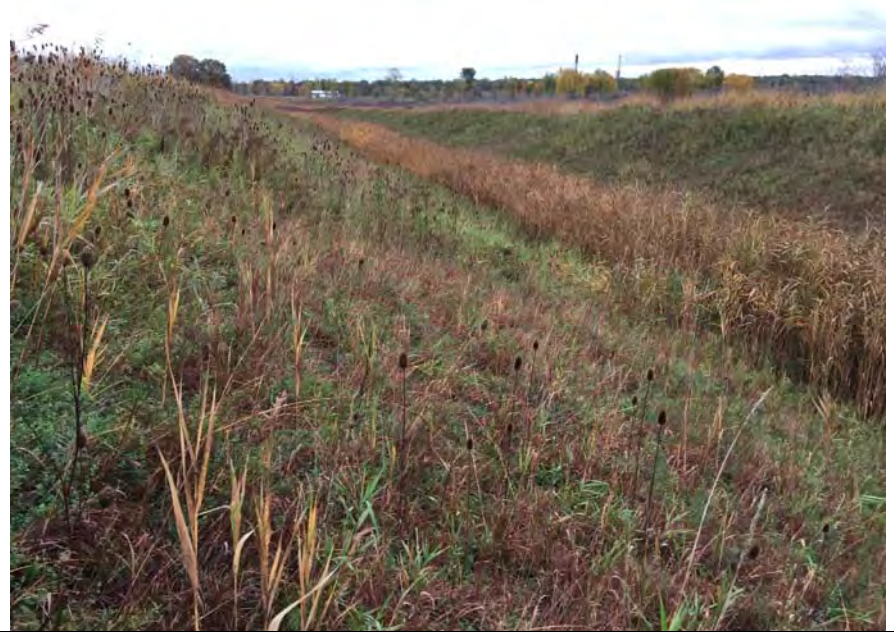
18. View of Perimeter Ditch Along South Side that was Reconstructed in 2010. Slopes Appeared Stable, Well Vegetated and Erosion Free.
