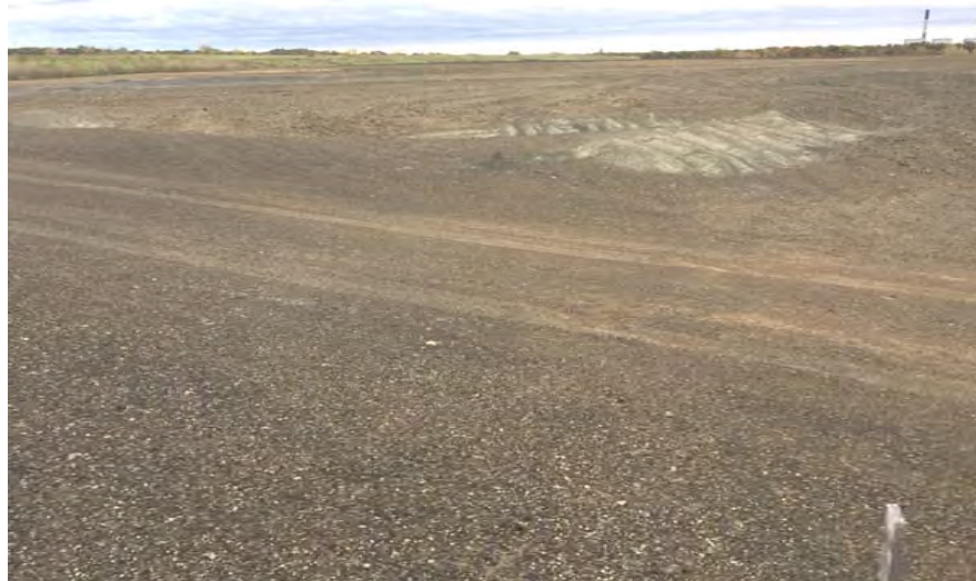
27. Looking North at Top of Active Area F3 Where Surface Being Graded for Final Cover.
