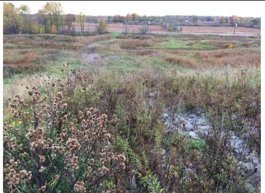
22. Ripped Downslope Drainage Flume Central West Side of Landfill at Corner of Closed Areas F1 and F2.
