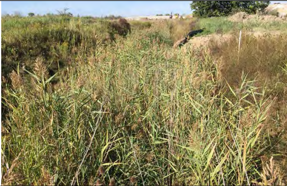
35. Internal Drainage Ditch Filled with Vegetation.
