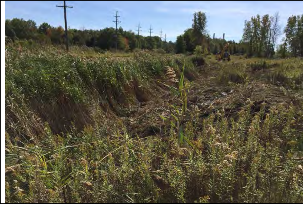
53. Ditch Maintenance and Vegetation Removal In progress. Equipment Shown Currently Under Repair or Maintenance.
