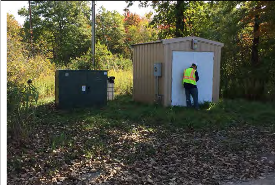
9. Northeast Off-Site Groundwater Capture System Building. Capture System Building Controls Inside were not Inspected Due to Wrong Key Available.
