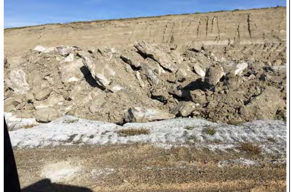
16. Closeup View of Cemented Chunks of Waste. Some Soil Mixed In. Chunks are Planned to be Broken-Up and Placed & Compacted.
