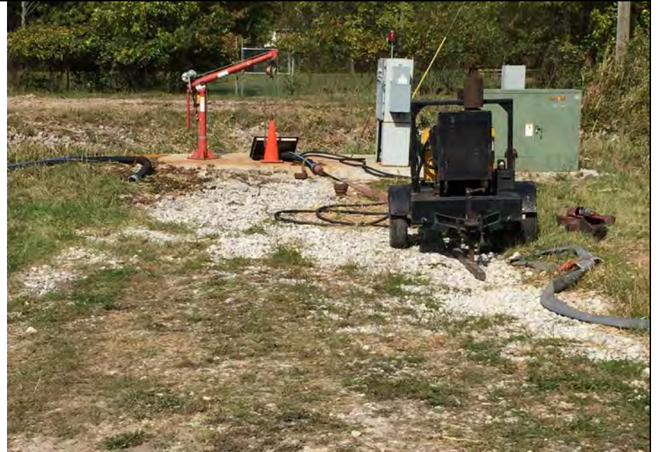
62. Pumps in Sump at NW Groundwater Capture System are Being Replaced. Contractor Temporary Pump Used to Remove Water from Sump.
