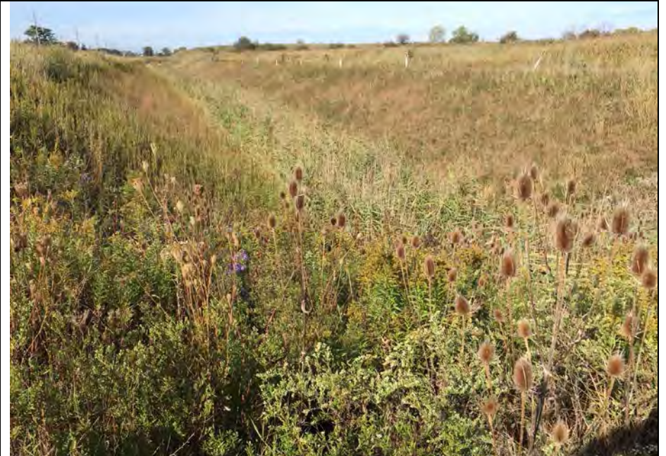
26. View Looking West at Modified Perimeter Ditch. G2 Survey Stakes Right Side Slope. White Markers Along Top of Slope at Road for Safety.
