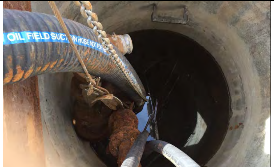
64. Sump at NW Groundwater Capture System with Old Pumps Partially Removed. New Pumps to be Installed in October 2017, per DTE.
