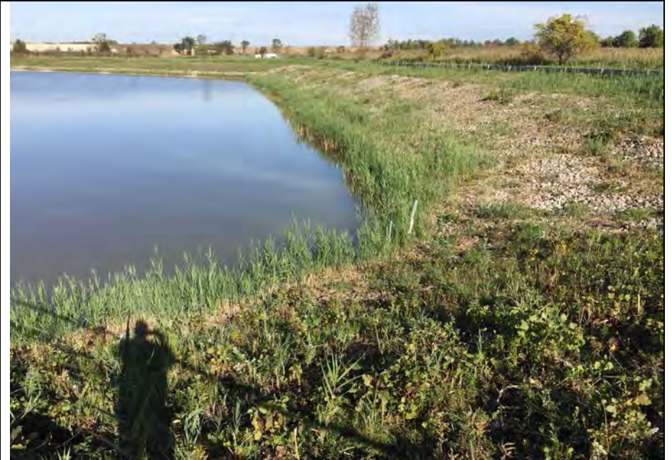
2. SWDB, North and East Sides. Slopes are Protected with Stone Within Water Level Range. No Visible Slope Erosion. Vegetation Cut on Slopes.
