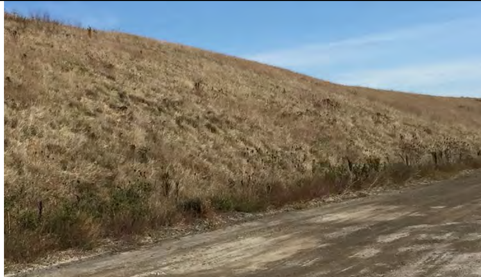
39. View of Slope of Closed Area C. Slope Well Vegetated and Appearing Very Stable.
