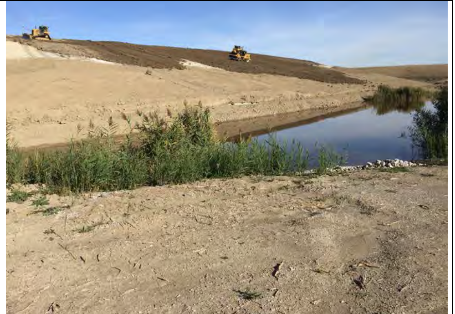
10. Looking NW at Cover Placement on 4H to 1V Interim Slope of Area F3. Waste Placement & Compaction to Construct Slope is from Bottom Up.
