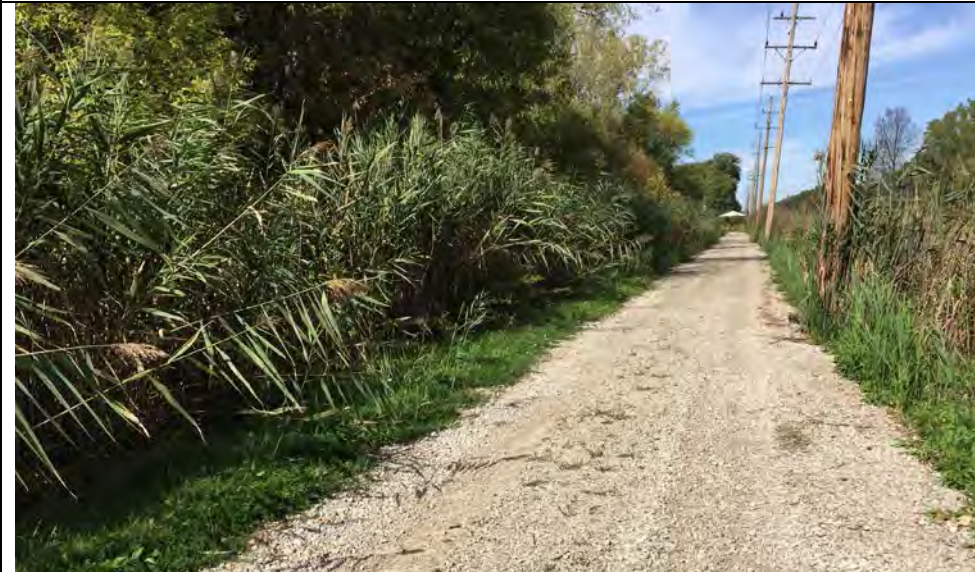
51. Perimeter Road Along East Side Maintained. Perimeter Ditch Along Left Side and Slurry Wall Alignment Beneath Road in this Photo.
