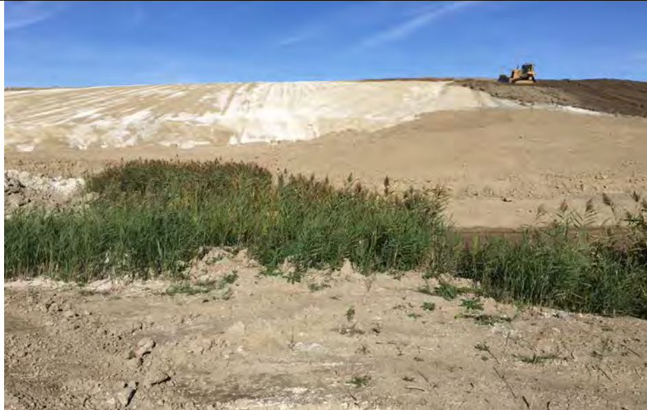
11. Looking North at Interim Slope of Area F3. Slope Reported to be 4H to 1V or Flatter.
