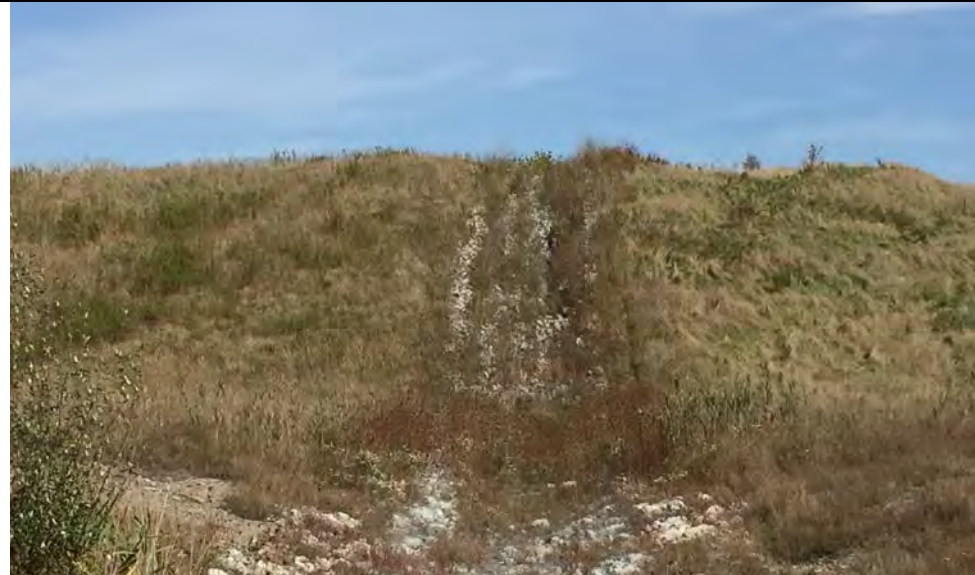
67. Looking at Slope Downchute From Intersection of Closed Areas F1 and F2. Some Runoff Erosion in Riprapped Area. Downchute Drains to Perimeter Ditch.
