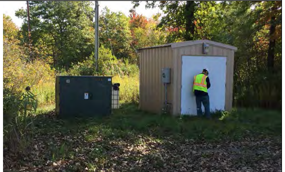
44. Offsite Groundwater Capture System Building. Controls Inside were not Observed as Door Remained Locked. No Issues Reported in DTE Reports.
