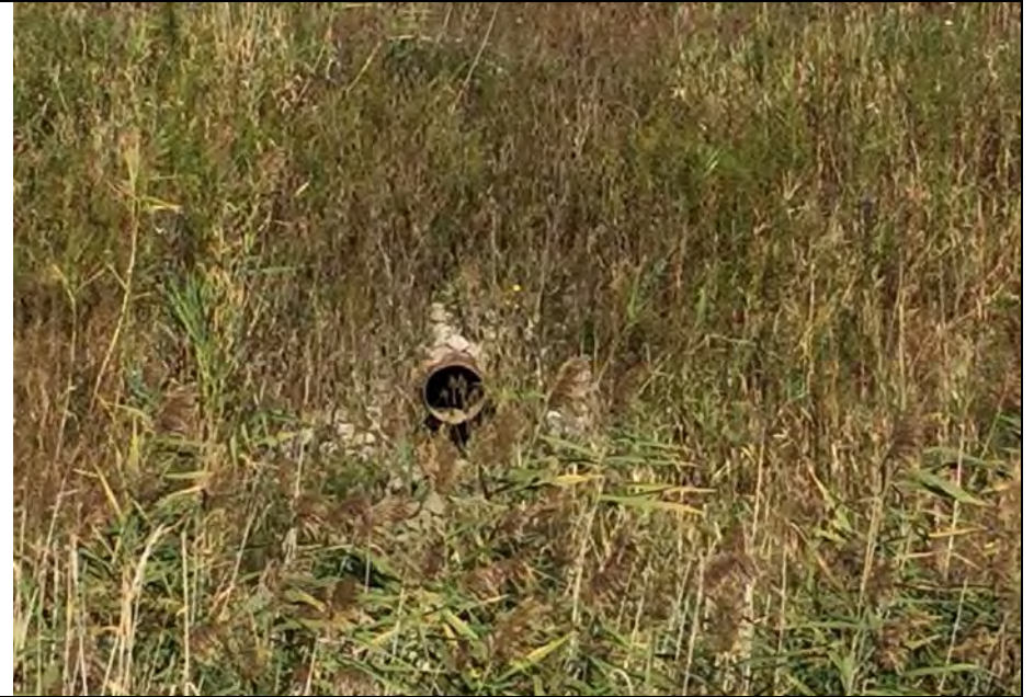
30. Close-up View of Drainage Pipe Discharging into Perimeter Ditch. Some Small Stone Riprap Protecting Slope. Protection Appeared Satisfactory.
