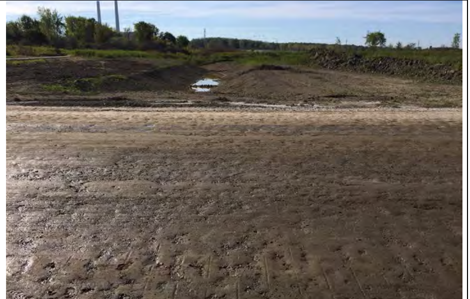
12. View of Active Clay Borrow Area from Top of G2 Fill Area.
