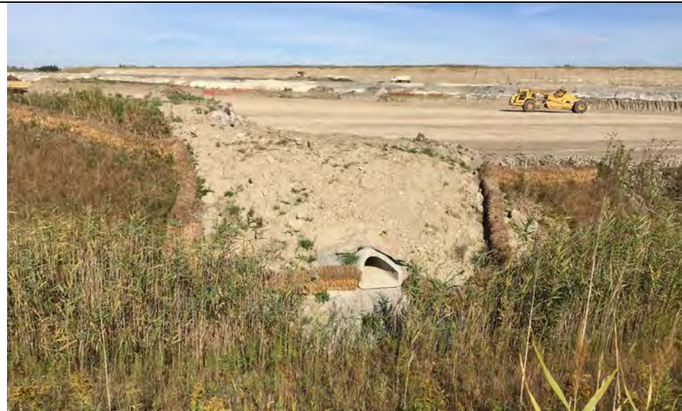
31. Culvert Flare Draining Surface Water to Perimeter Ditch from a G2 Borrow Development Area.
