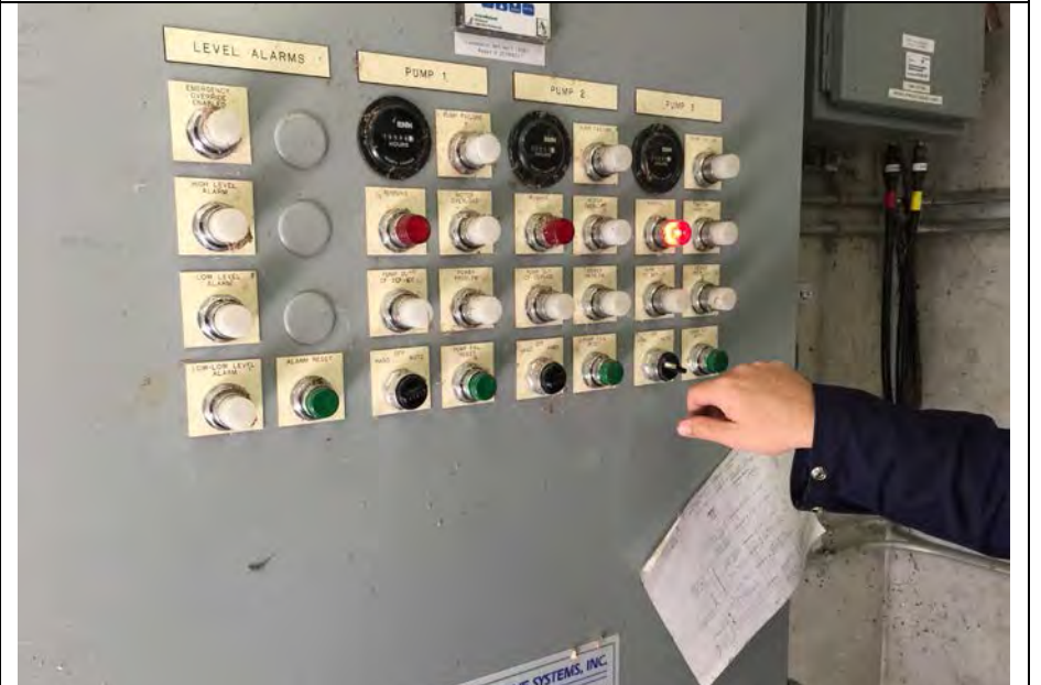
4. Pump Control Panel. Each Pump was Run Checked. Pump #3 Running. Pumps Cycle Each Run Unless Higher Pond Level Needs More Pumps On.
