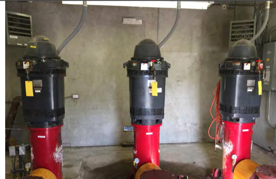
3. Pump House Pumps. Water from Basin is Pumped Back to Power Plant. DTE Plant Inspects Daily and Records Pump Observations and Flow.
