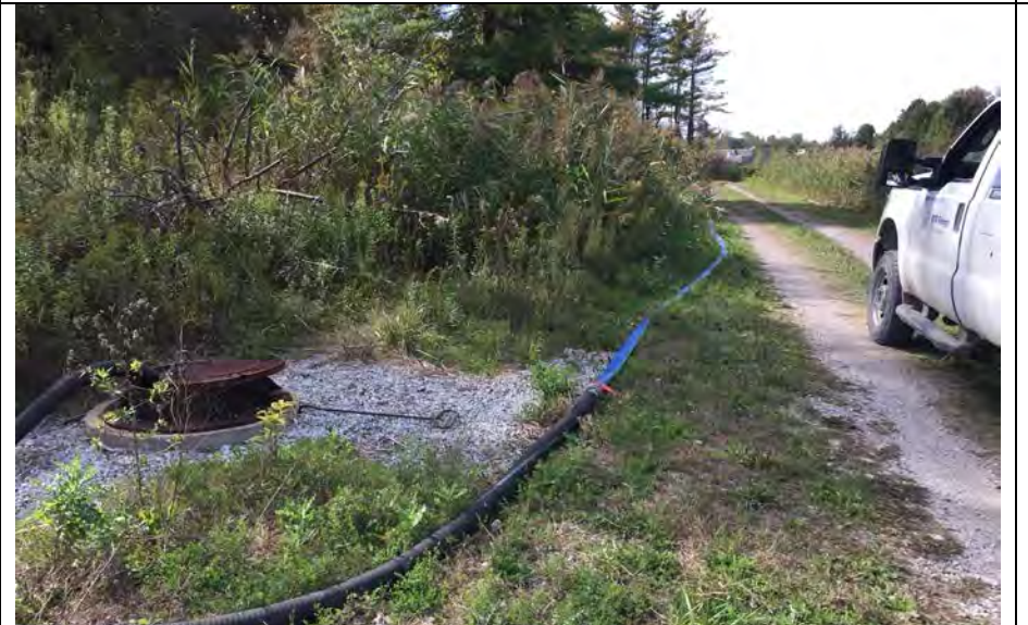
60. Sump Collecting Pumped NW Groundwater that then Drains by Pipe to Perimeter Ditch on Other Side of Truck.
