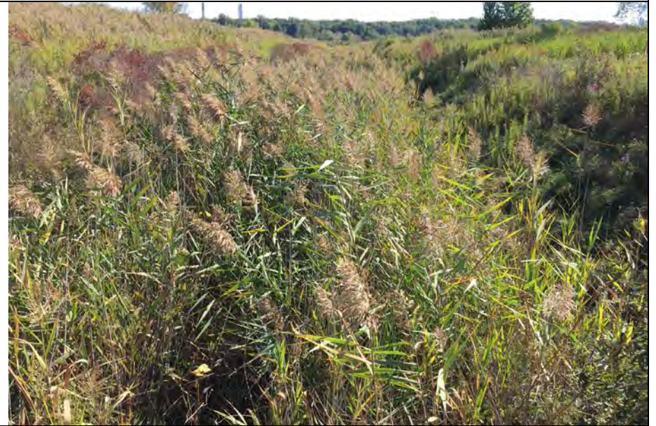
36. Internal Drainage Ditch Filled with Vegetation.
