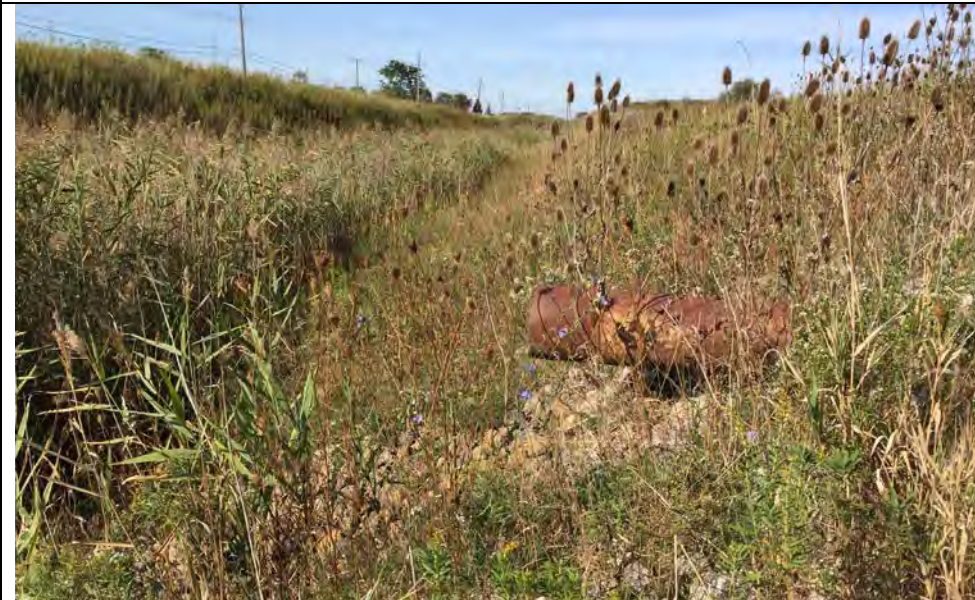
23. Looking East Along Inside Slope of Perimeter Ditch Where Drainage Pipe Enters and Slope Protected by Riprap. Slope Protection Appeared Satisfactory.
