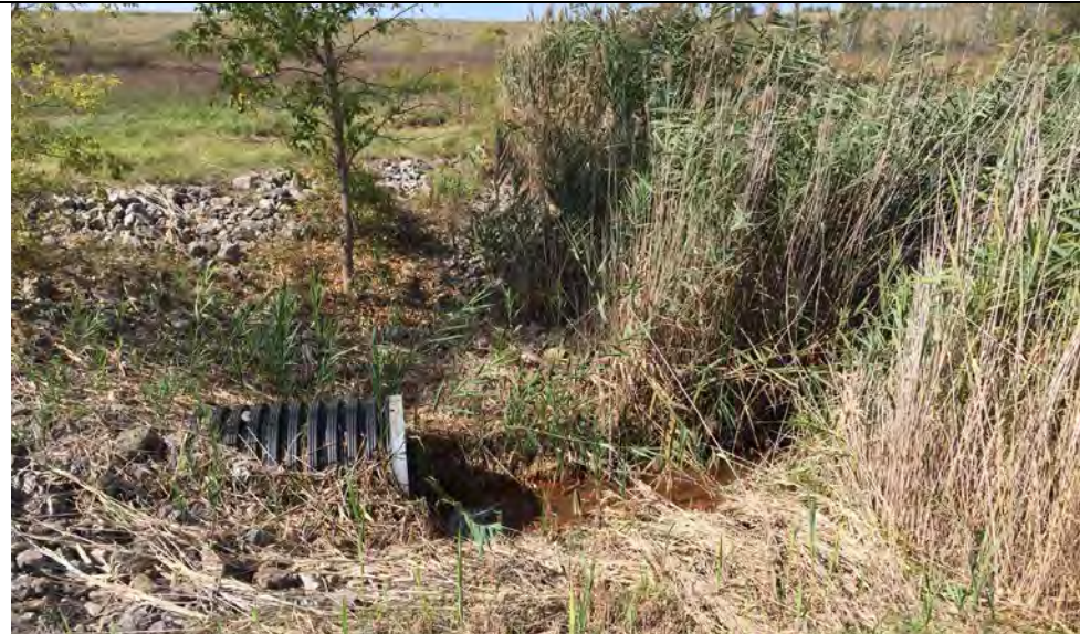
47. Perimeter Ditch Culvert Beneath Road Crossing Has Been Cleared of Vegetation Around Entrance.
