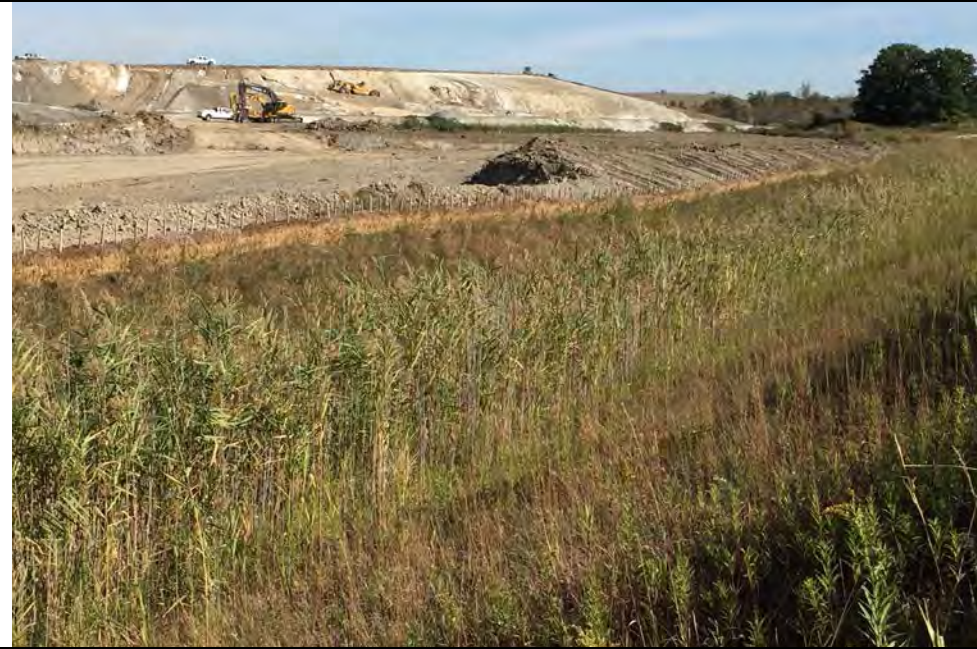
33. Internal Landfill Drainage Ditch on South Side and Capping on Top of Area F3.
