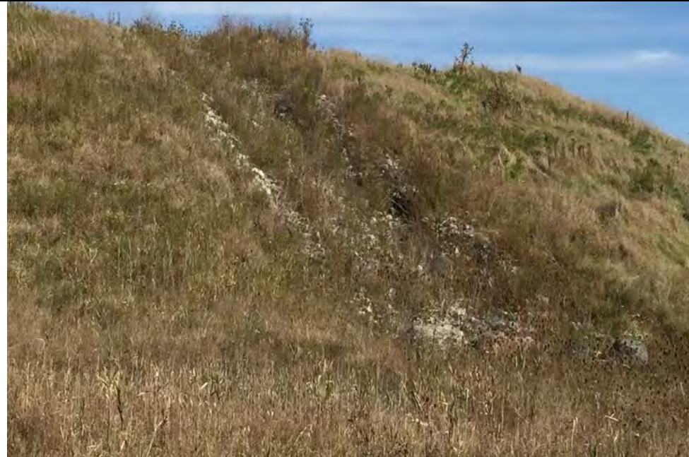
69. Close-up of Slope Downchute From Intersection of Closed Areas F1 and F2. Some Runoff Erosion in Riprapped Area. Same as Photo 67.
