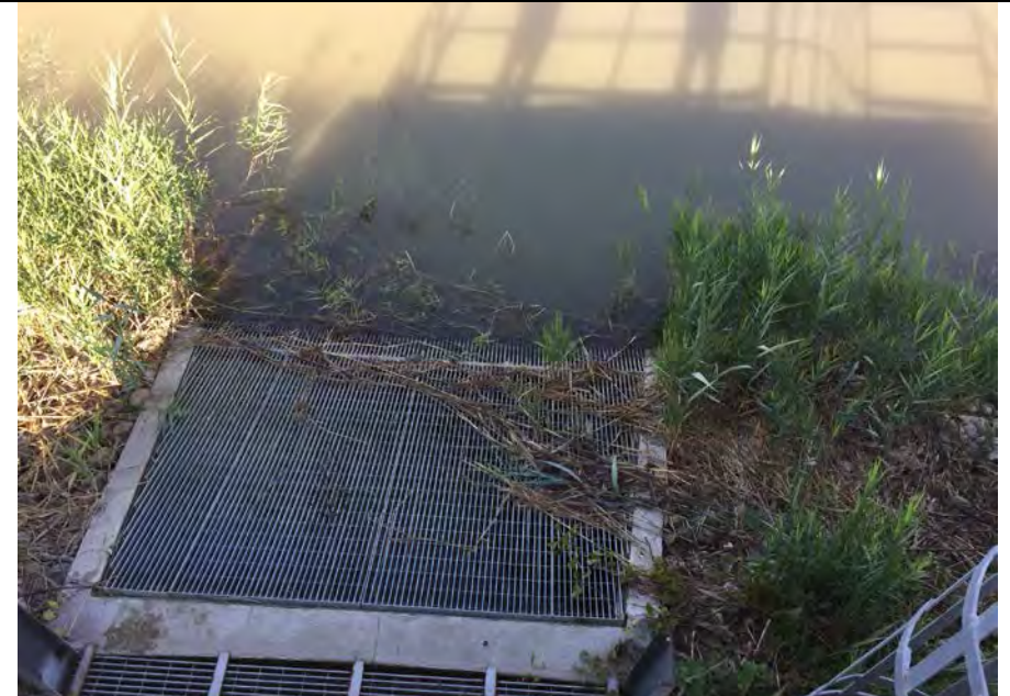
6. Basin Intake Screens. No Significant Blockage Noted. DTE Routinely Inspects and Cleans Grate Area.
