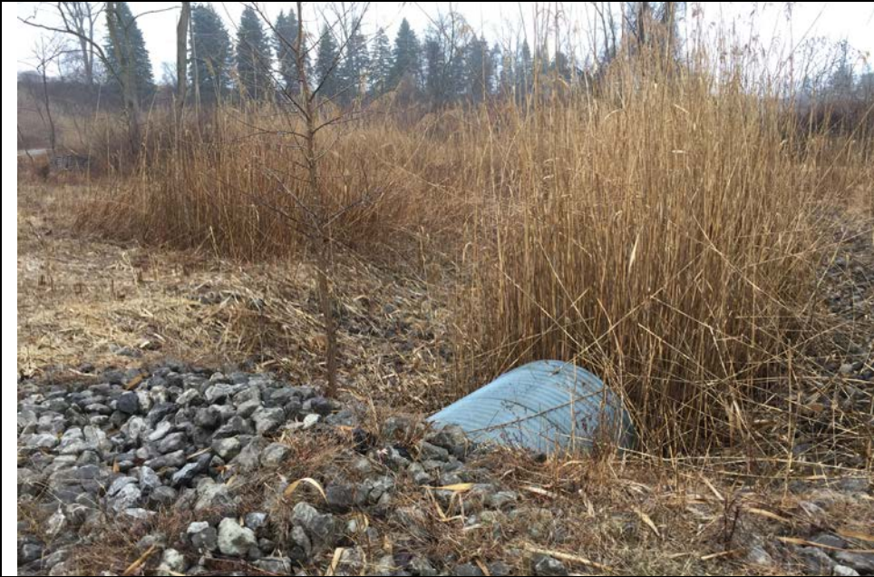
29. View of East Side Ditch Crossing Culvert with Heavy Vegetation at Flow Entrance. Road Crossing to Access Top of Landfill.
