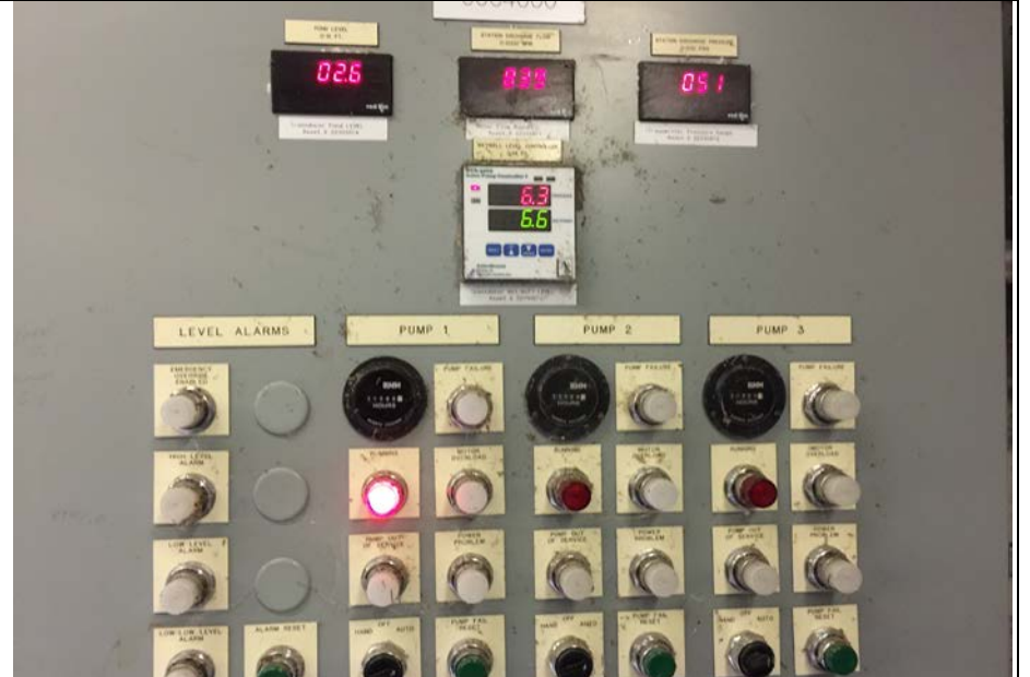
4. Pump Control Panel. Pump #1 Running. Pumps Cycle for Each Run Unless Higher Pond Level Needs More Pumps On.
