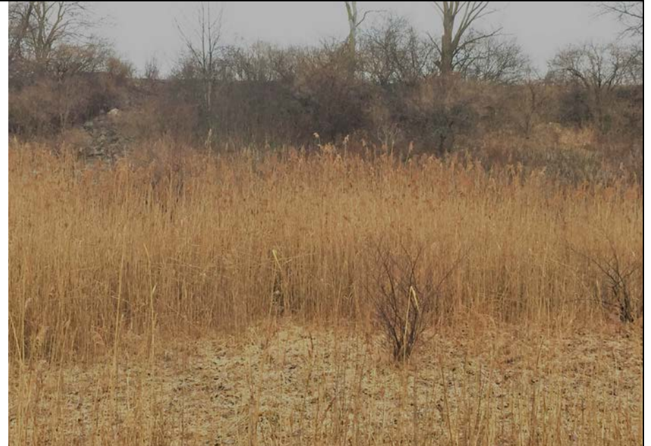
38. View of Closed Landfill Slope with Trees and Brush on Slope. A Riprap Downchute Visible. No Slope Erosion Noted During Close-up Inspection.
