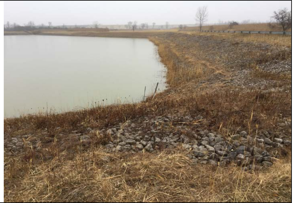
2. SWDB, North and East Sides. Slopes are Protected with Stone Within Water Level Range. No Visible Slope Erosion. Vegetation Cut on Slopes.
