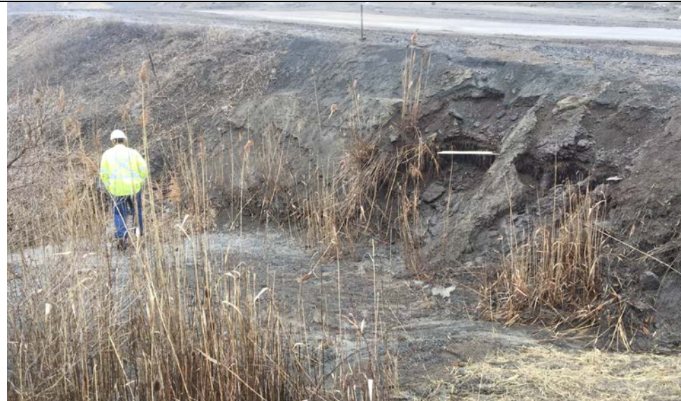
79. Discharge Location of Old Culvert Beneath Haul Road. Some Previous Road Slope Erosion.
