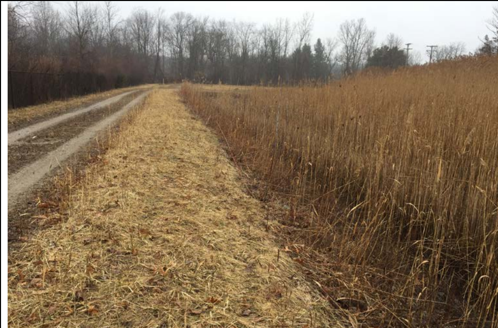
37. Looking East Along North Side of Perimeter Road and Ditch. Road and Slope in Good Condition.
