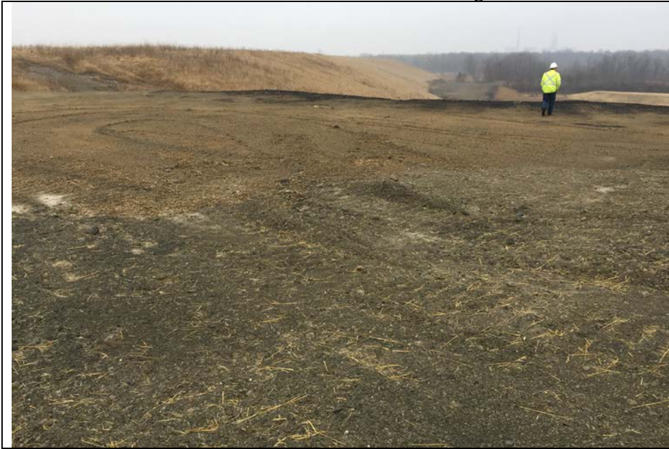
65. Portion of the North End of Areas F3 and/or D3 where Seeding and Final Grading May Not be Completed. No Visible Surface Erosion. Edge Berm Shown.
