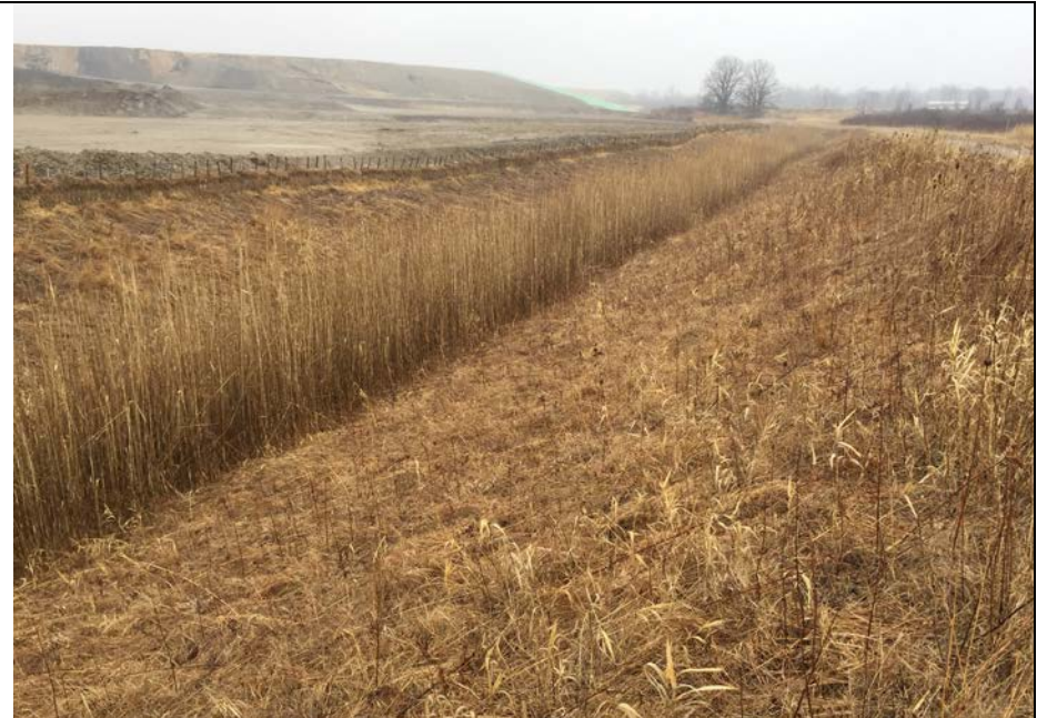
86. Looking NE at Perimeter Ditch and G2 Area. Ditch Slopes were Reconstructed in 2010, Appear Stable, and Well Vegetated.
