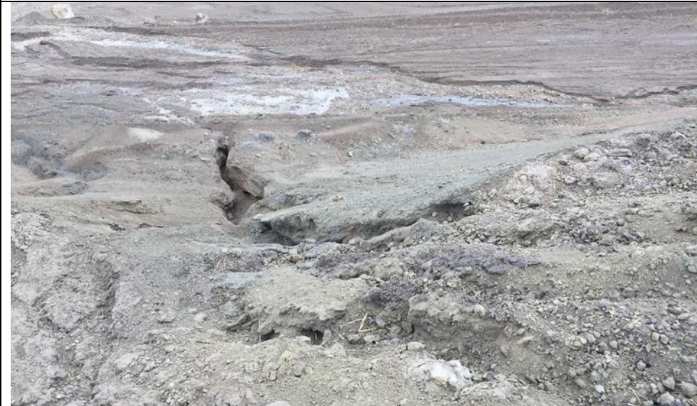
103. Top of Erosion Gully Shown in Photo 102. Runoff from Cover Surface Flow from Area F3. Haul Road Shown at Top of Photo with Gully Flow Across Road. Repair Needed
