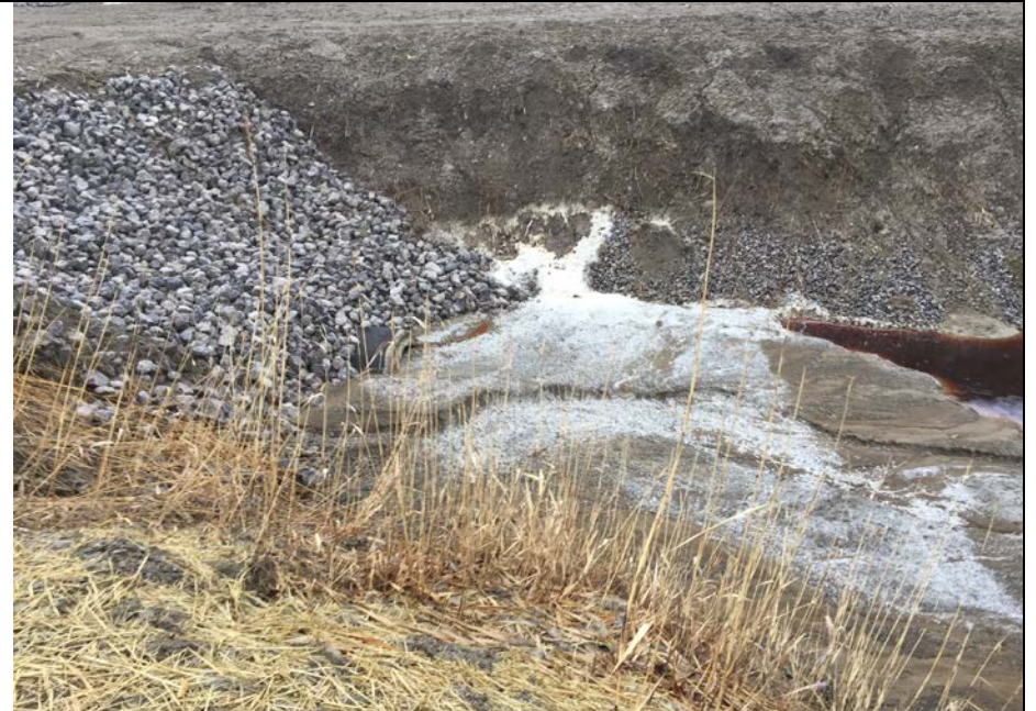
78. Previous Location of Old Culvert and Discharge from Pond in Photo 77. New Culvert Crossing Beneath Main Haul Road Installed Late 2017.
