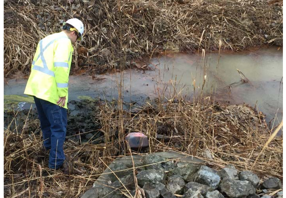
14. Looking at Trickle of Flow (09:08 AM) from Discharge from Pump in Building and Controls Shown in Photos 13 and 12, Respectively.
