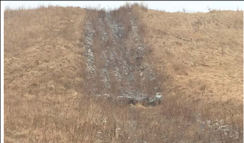
47. Major Riprapped Downchute Near West Corners of Closed Landfill Areas F1 and F2. Close Inspection Indicated Chute Stable & No Change Since 2015.
