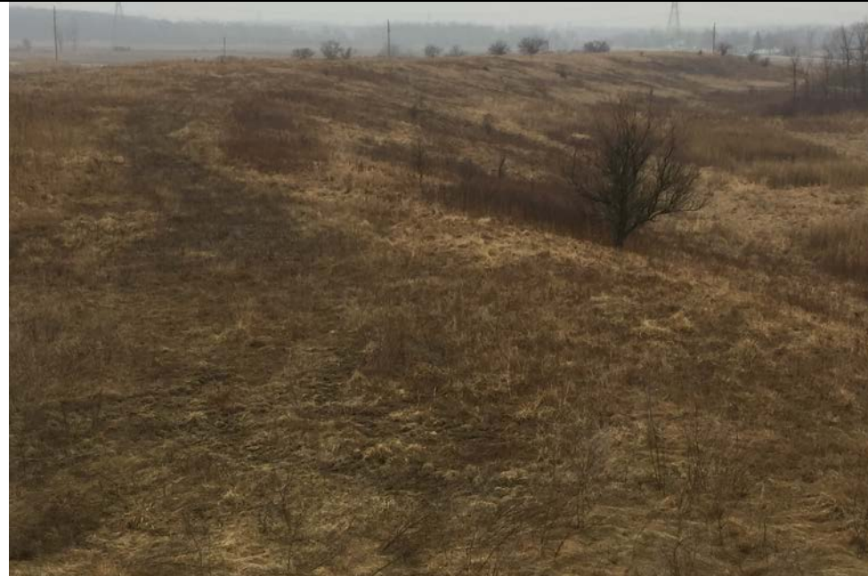
61. View of Outside Slope of Northeast Side of Landfill. Area downslope is Not a Closed, Active or Future Landfill Area. Minor Woody Vegetation on Slopes.
