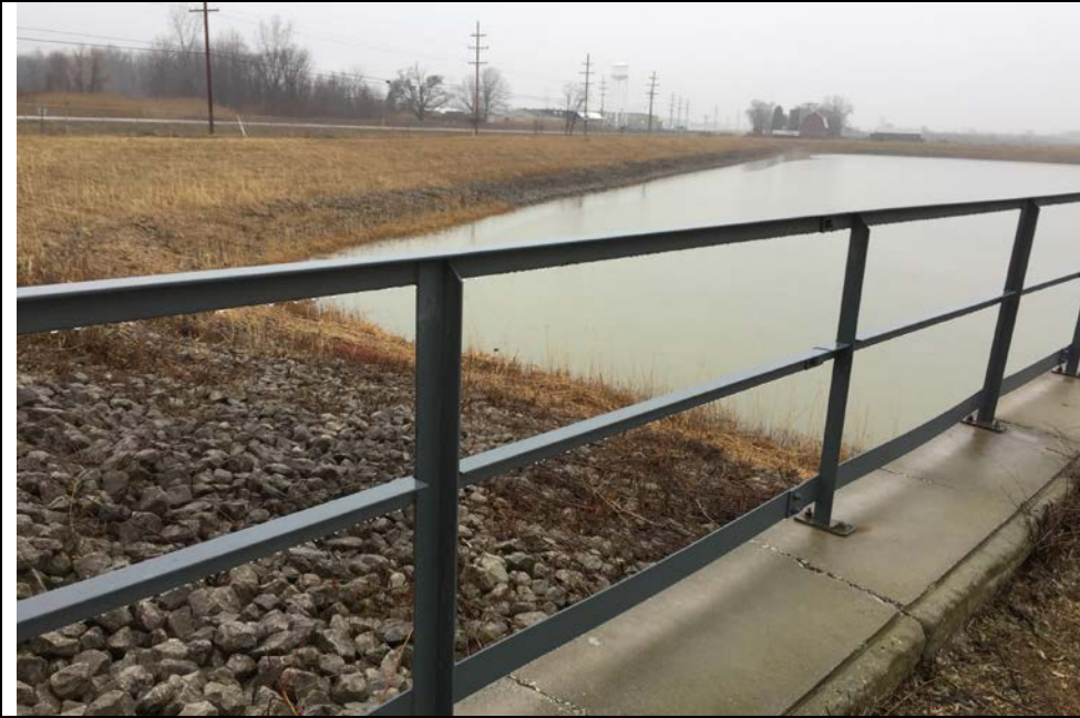
1. Storm Water Detention Basin (SWDB), South and West Sides. Slopes are Protected with Stone. No Visible Slope Erosion. Vegetation Cut on Slopes.
