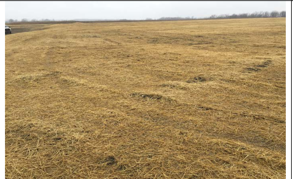
104. Final Cover Surface in Area F2. Drainage to F3 Corner that Drains to Fill Slope Shown in Photo 103.
