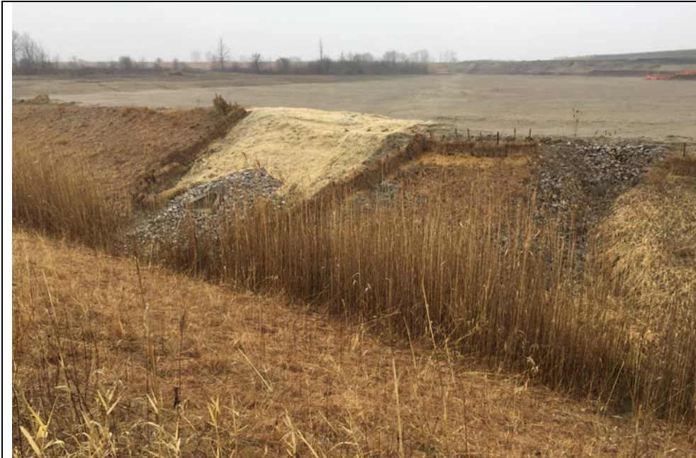
85. Perimeter Ditch Alongside G2 Area. Right Side Gully Filled with Riprap from Previous Repair. New Pipe Discharge Chute from G2 Surface Runoff Flow.
