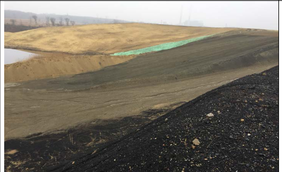
68. Internal Haul Road and Area F3 Interim Seeded Slope. Photo Right Side Match to Photo 67. Some Erosion Gully into Pond in Center of Photo 67.
