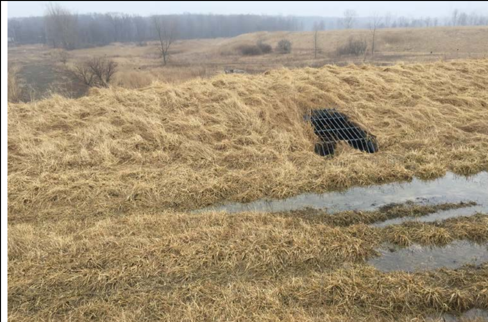
73. Collection Swale & Berm with Downslope Drainage Pipe with Steel Grate. No Blockage but Some Minor Wheel Ruts in Surface Area.
