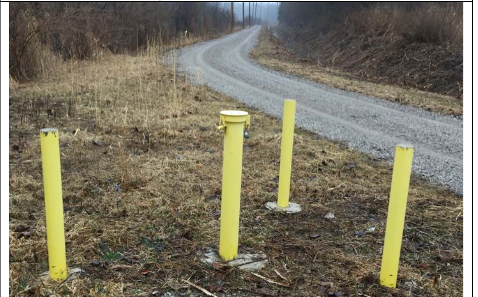
20. Close-up of Monitoring Well 16-04 and Perimeter Road Along Ditch. Ditch and Road Maintenance has been Performed. No Slurry Wall Markers.
