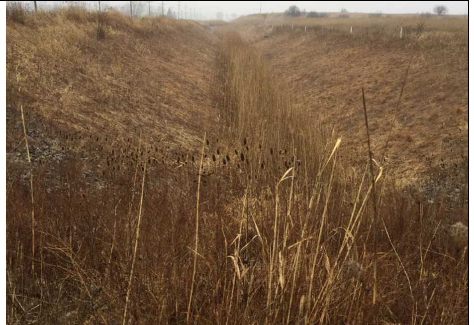
90. Looking West at Perimeter Ditch West of Gate Location. Slopes Stable and Well Vegetated. Ditch Slopes were Reconstructed in 2010.
