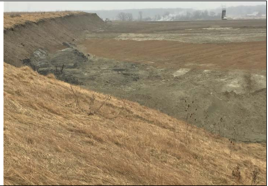
110. Looking SE at Active Area G2 Phase 1. Waste Placed at Bottom Slope, but Not Graded or Compacted Yet. Steep F1 Slope Cemented and Stable.
