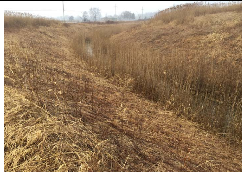
94. Landfill Perimeter Ditch at Southwest Corner of the Site. No Road Construction Alongside of Ditch. Slopes Stable and Well Vegetated.
