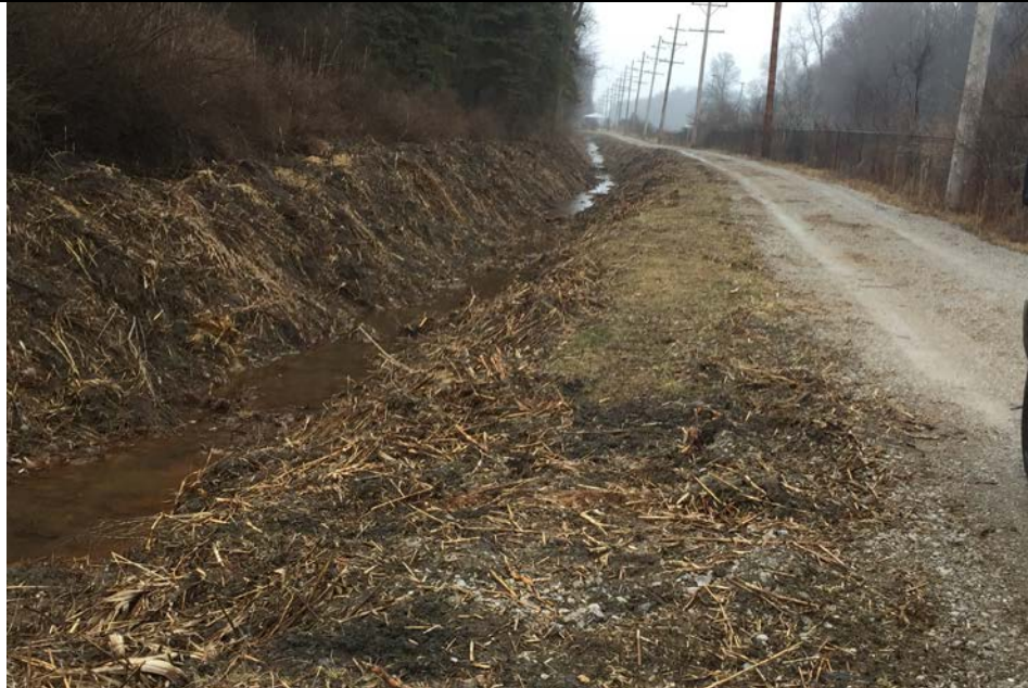
17. Looking at Recent Maintenance Along East Side Perimeter Ditch. Road Remains in Good Condition. No Slurry Wall Markers Shown. New Road.
