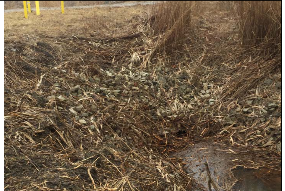
18. Clogged Culvert Entrance at Road Crossing Along East Side. DTE Indicated Removal of Vegetation will be Scheduled. MW 16-03 Shown.
