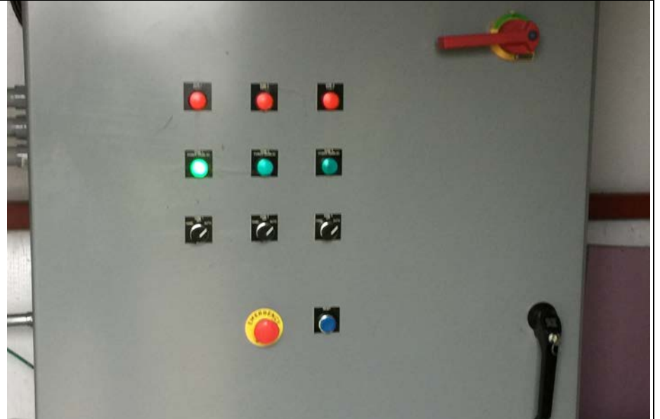
12. View of Control Panel in NE Off-Site GW Capture System Building. Zone 1 Pump Operating. All Run Switches in Auto Mode.
