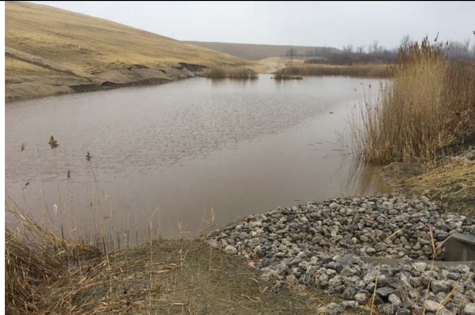
77. Pond Side of New Outlet Culvert with Riprap Check Dam. Culvert Discharge Side Shown in Photo 76.
