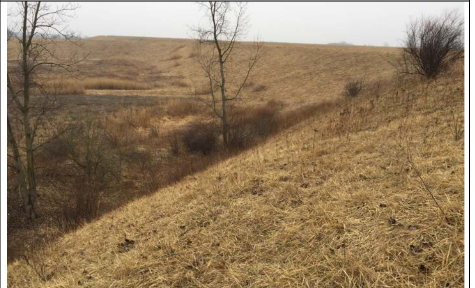
48. View of West Side Landfill Slopes of Closed Areas. Slopes Well Vegetated and Free of Any Significant Woody Vegetation.
