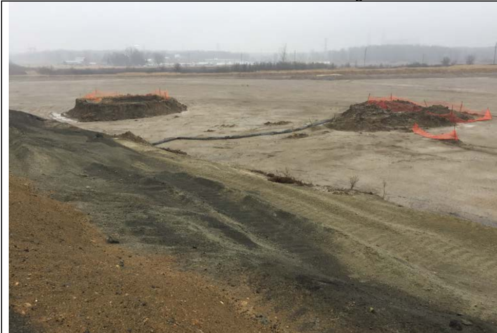
81. Active Area G2 Phase I where an Abandoned Gas or Oil Well was Located.
