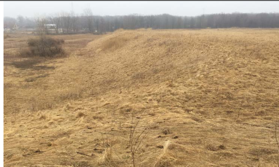
71. Looking South at Slope and Surface of Closed Area C. Slope and Surface Well Vegetated.
