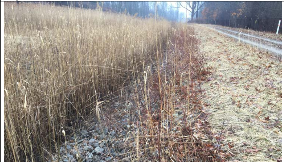
39. Perimeter Ditch Vegetation and Riprap Along Slope. Road in Good Condition. Slurry Trench Marker on Side of Road.
