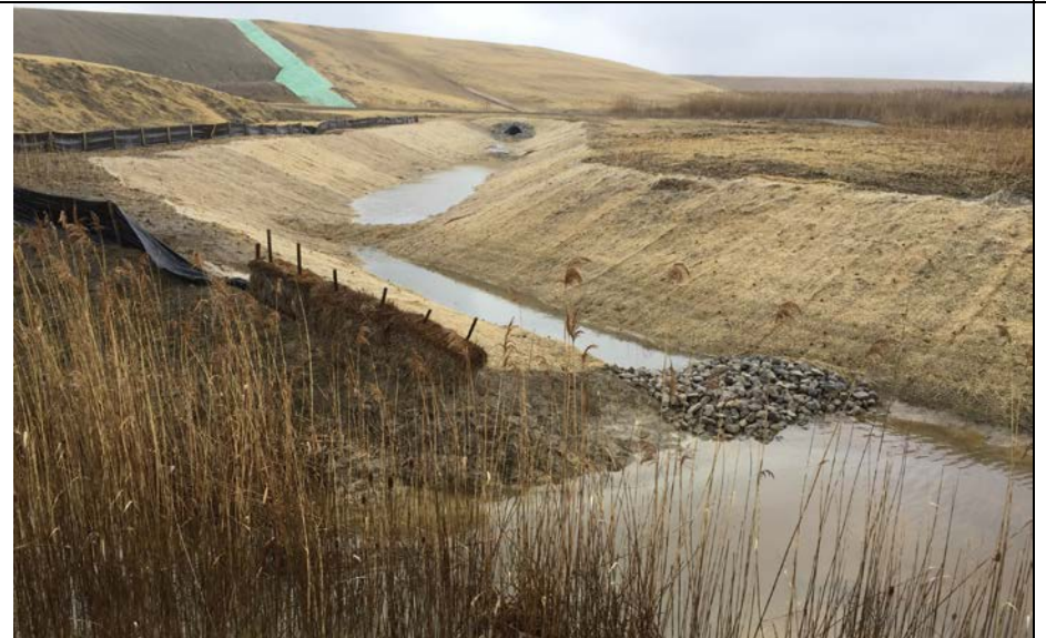
100. View of the New Internal Ditch from Point of Intersection with Perimeter Ditch. New Ditch Also Shown in Photo 76.
