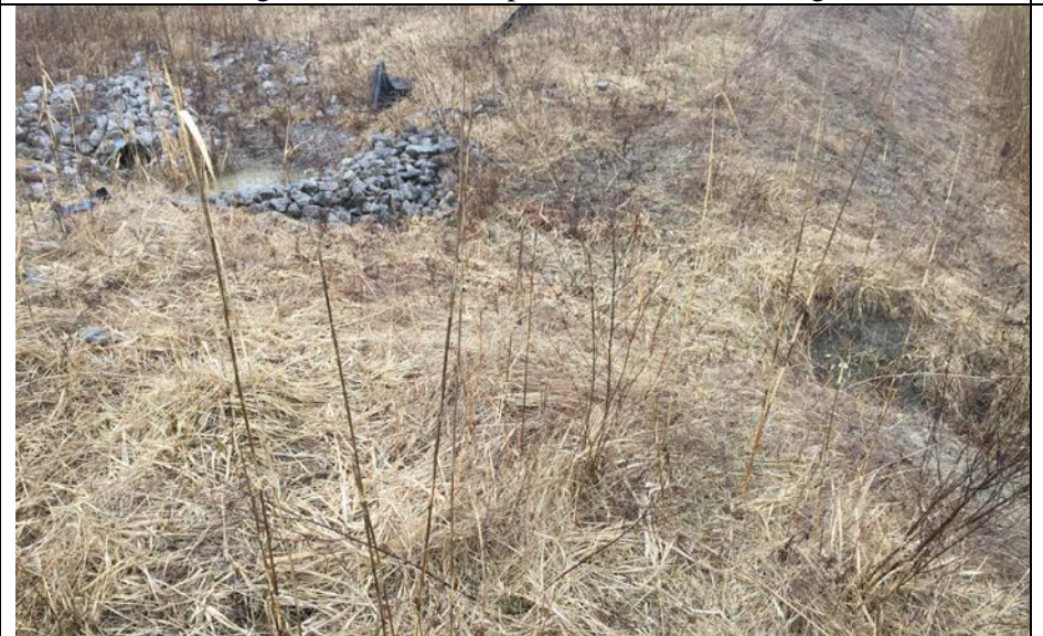
96. Culvert and Riprap Check Dam with Flow Draining into Perimeter Ditch. Some Slope Runon Erosion Noted Along Ditch.
