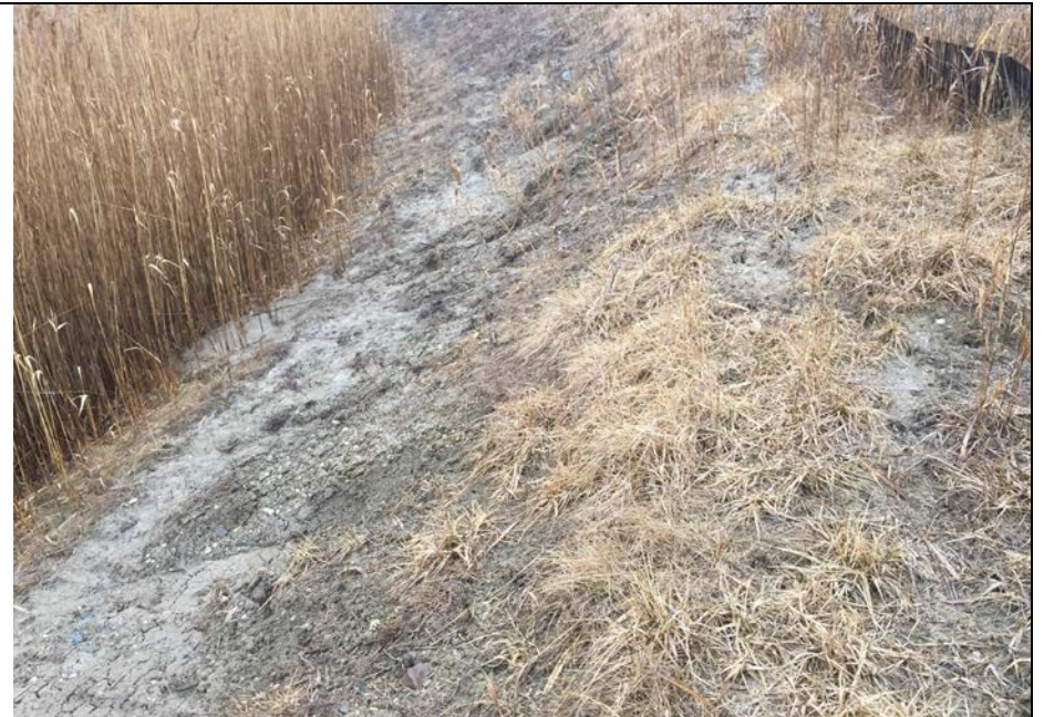
98. Portion of Ditch Near Gas Piping Fence Enclosure that has been Graded. Slope Appeared Stable but Vegetation is Sparse and May Regrow in Spring.
