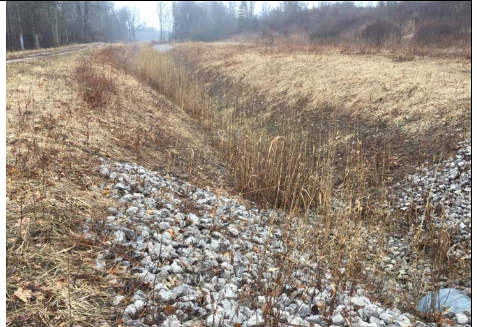
42. View of Perimeter Ditch with Little or No Water Flow. Slopes Appeared Stable and Culvert Not Blocked.
