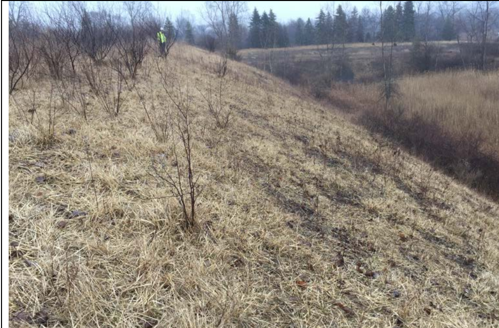
49. Looking at East Slope of Closed Area D1. Slope Appeared Stable, Some Small Woody Vegetation and Person Standing at Top of Ditch in Photo 50.
