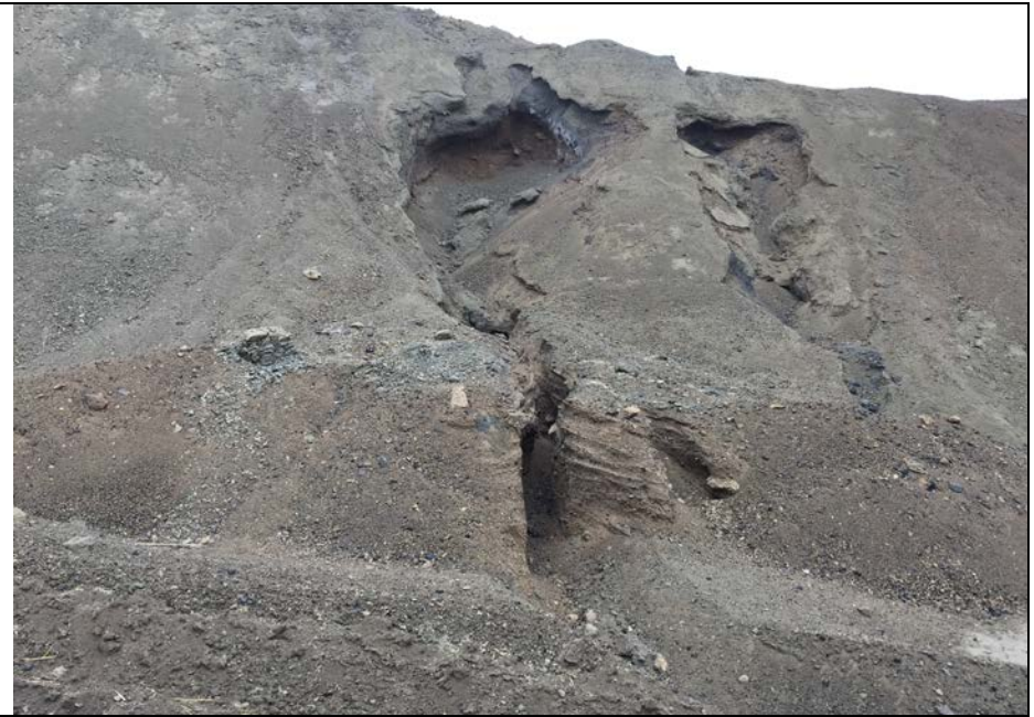
102. Significant Runoff Erosion Gully Present on Fill Slope Alongside Road to Top of Landfill at Area F3. DTE to Discuss Repair with Contractor.
