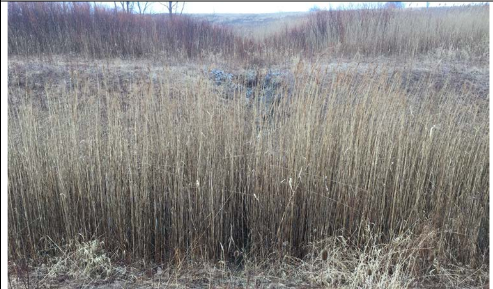
99. View of Erosion Gully Along Landfill Side of Perimeter Ditch at SW Corner Parallel to King Road. Additional Gully Repair Recommended.
