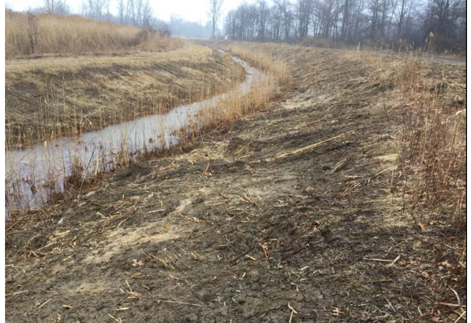
10. Looking at Perimeter Ditch Where Ditch Maintenance and Vegetation Removal Occurred Late Last Year (2017).
