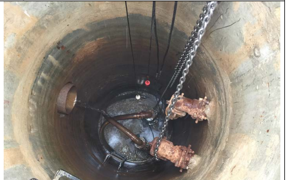
32. View of Sump, Pump Piping and Flow Pipe Entering Sump from Collection Ditch Shown in Photo 35.
