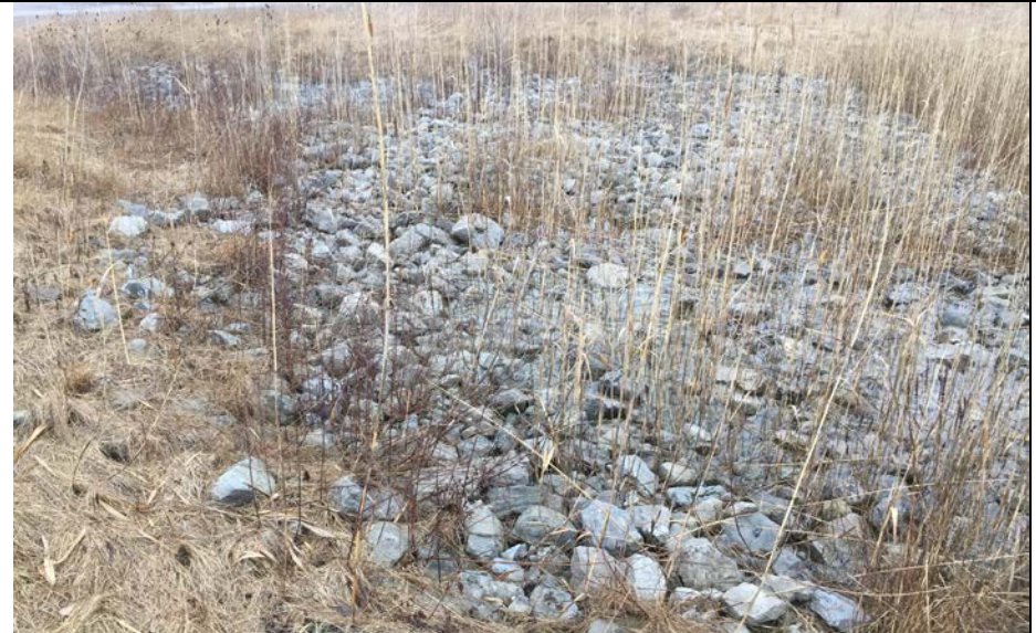
108. View of Riprapped Filled Swale at Top of Closed Area F2 as the Swale Approaches the Downchute Shown in Photo 110. Water in Middle.
