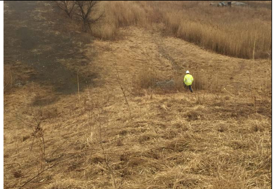
74. DTE Person Checking Outlet of Downslope Drainage Pipe. No Blockage and Acceptable Flow Conditions Reported.
