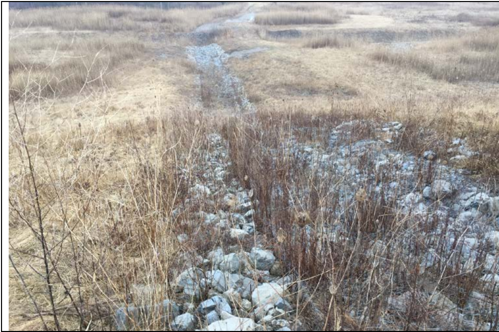
109. Area F2 Downchute Filled with Riprap and Screened Drains into Riprapped Perimeter Ditch. Road Crossing Right Side with Culvert. Slope & Chute Stable.
