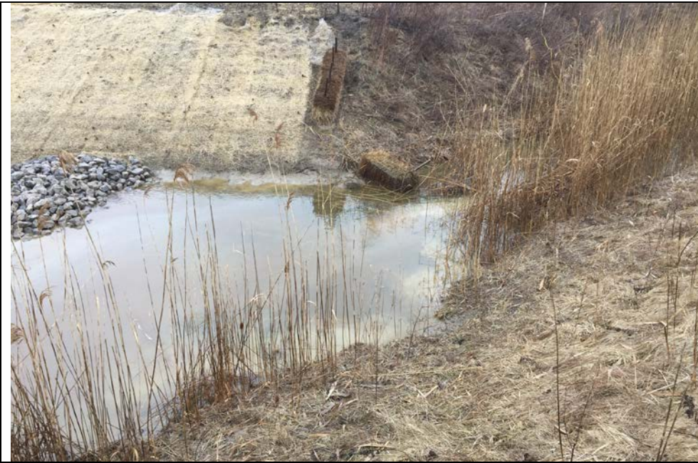
101. Pool of Water from Internal Drainage Pond. Future Slope Work Required.
