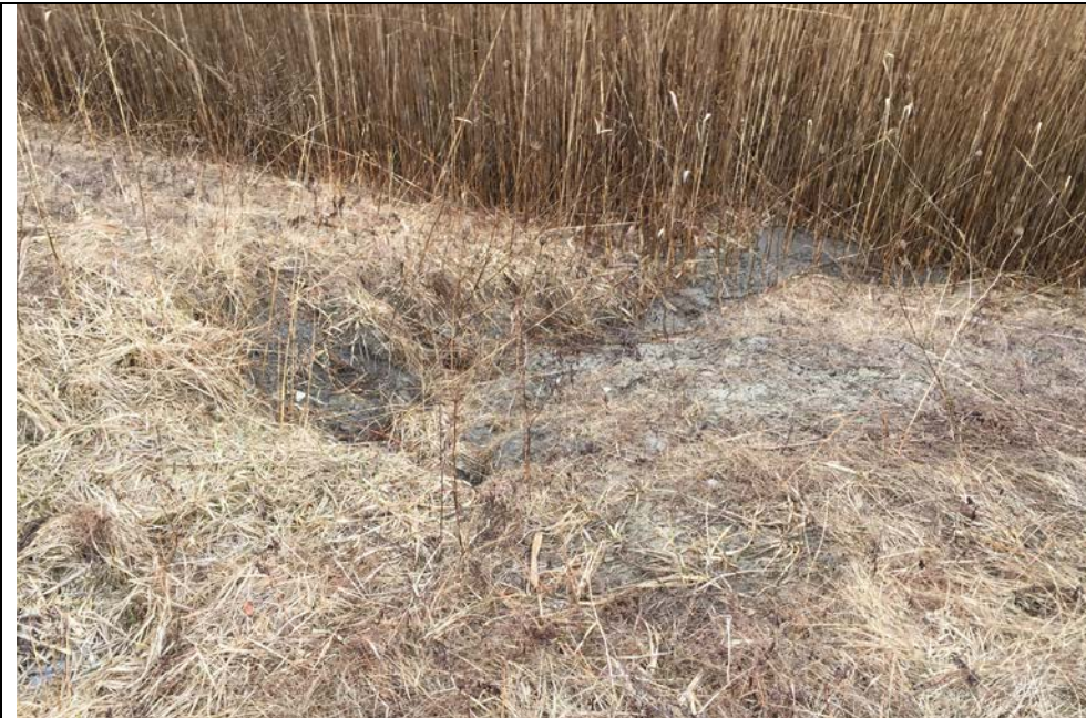
97. Photo of Ditch Bottom Slope Erosion Shown in Photo 96.
