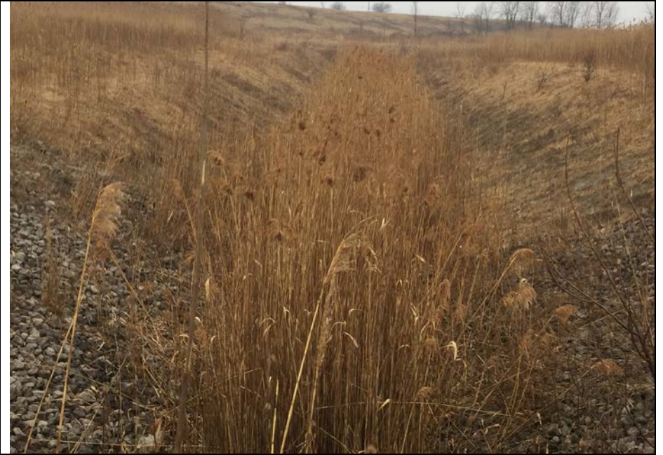
46. Looking South at Perimeter Ditch. Far Slopes at Top of Photo is Un developed Portion of Landfill. Ditch Slopes were Stable and Erosion Free.
