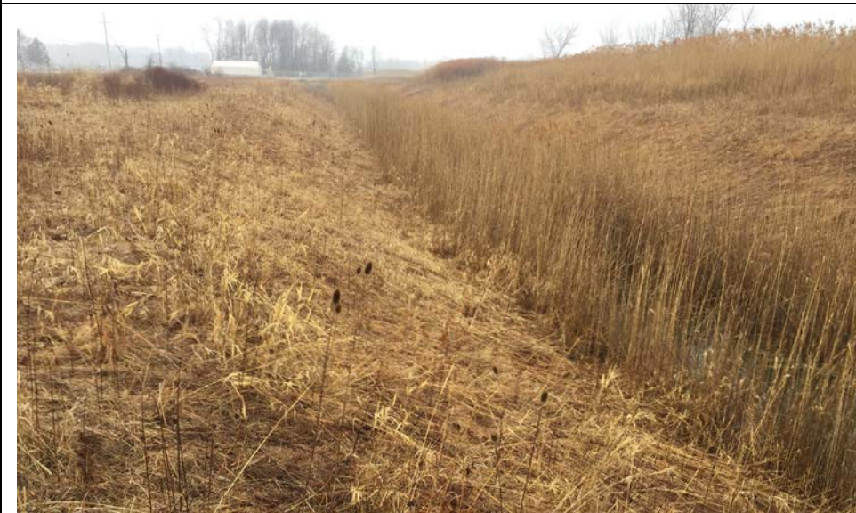
95. Looking North Along Portion of Perimeter Ditch Parallel to King Road and Reconstructed in 2010. Couple of Slope Erosion Gullies at Far End Photographed.
