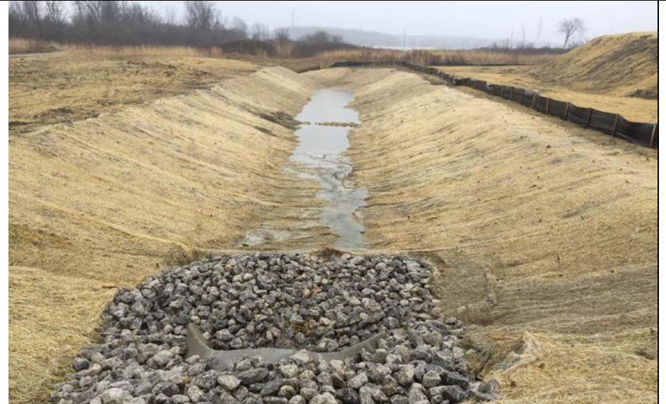
76. New Internal Drainage Ditch, Culvert and Riprap Check Dam Draining Flow from Internal Ponds. Ditch Connects with Landfill Perimeter Ditch.
