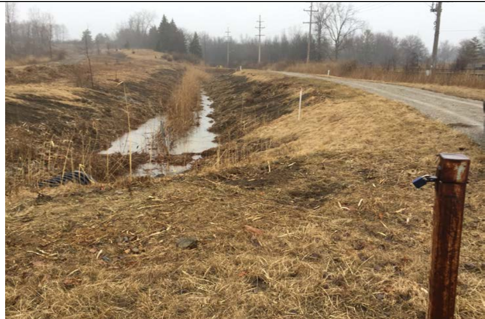
15. Perimeter Ditch Along NE Side of Landfill. Vegetation Maintenance. Piez. PZ-2 Shown. Ditch Culvert Entrance Open. No Slurry Wall Markers Present.
