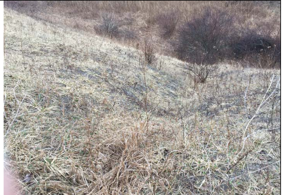
50. Close-up of Drainage Ditch Cut to Drain Landfill Surface Water. Ditch Appeared Stable and Well Vegetated.
