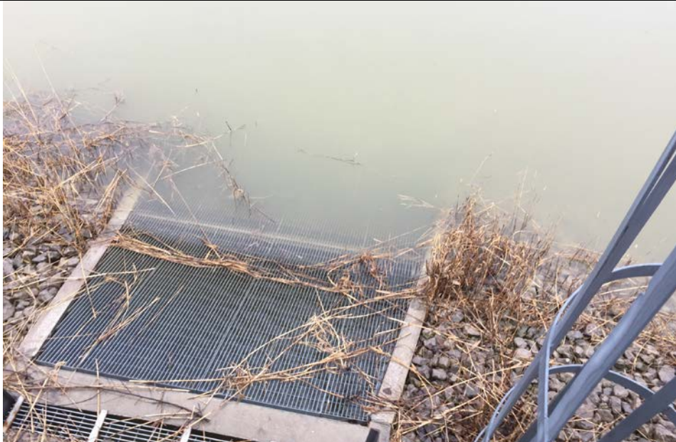
3. Intake Screens at SWDB. Water from Basin is Pumped Back to Power Plant Using One or More of 3 Pumps. DTE Inspects Daily and Records Pump Flow.
