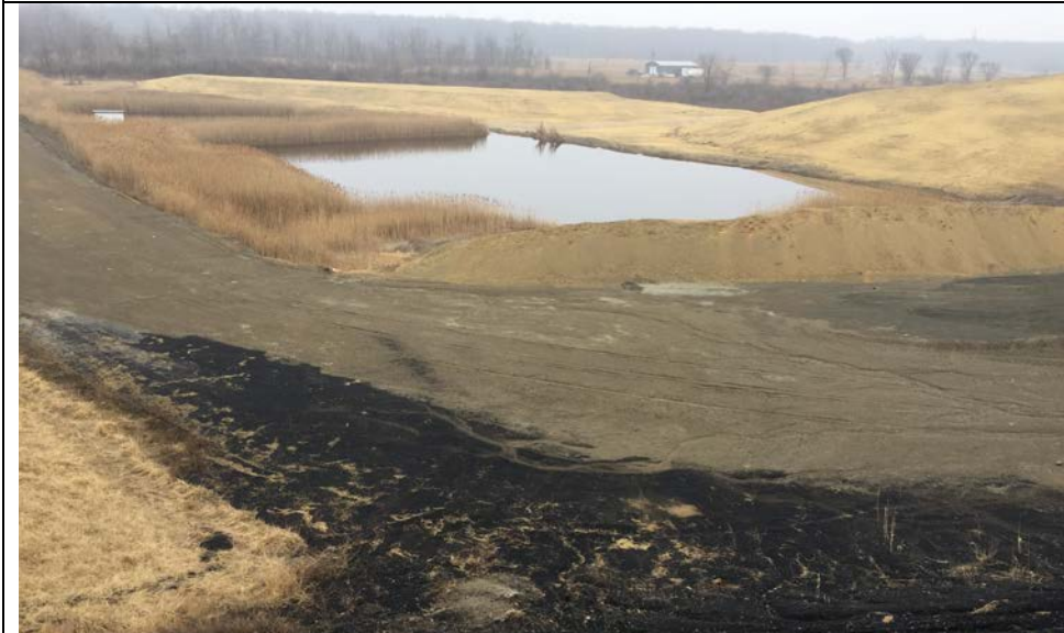
67. Looking East at Internal Stormwater Pond and Seeded Fill Stockpile (Top Left) and Area F3 Interim Seeded Slope (Top Right). No Significant Erosion Along Road.
