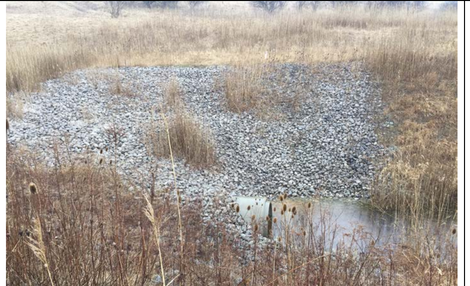
92. End of Concrete Pipe Installed as Ditch Replacement where Ditch Could Not Have Slopes Flattened Due to Adjacent Steep Slope. Flow Noted.
