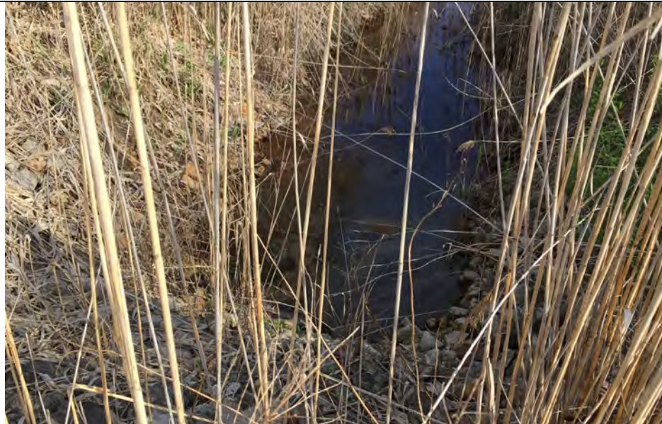
11. Looking at Perimeter Ditch Upstream of Culvert Under Site Road. Condition Typical of Unobstructed Flow into Culverts Along Perimeter Ditch Alignment.
