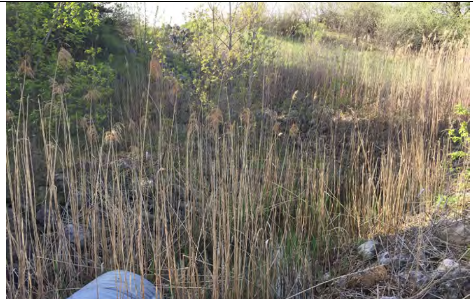
20. Culvert and Riprap Downslope Where Ditch Clearing of Vegetation Had Not Recently Occurred. Flow did not Appear to be Blocked.
