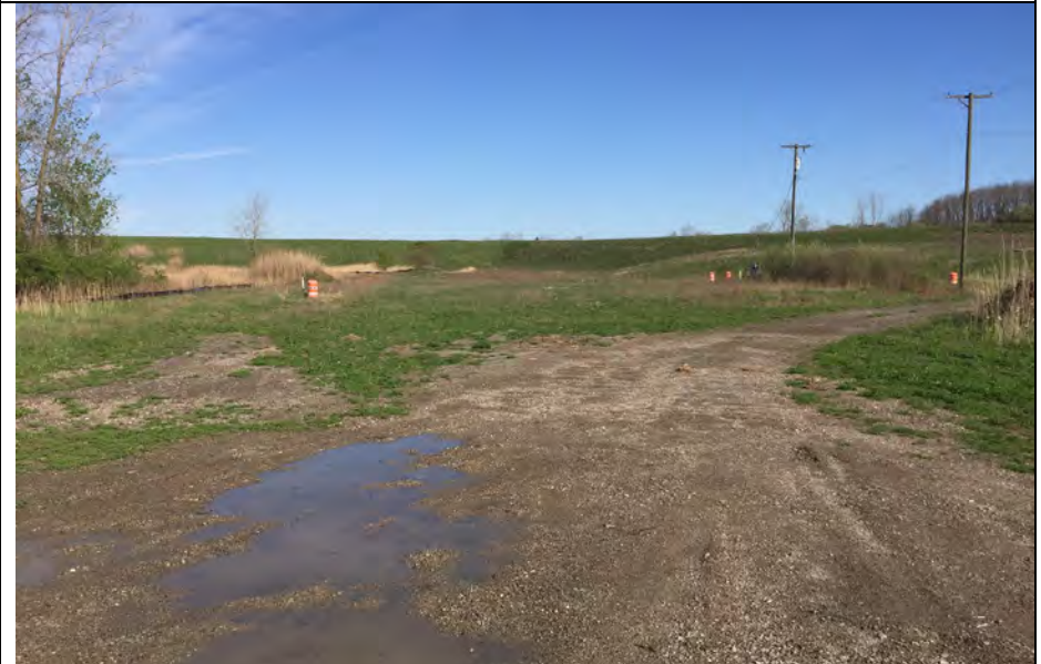
12. Looking at Barrels Locating and Protecting White Markers for Underground Electric Utility.
