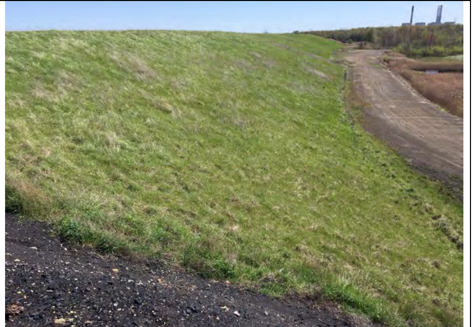
38. Embankment Slope Well Vegetated and Maintained. Area D2 Slope Looking East from Portion of Active Area D3.
