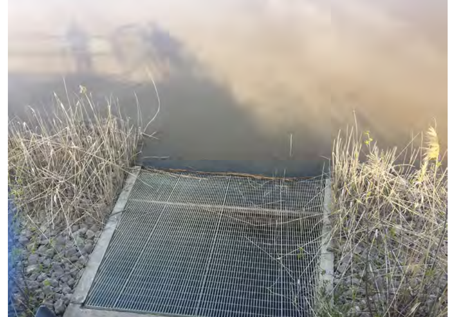
2. Intake Screens at SWDB. Water from Basin is Pumped Back to Power Plant Using One or More of 3 Pumps. DTE Inspects Daily and Records.
