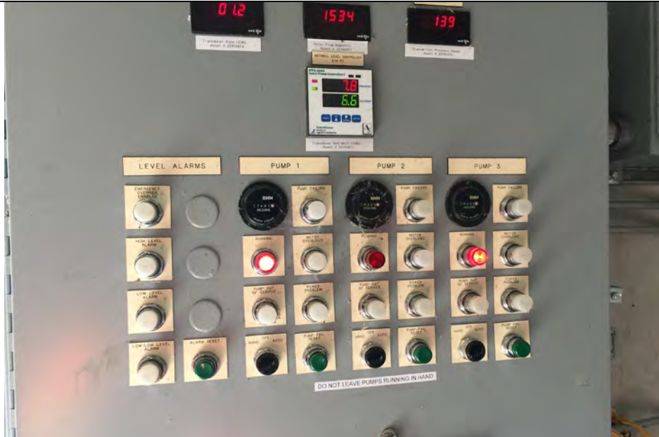
3. Pump Control Panel. Pump #3 Running. Pumps 1 & 2 Identified as Out of Service. Wall Flow Meter (Not Shown) was Operating. Pumps were Observed.
