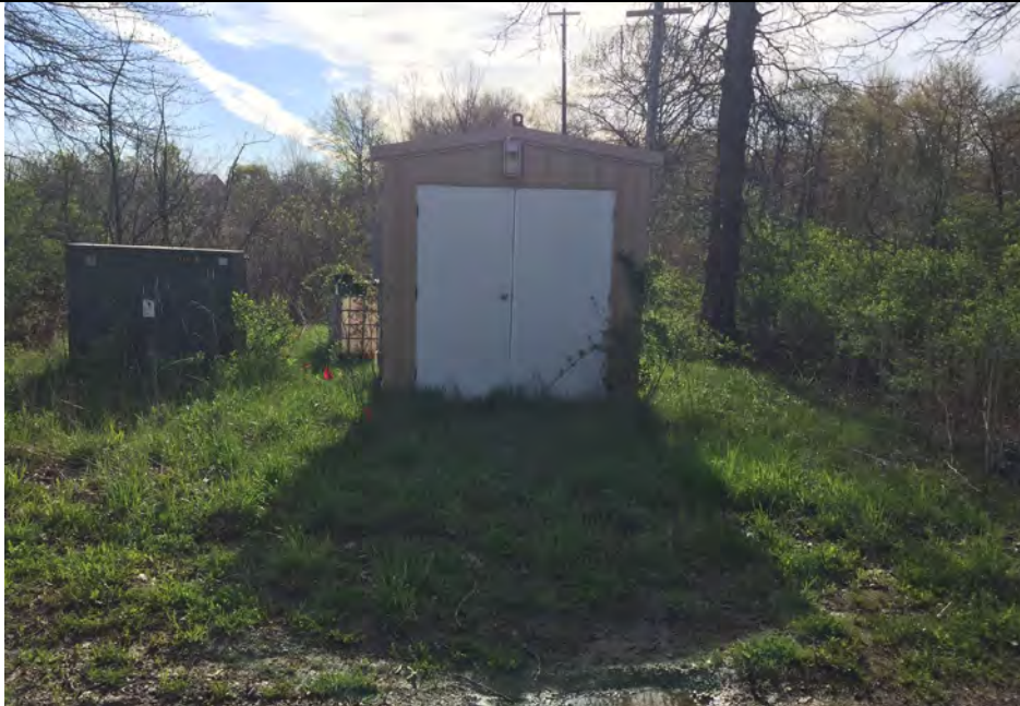
9. View of Locked Control Panel Building for East Side Groundwater Offsite Collection System. Panel Not Observed. Pipe Flow to Ditch Observed.
