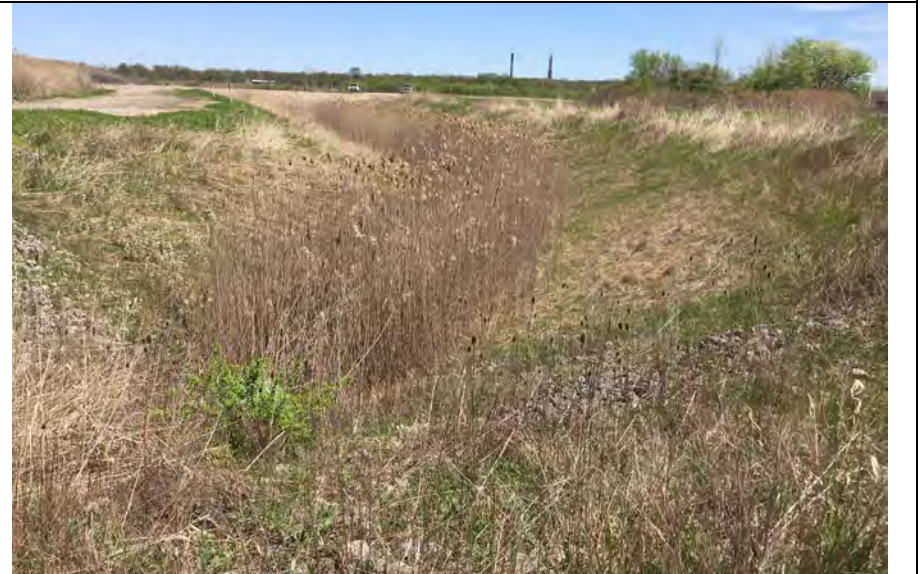
48. Looking at South Side Perimeter Ditch Where it Bends to the NE. Some Vegetation Present in Bottom but No Blockage Noted.
