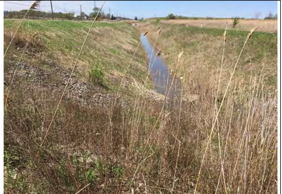
46. South Side Perimeter Ditch Looking West. Small Riprap Place at Road Crossings and Around Drainage Pipe Inlets and Outlets to Prevent Blockage.
