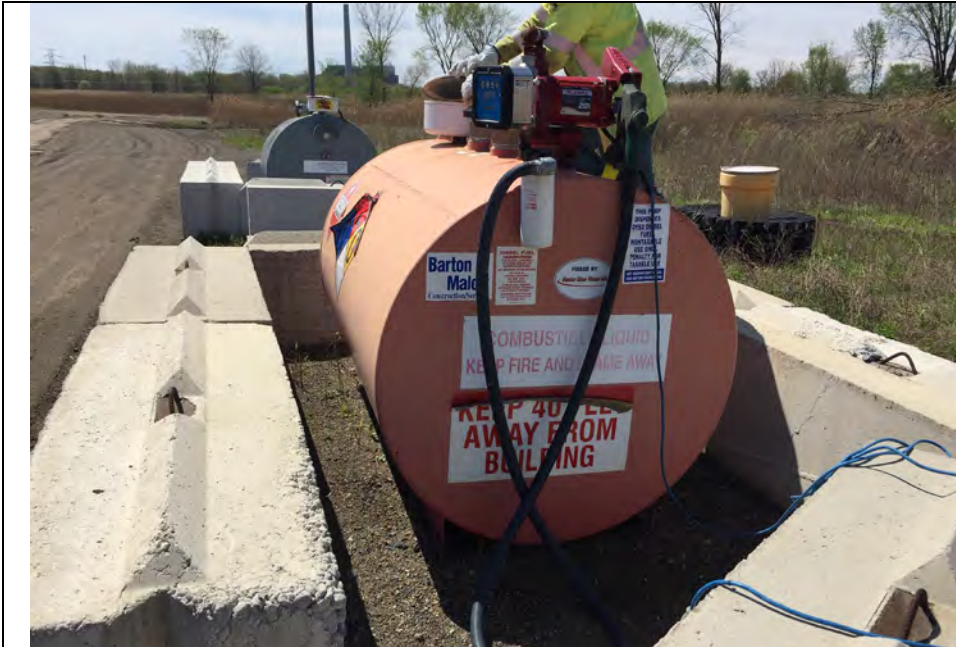
41 Second Fuel Tank that had Possible Dispensing Leak Repaired in 2019 after Inspection. Both Tanks Viewed in this Inspection and No Visible Leaks Noted.
