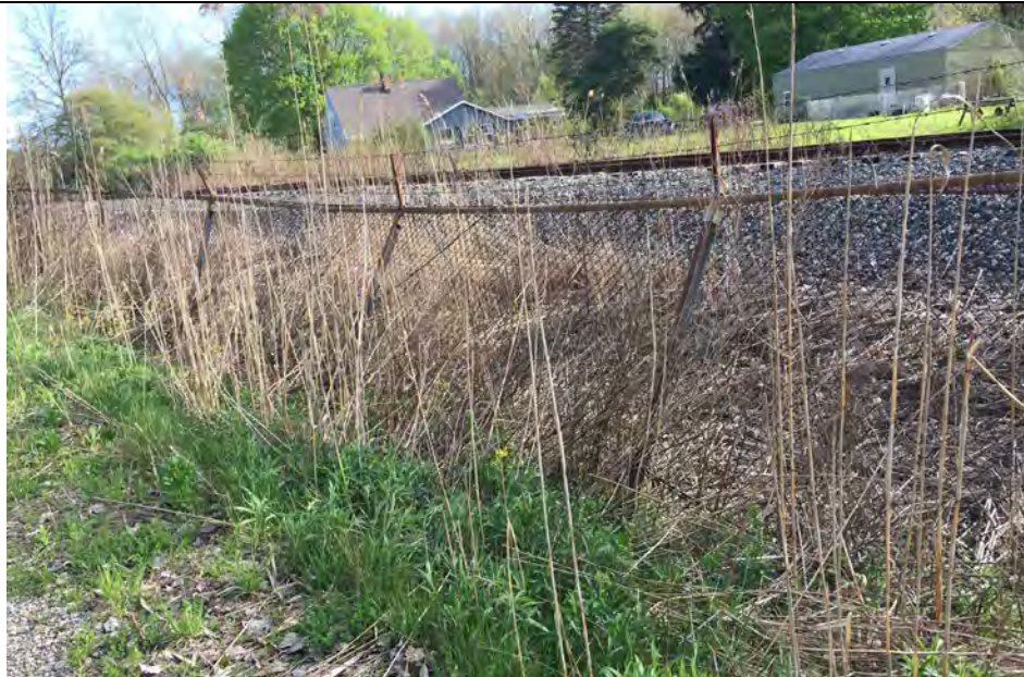
15. Perimeter Fence Leaning. However, Posts Appeared Solid when Attempted to Move.
