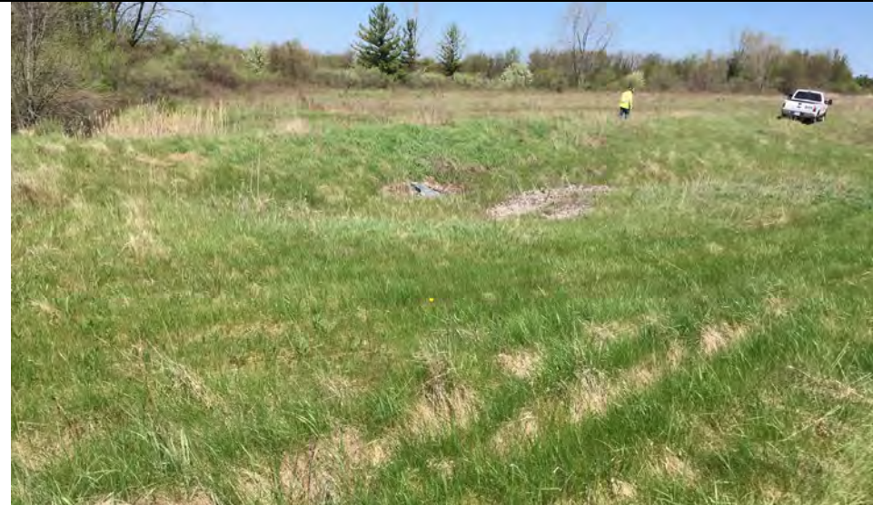
39. View of Top of Cover where Cover Drainage Swale Terminates at Exit Culvert Draining Flow to Outside of Landfill Cover.
