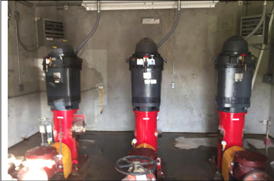
5. The 3 SDB Pumps. Pump No. 3 (Middle) was Verified as Running per Run Light.
