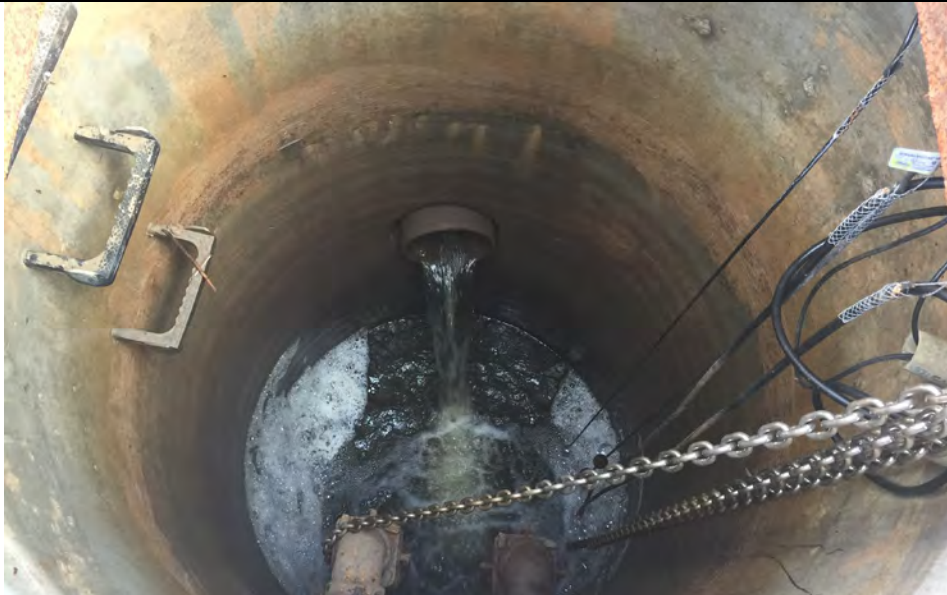
23. Sump Where 2 New Pumps Installed 2018. Pump Operation Verified by DTE Inspector. Panel Lights Operation to be Rechecked by DTE.
