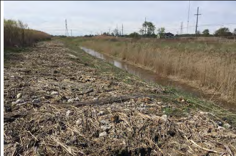
25. Another View of West Side Perimeter Ditch Where Recent Vegetation Removal Has Occurred.
