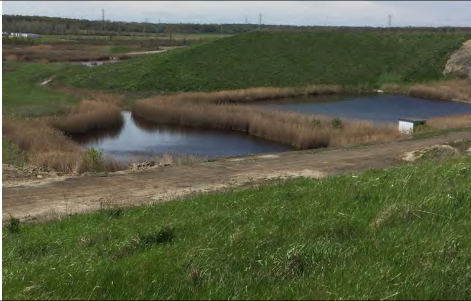
35. Runoff collection pond within landfill limits. Landfill area slopes appeared stable and well vegetated.
