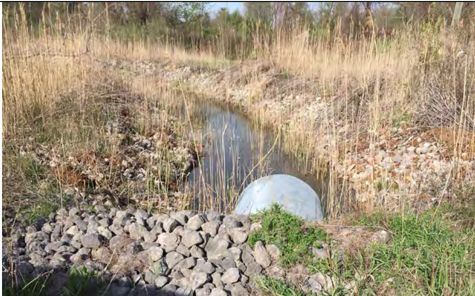
19. Another View of Portion of Perimeter Ditch Cleared of Vegetation During Routine Maintenance Activity.
