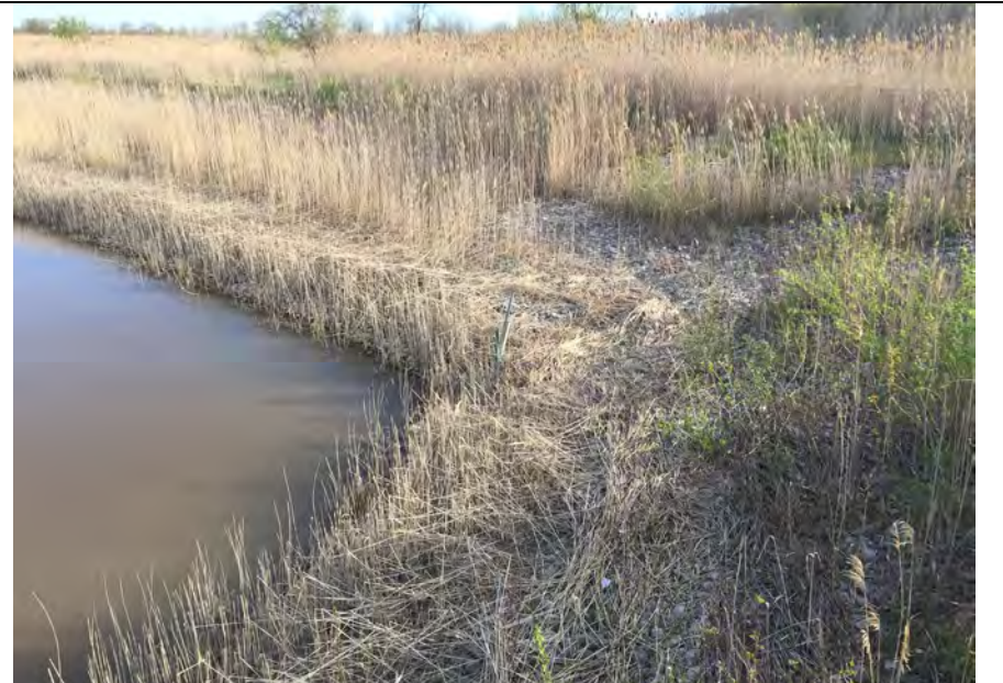
4. Looking at North East Corner of SWDB. Slope Protected from Erosion with Stone. Staff Gauge SG-13 in Middle of Photo Just Above the Water.
