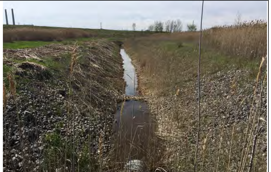
24. Perimeter Ditch West Side of Landfill Opposite Area B Looking South. Small Stone Check Dam Shown. No Visible Blockage or Flow.
