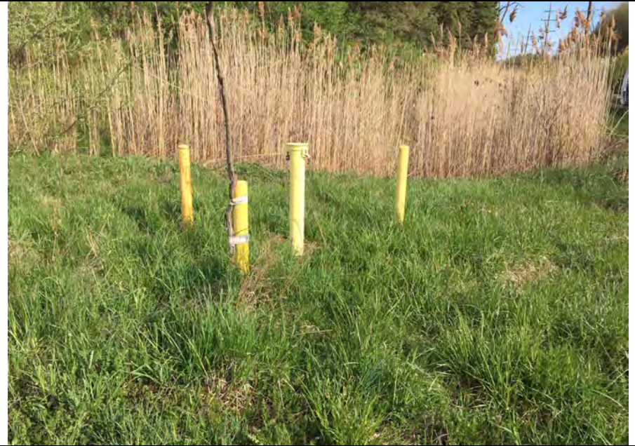
6. Monitoring Well 16-03. Well Protected and Cap Locked. Well Protection and Capping Typical of Inspected Above Ground Monitoring Wells.
