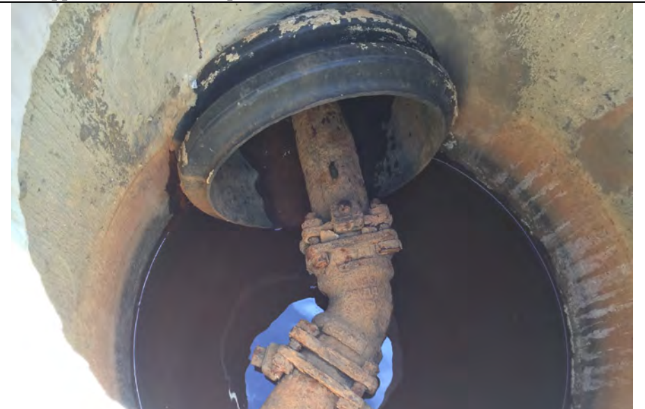
32. Inspection Sump and Piping from Pumps Shown in Photo 23. Inspected by DTE to Confirm Pump Operations and Flow (Flow Sound Within Pipe).
