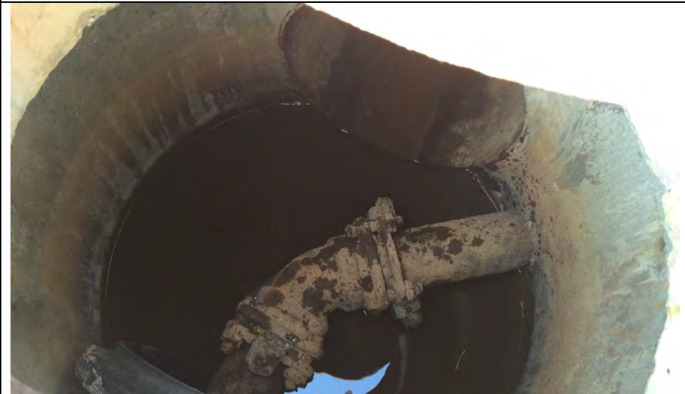
23. Manhole Containing Discharge Piping from Sump Pumps at Location Shown in Photo 24. Discharge will be to Culvert Connected to Ditch.
