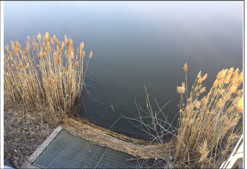
2. Intake Screens at SDB with Some Vegetation at Bottom. Water from Basin is Pumped Back to Power Plant Using One or More of 3 Pumps.
