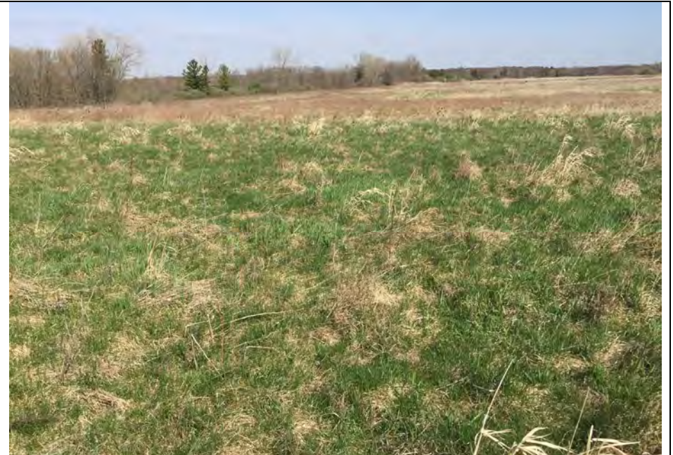
50. Another View of Typical Top of Landfill in Closed Areas. Area B.
