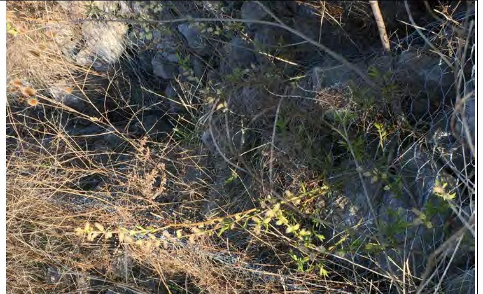
28. Photo Showing Large Void Between Riprap that can be Filled with Smaller Size Stone. Alternative Maintenance Methods are Possible.
