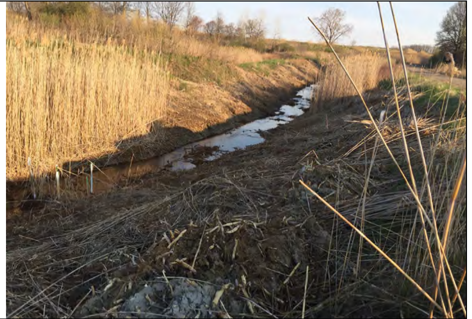
6. Again Ditch Maintenance Along One Side or the Other. Flow Maintained. Staff Gauge SG-7 Shown.
