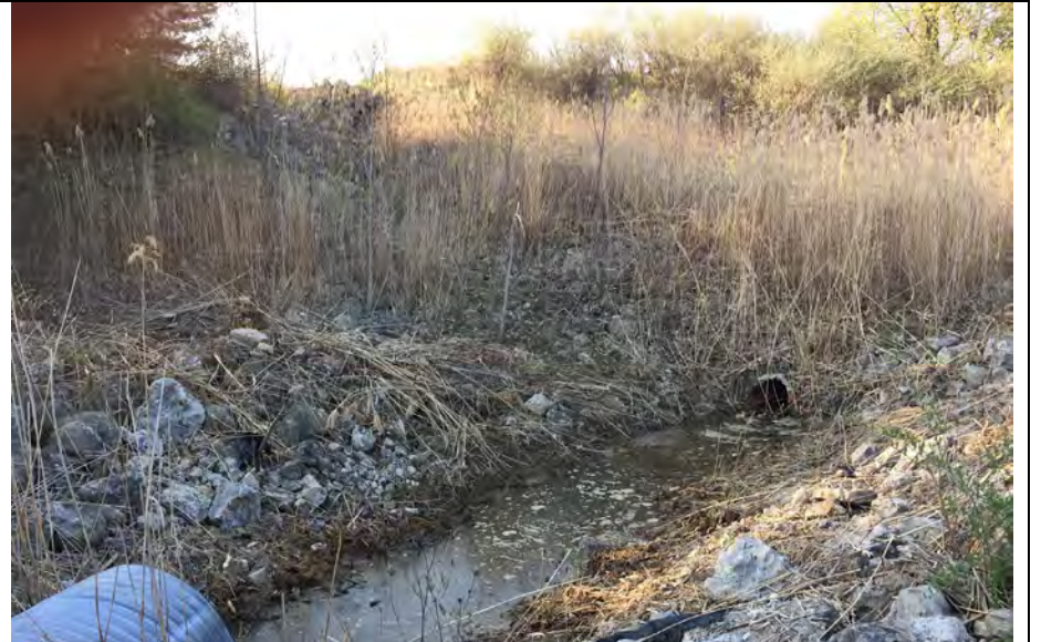
20. Culvert and Riprap Downslope Where Ditch Clearing of Vegetation Had Not Recently Occurred. Flow did not Appear to be Blocked.
