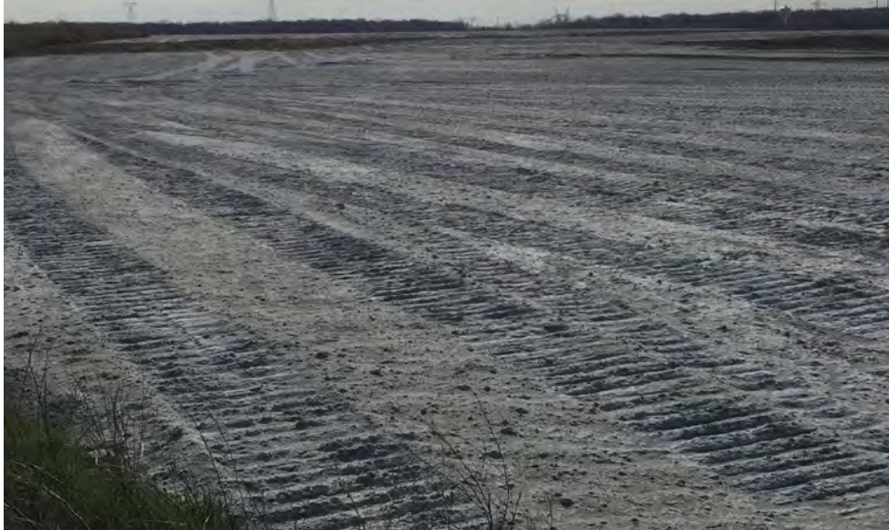
31. View of Top of Area G2 that has been Graded and Nearing Ready to be Capped in accordance with Landfill Cover Design. CCR Partially Cemented.
