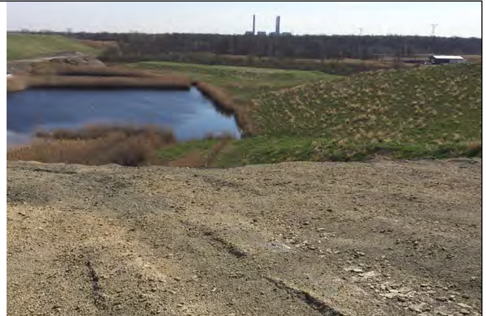
46. Another View of Runoff Collection Pond and Landfill Slope South of Pond. Slope Appeared Well Vegetated and Stable.
