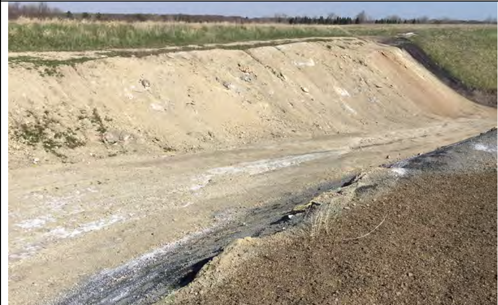
47. View of Active Haul Road to Top of Landfill Near Area F3D3. Slope Shown Part of Active Area F3. Minor Rutting in Road Surface.
