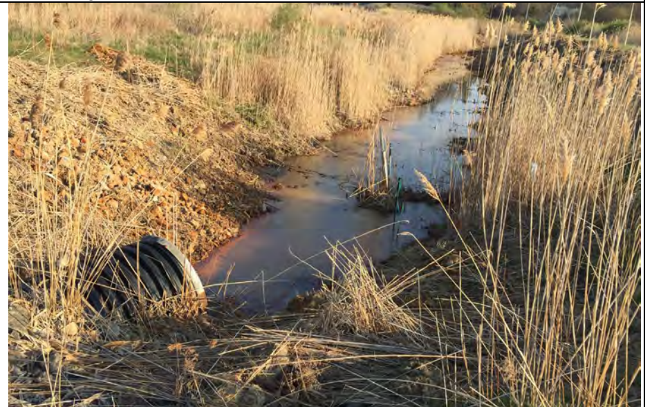
8. Perimeter Ditch Culvert and Staff Gauge SG-5. Culvert Entrance Open for Flow.
