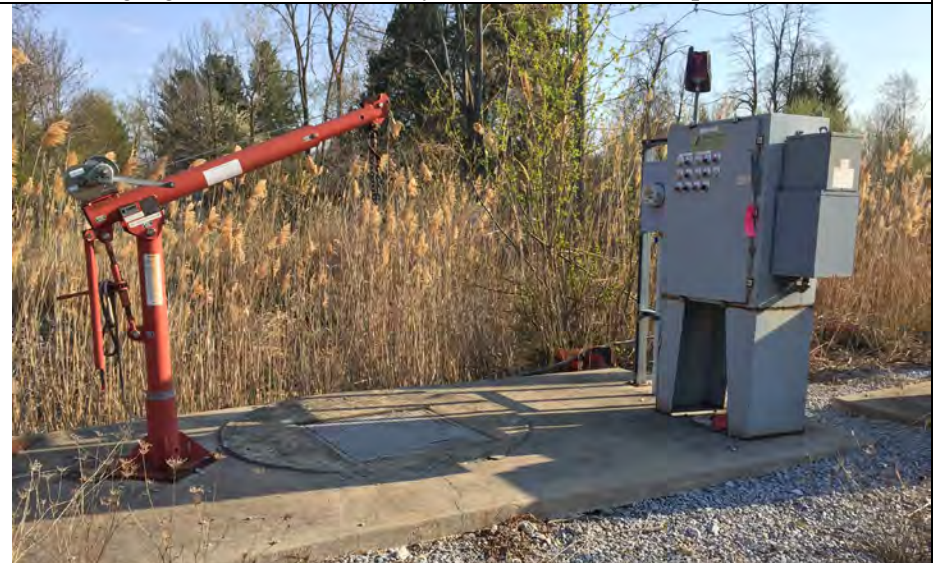
24. Sump Where 2 New Pumps Installed 2018. Pump #2 Operation Verified. Pump #1 Tripped and Scheduled for Maintenance.
