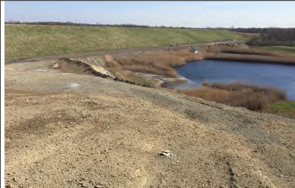
45. Runoff Collection Pond within Landfill Limits. Landfill Area Slopes Appeared Stable and Well Vegetated.
