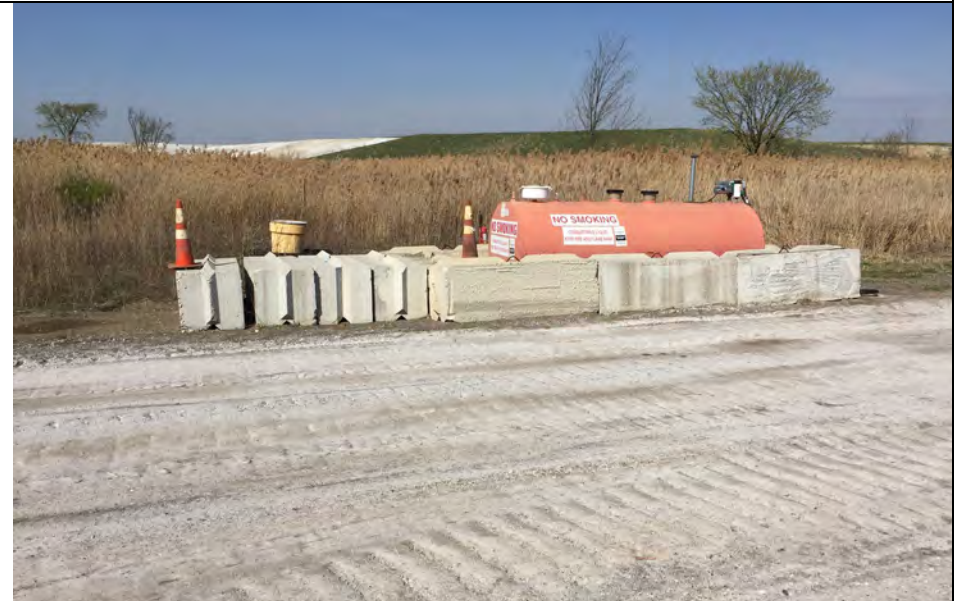
48. View of Single Fuel Tank and Enclosure Protection. Second Tank had been Removed and May No Longer be Needed.
