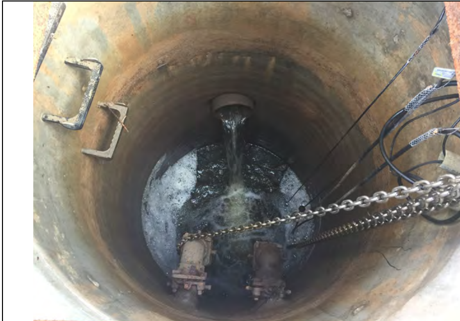
25. View Inside Pump Manhole During 2020 Inspection (No Photo for 2021; Manhole Observed. Offsite Flow into Manhole. One Running Kept up to Flow.
