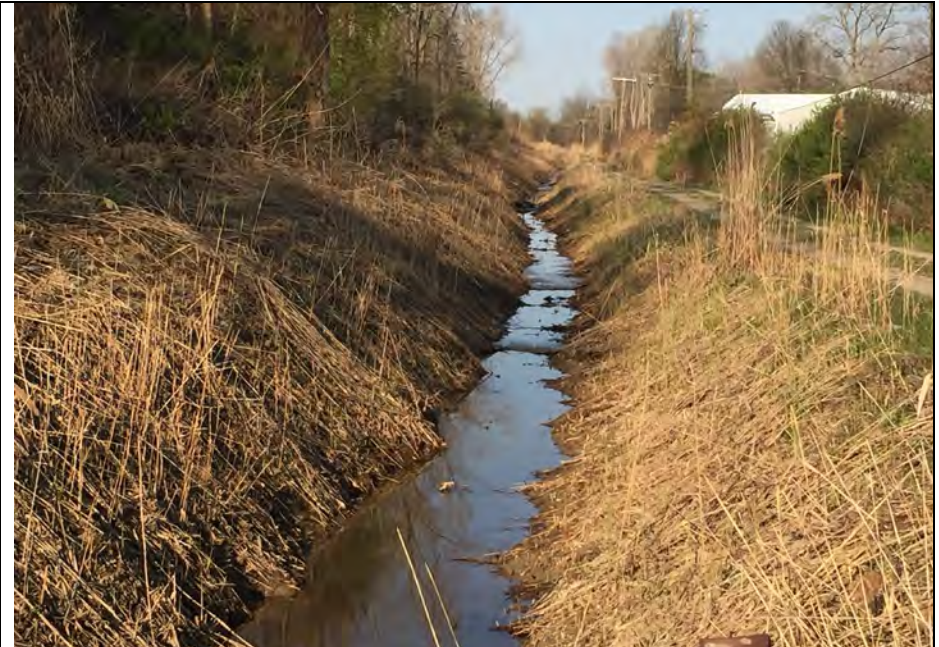
14. Looking at Ditch Alignment Approximately 200 ft Further Upstream than in Photo 13. Ditch Clear Except for Small Soil Run-in from Slope.
