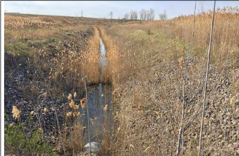
33. Older Internal Drainage Ditch within Landfill Draining to the Perimeter Collection Ditch.
