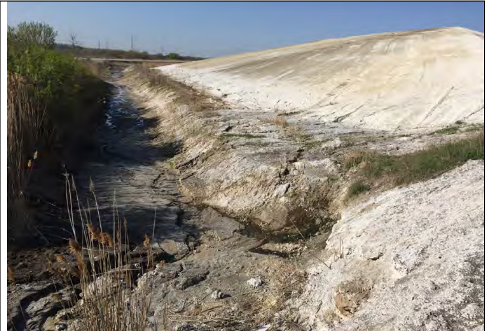
34. Temporary CCR Slope in Area G2 Along South Side. Toe Ditch Installed to Collect Directed Runoff. Slope Appears Stable and Well Graded.
