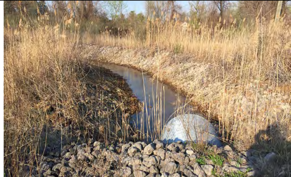
19. Another View of Portion of Perimeter Ditch Cleared of Vegetation During Routine Maintenance Activity. Culvert Open and Clear of Vegetation.
