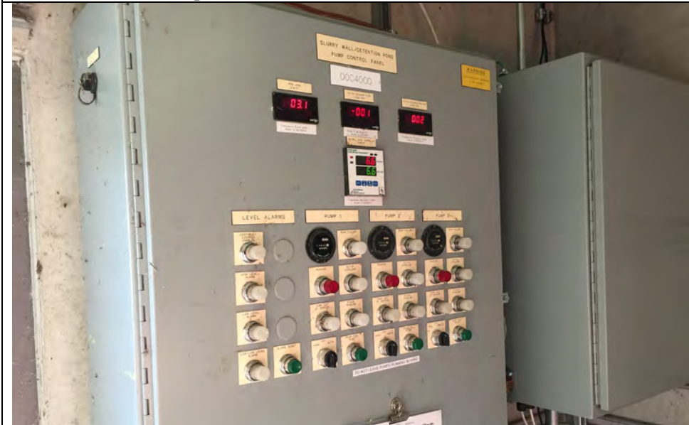
3. Pump Control Panel. All 3 Pumps were Available for Use. Wall Flow Meter (Not Shown) appeared OK. Pumps were Observed but not Pumping at the Time.
