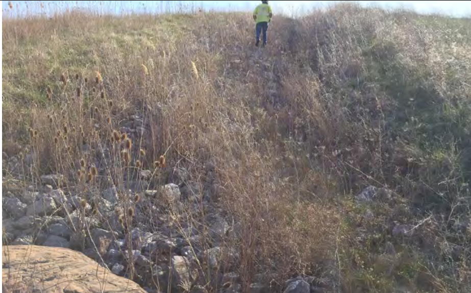
27. Inspection of Riprap Down Drain with Surface Net. Visual Voids Between and Below Riprap Suitable for Filtering in Small Size Stone, per DTE.
