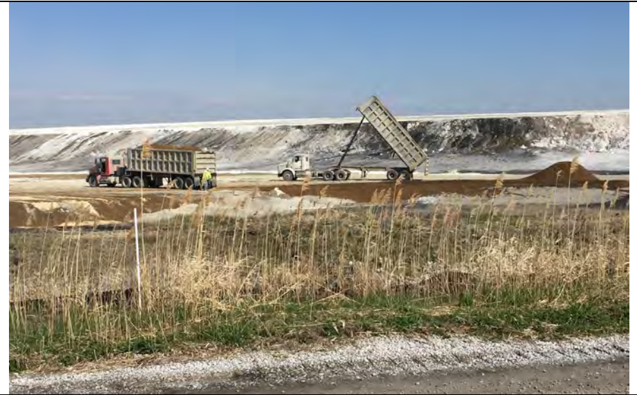
44. CCR Haul Trucks Safely Unloading What from a Distance Appears to be Bottom Ash and/or Fly Ash.
