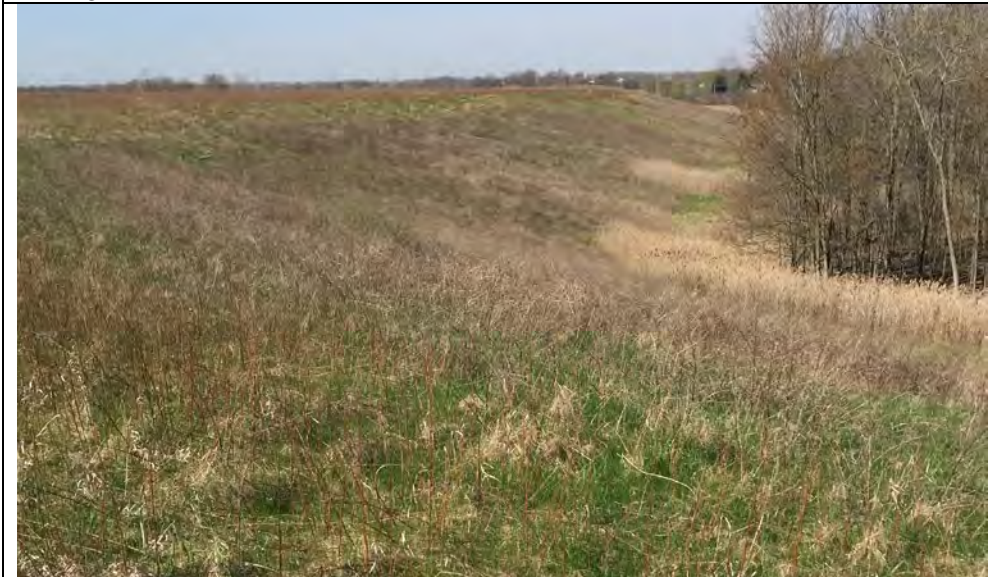
51. Outside Perimeter Slope Along Closed Area F1. Slope Appeared Stable and Well Vegetated.
