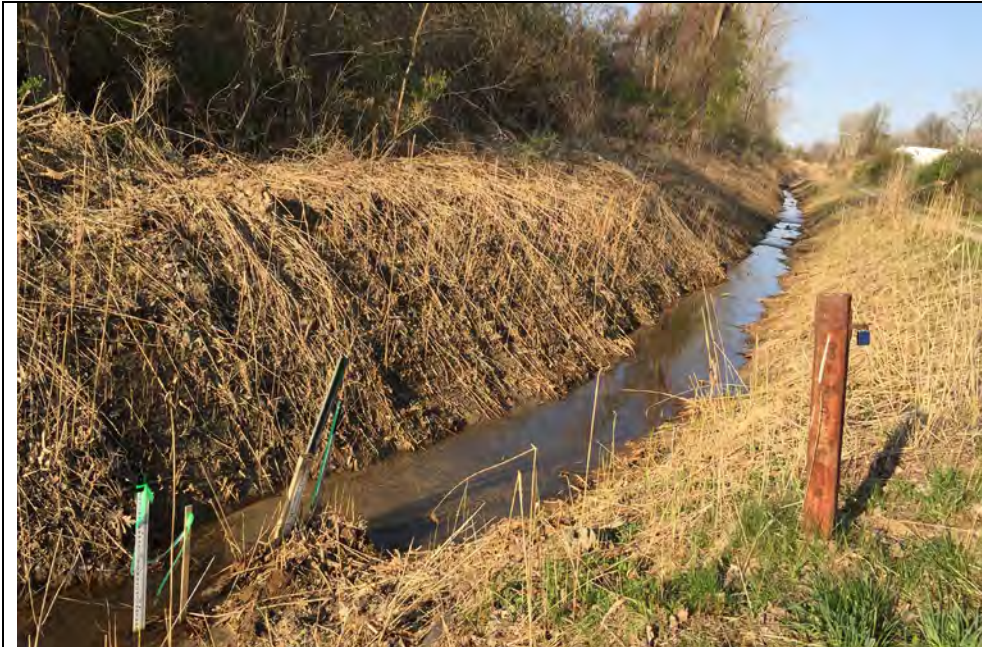
13. Looking at Location of Staff Gauge SG-02. Water Present. No Visible Flow Noted.
