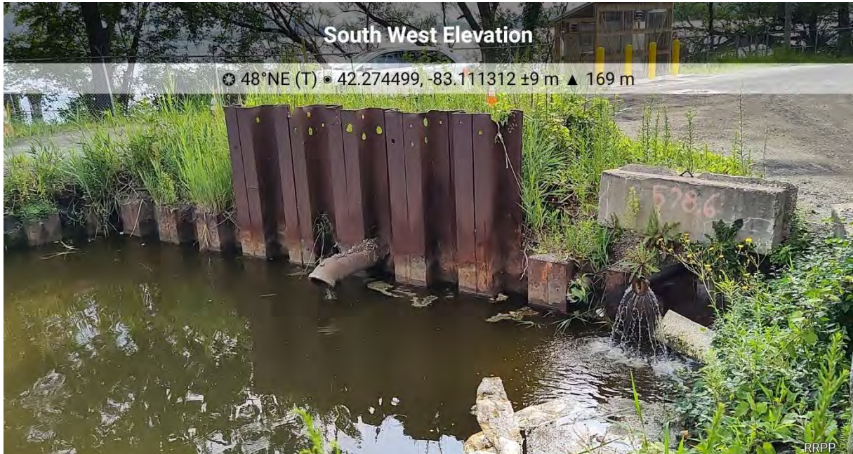
Photograph 1: Inlet Pipes at East End of Basin from Southeast Corner of Basin Looking Northeast
