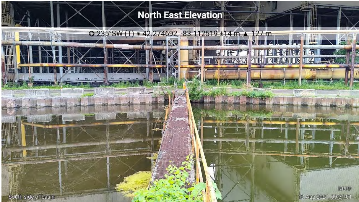
Photograph 5: Underflow Weir and BFG Condensate Drain from North Side of Basin Looking South
