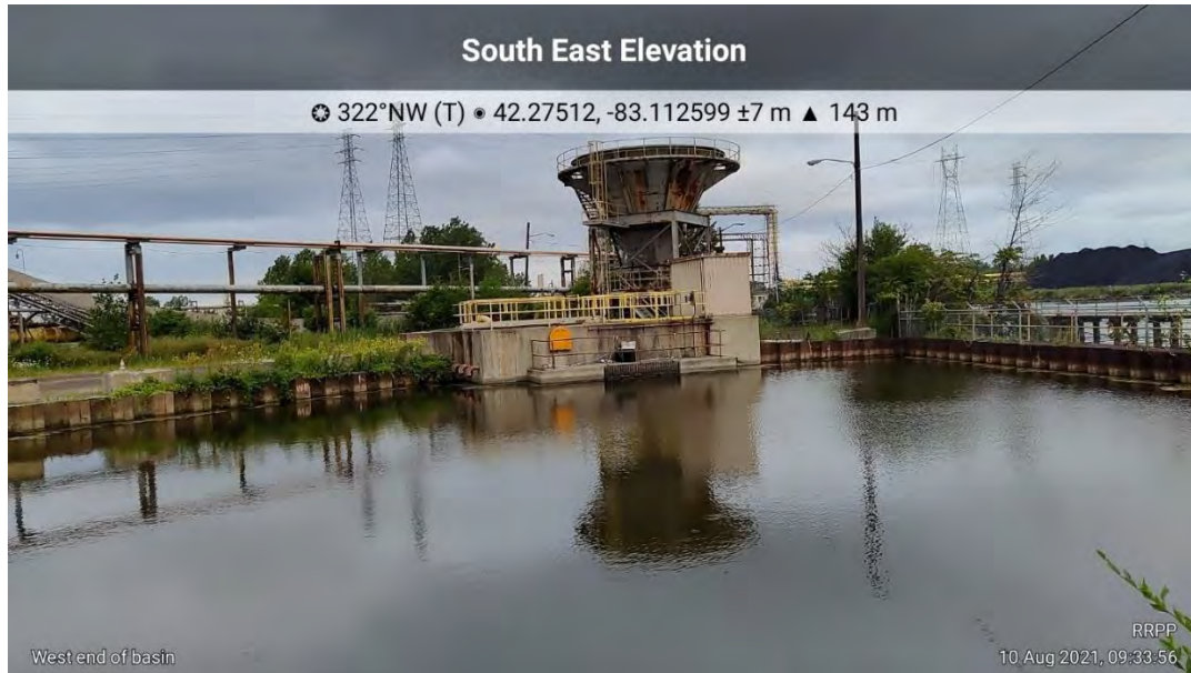
Photograph 7: Pump House and Overflow Weir Looking West from North Side of Basin
