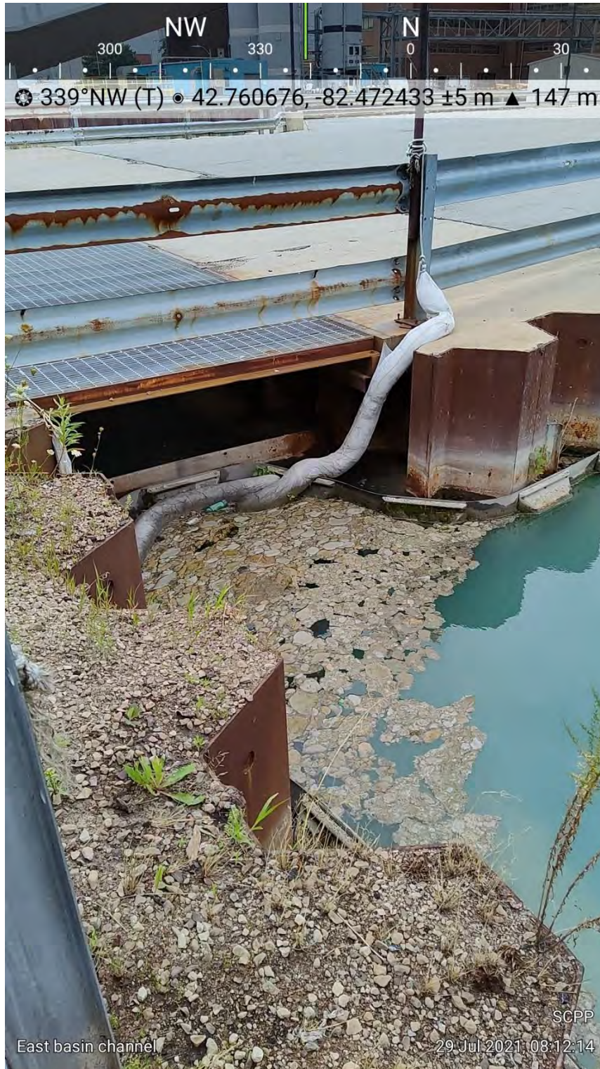
Photograph 4: East Basin Box Culvert Opening from Southwest Corner of East Basin Looking Northwest
