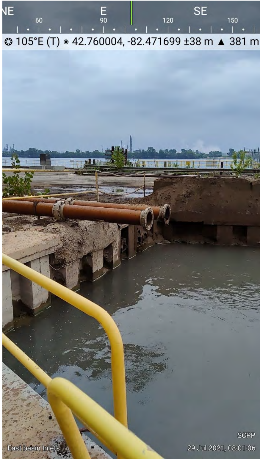
Photograph 1: East Basin Inlet Pipes from Northwest Corner of East Basin Looking East
