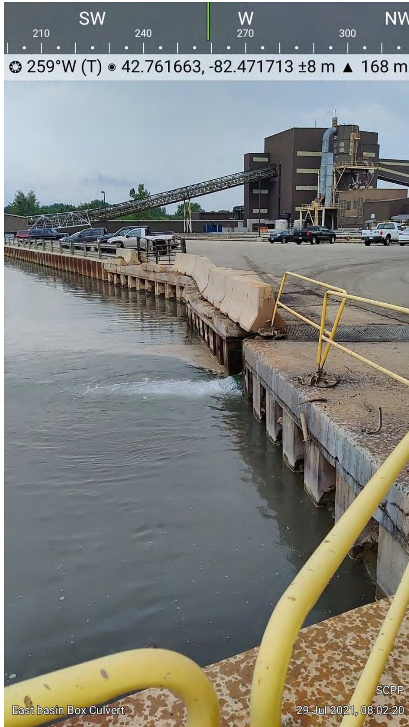
Photograph 2: East Basin Box Culvert Inlet from North End of Basin Looking Southwest
