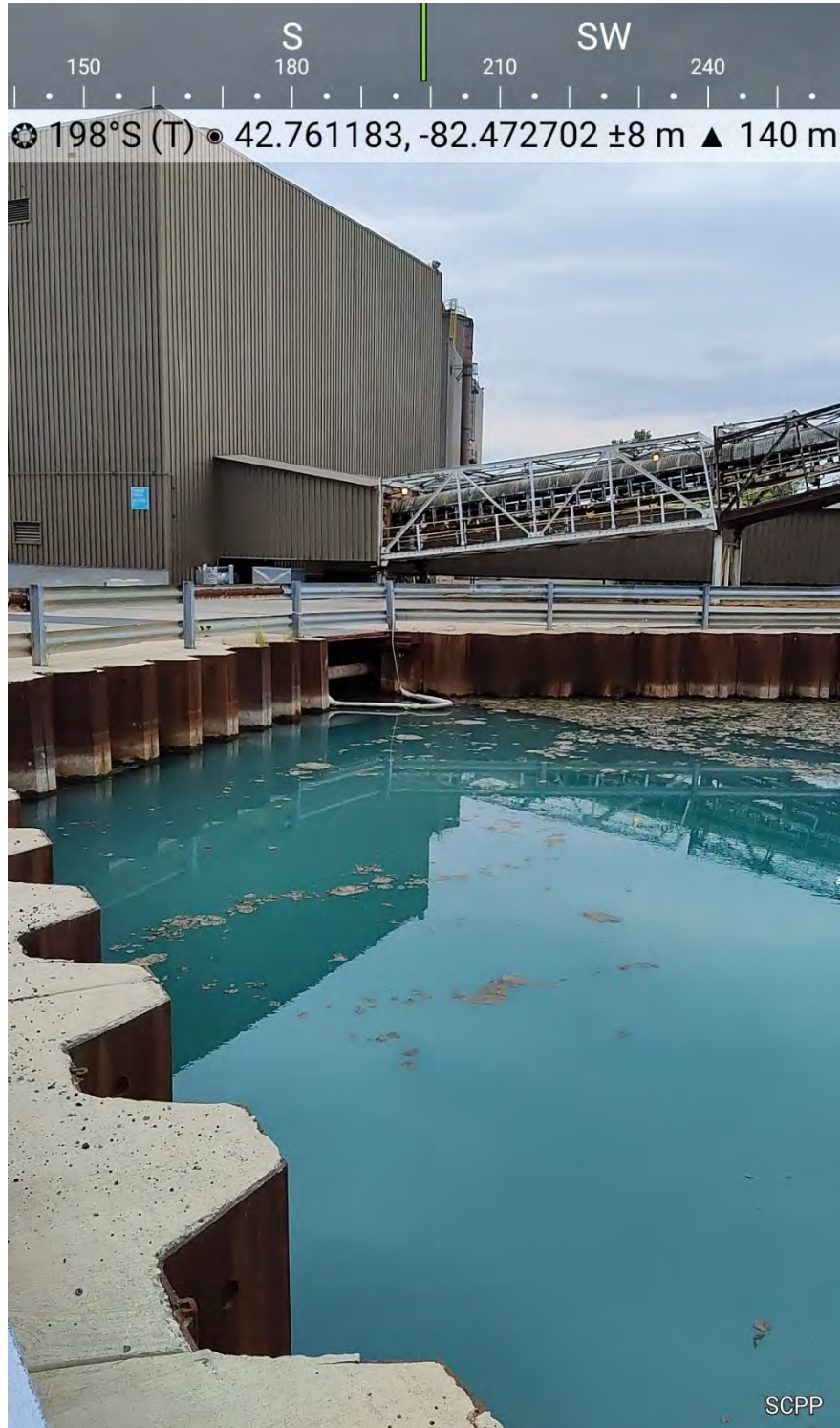
Photograph 5: West Basin Box Culvert Opening from East Side of West Basin Looking South
